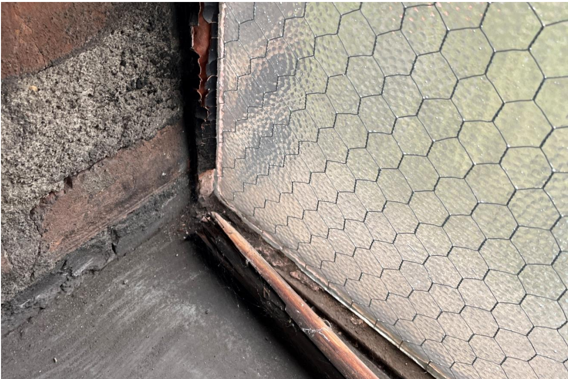
Window 11. 3 rd Floor, rear (north) elevation. Hot rolled steel unit. 12/11/2024.
