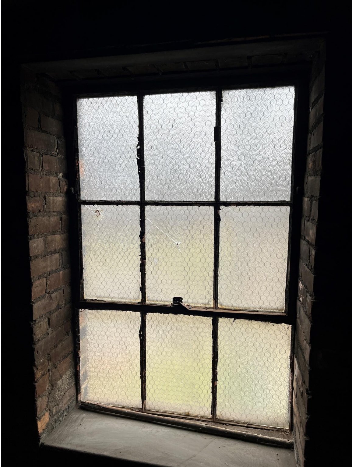
Window 11. 3 rd Floor, rear (north) elevation. Hot rolled steel unit. 12/11/2024.
