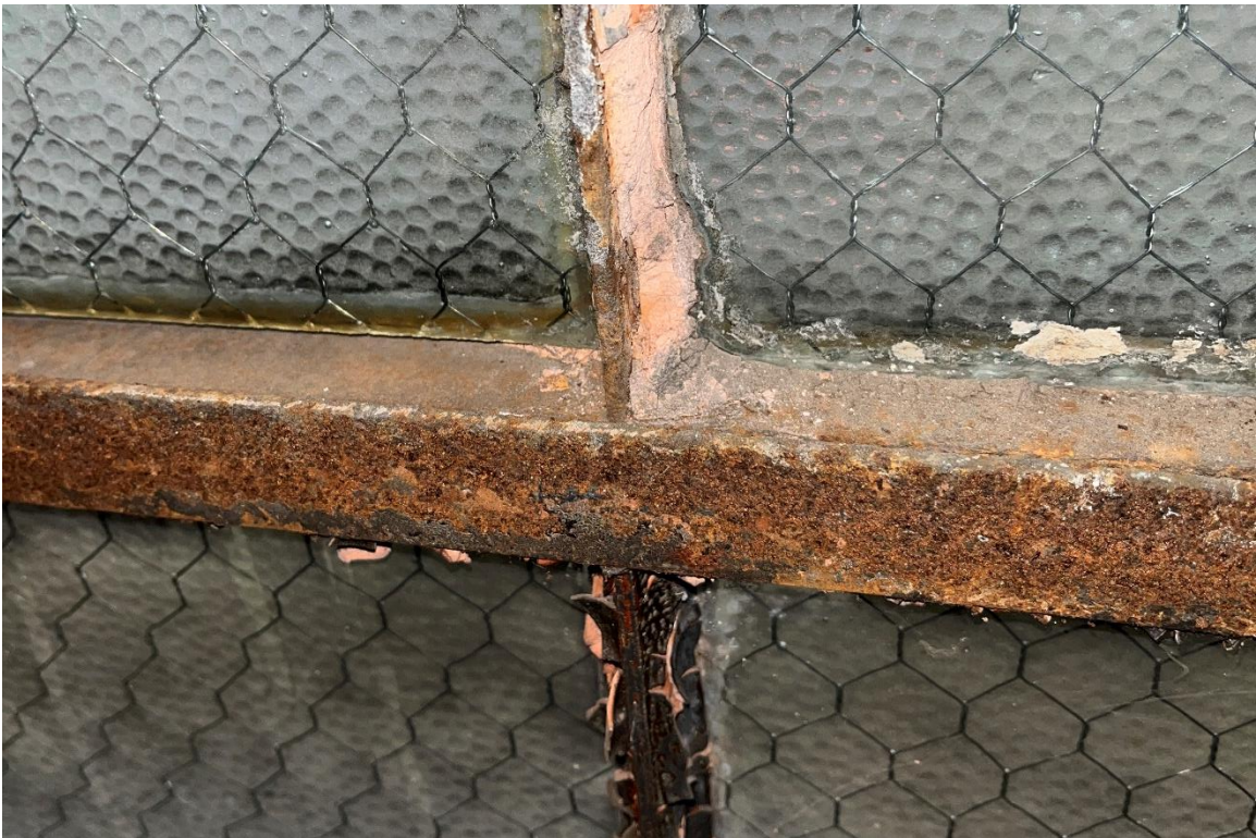
Window 12. 2 nd Floor, rear (north) elevation. Hot rolled steel unit. 12/11/2024.
