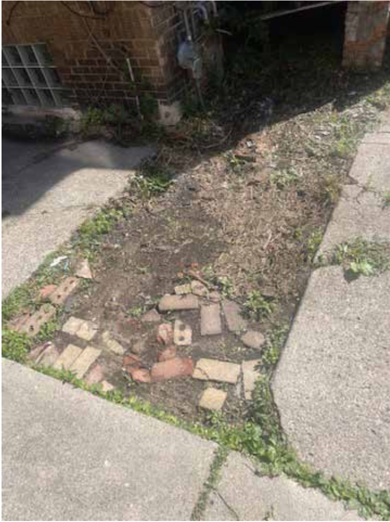
Missing concrete in driveway leading into the backyard.
