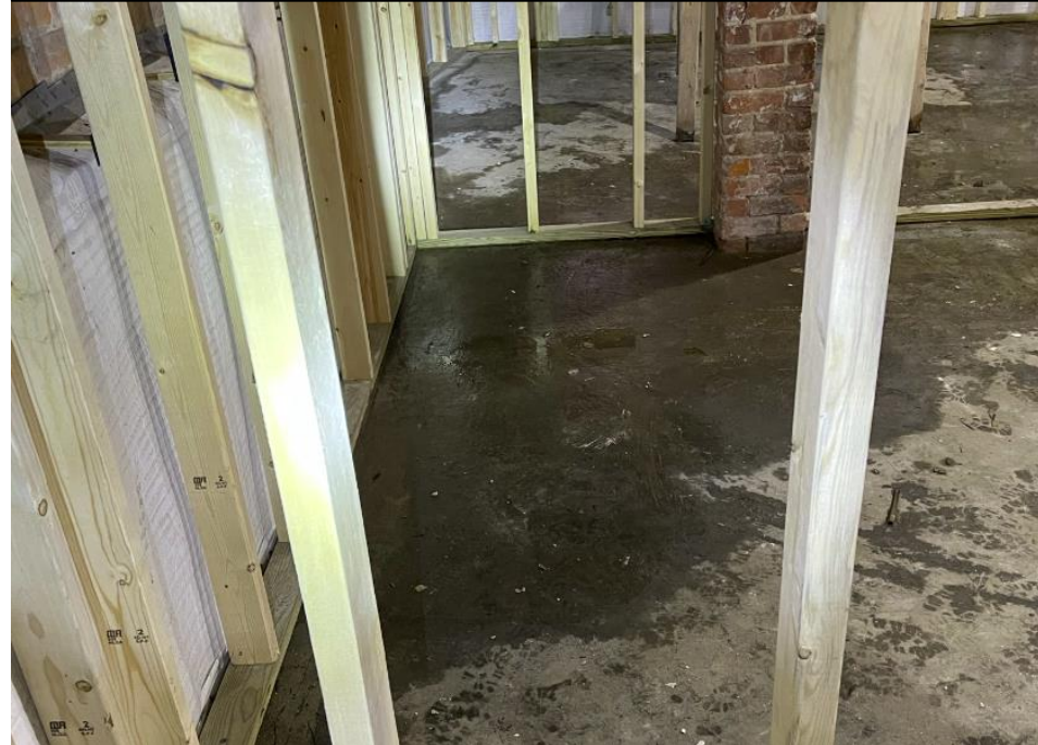
Basement living area water intrusion
