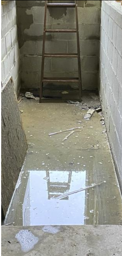
Stairwell water intrusion
