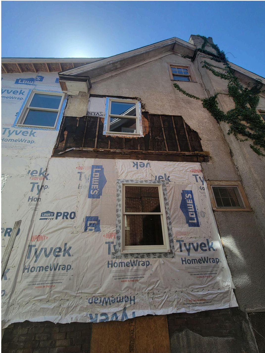
Typical Stucco Damage
