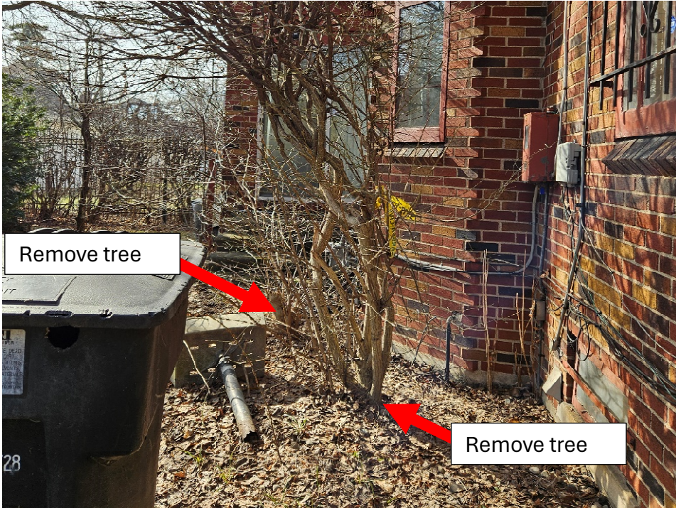
House South Elevation - Remove two small trees near foundation wall
