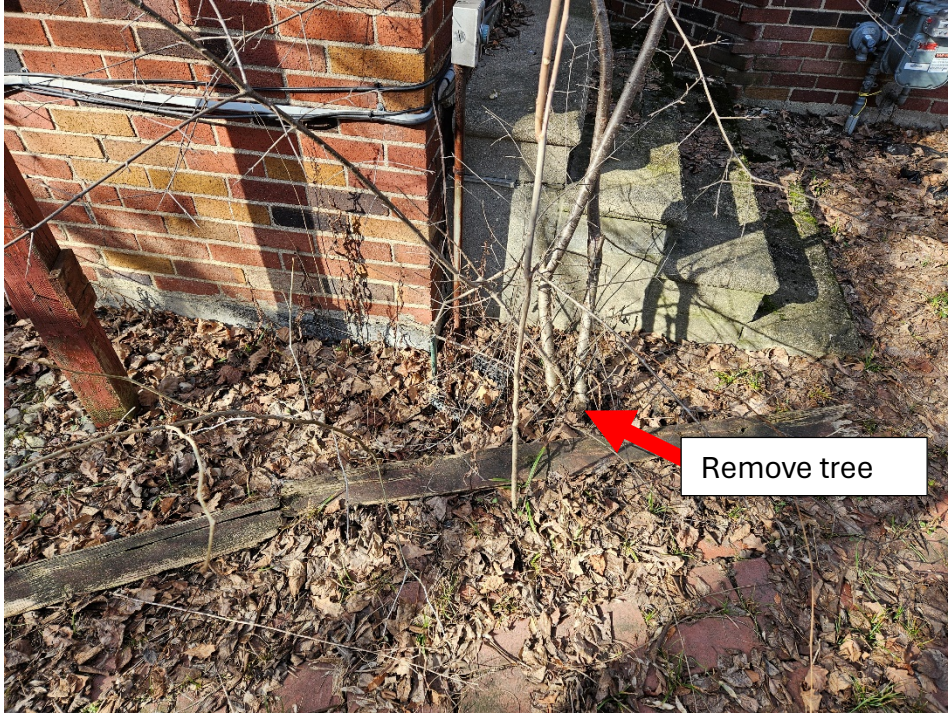
House South Elevation - Remove small tree near foundation wall
