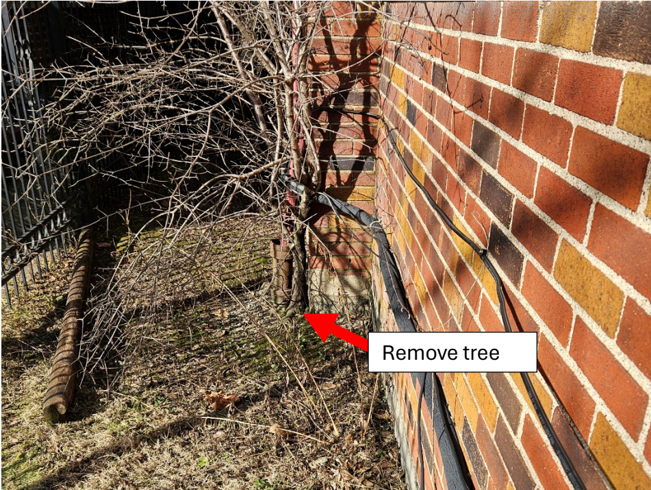
House West Elevation - Remove small tree near foundation wall
