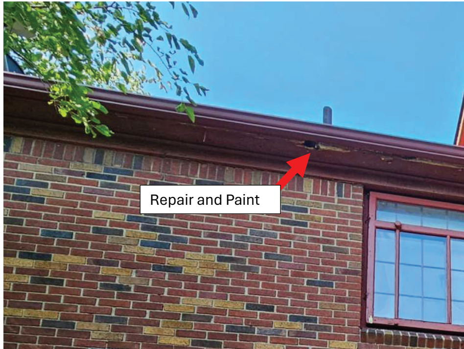
House East Elevation – Damaged wood soffit
