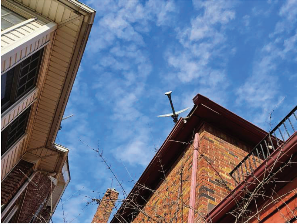
House West Elevation – Damaged gutter overview
