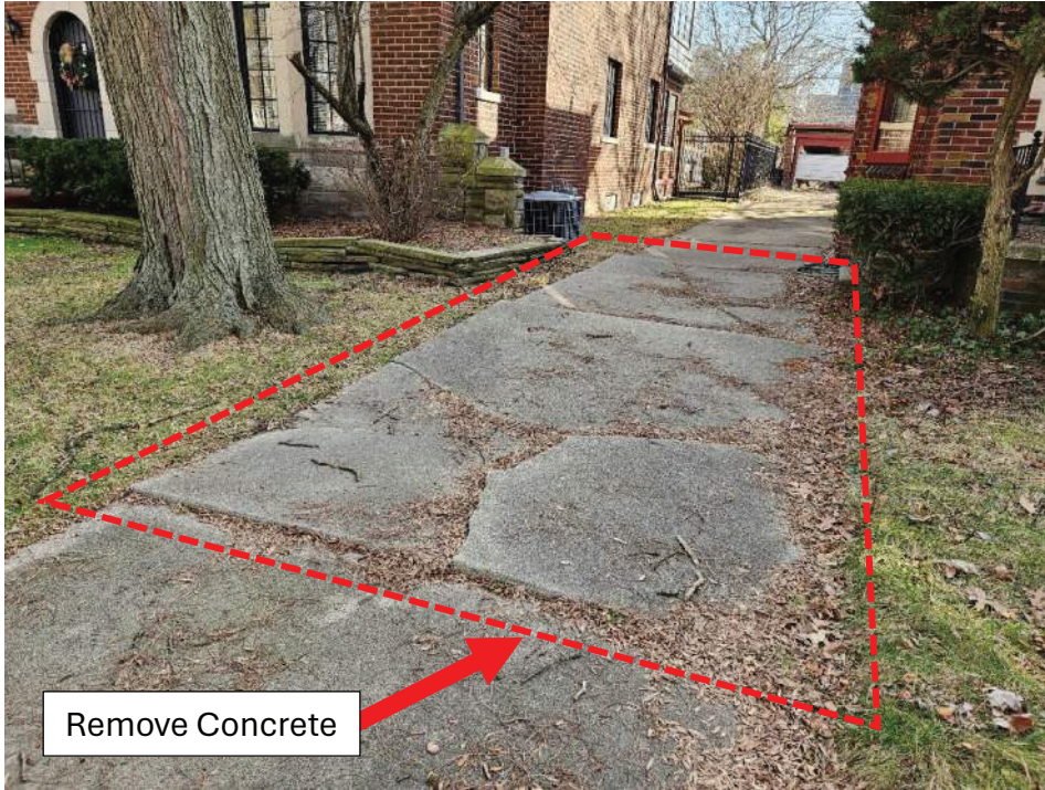
Driveway Looking South – Two damaged concrete pads
