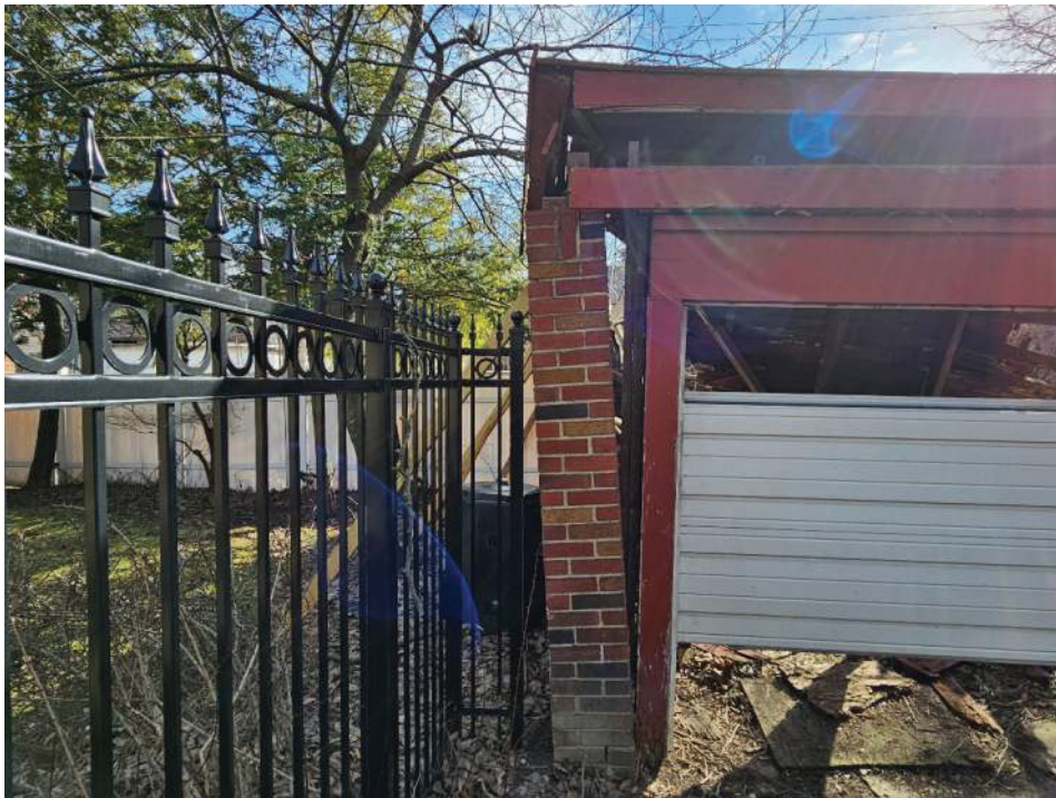
Garage North Elevation – Displaced wall
