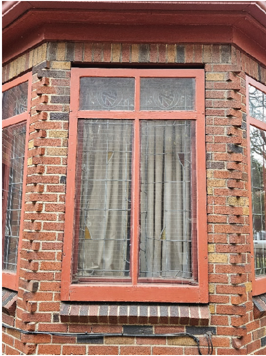
House East Elevation – Exterior view of damaged window
