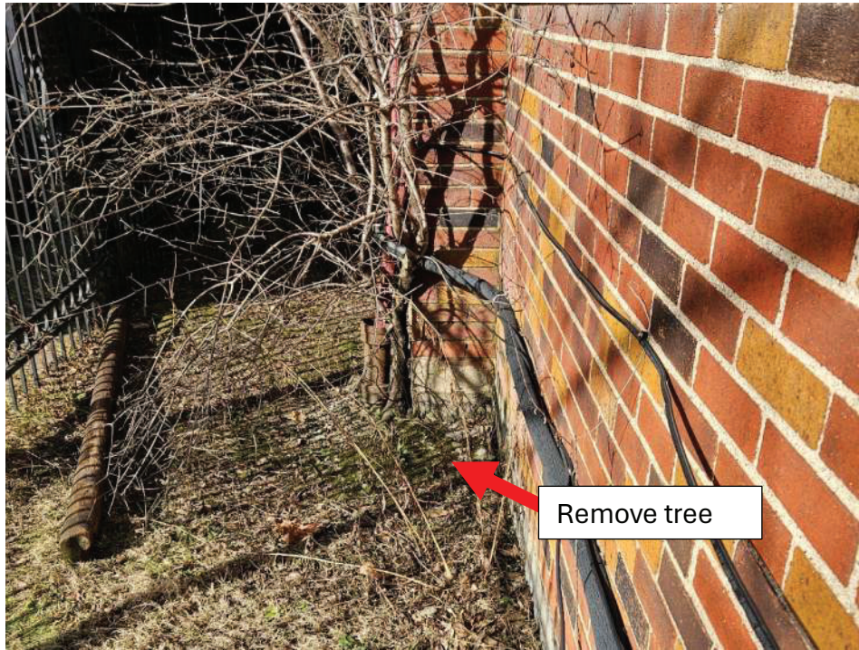
House West Elevation - Example of small tree near foundation wall
