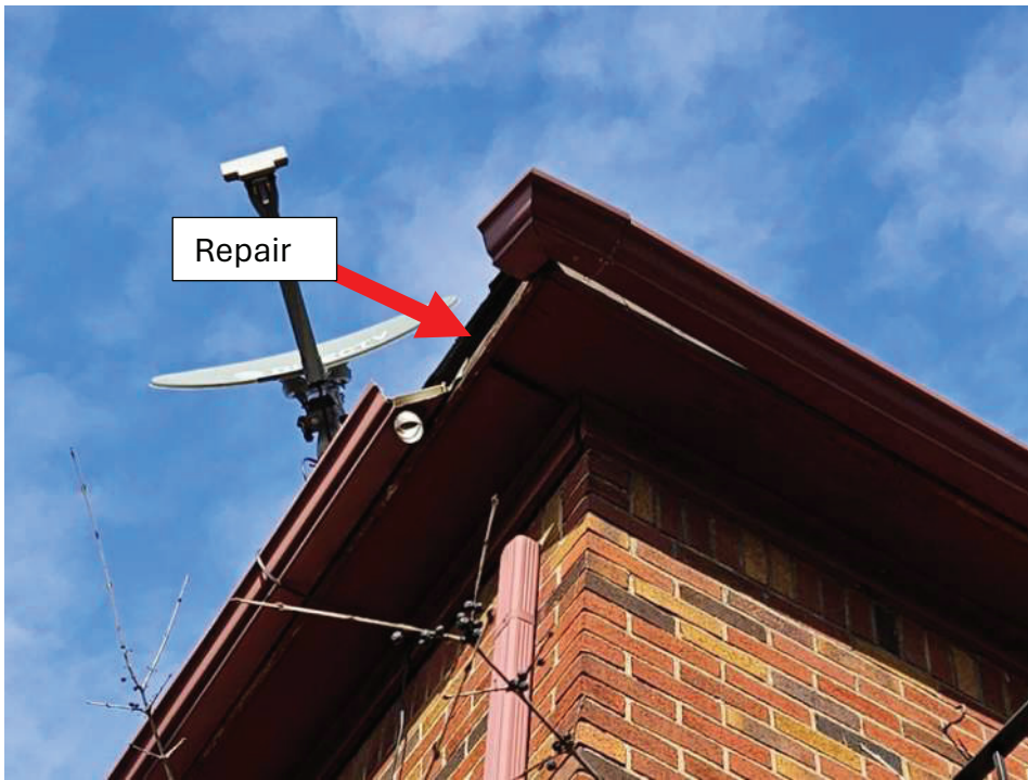
House West Elevation – Damaged gutter enlarged view
