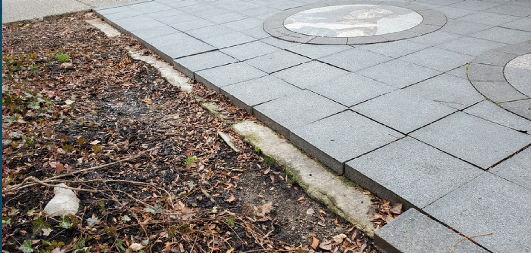
F. Interior Park Pavers: Where cracked, will be replaced and repaired, power-washed to refresh
