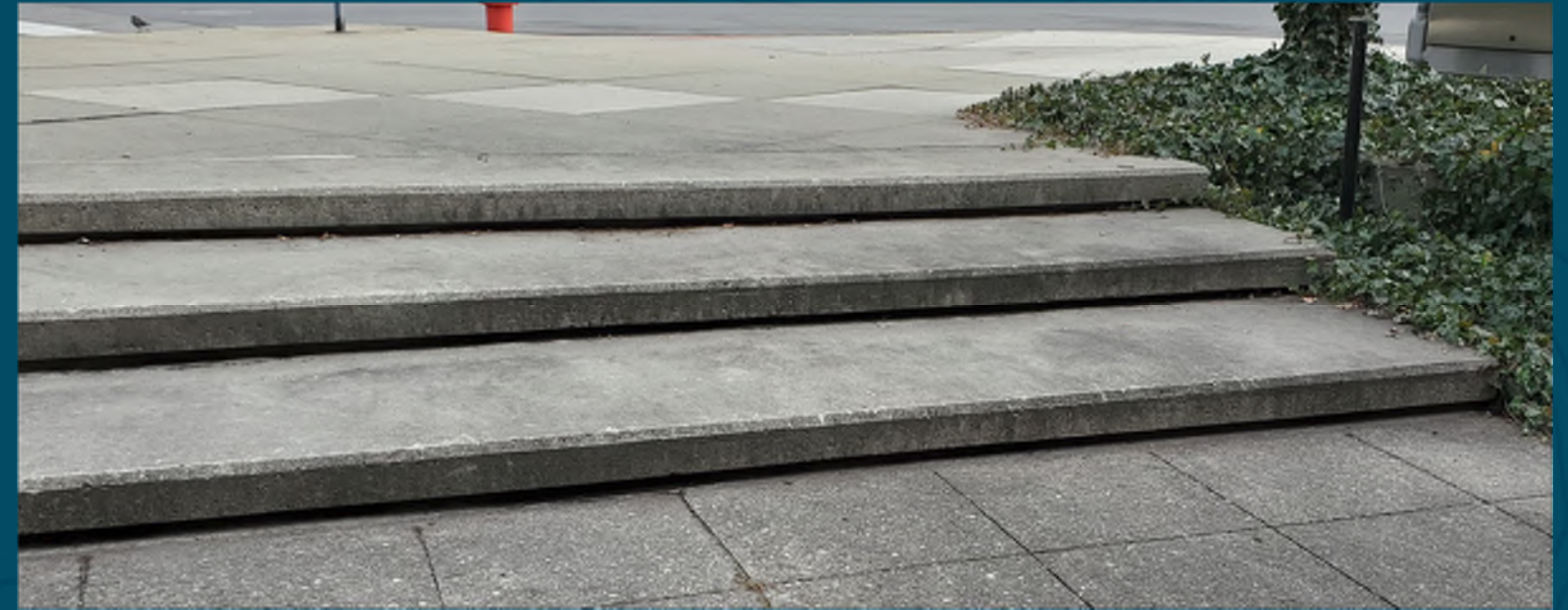
Z. Concrete Stairs to be removed, increase paver area & connect concrete retaining wall
