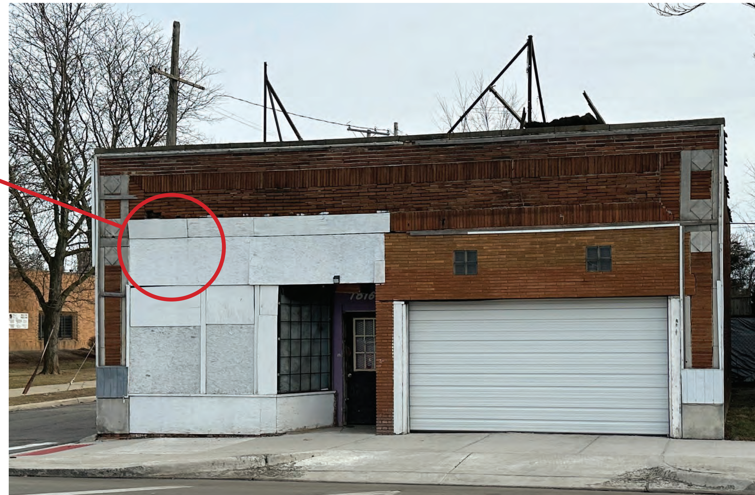
EXISTING BOARDED UP STORE FRONT
