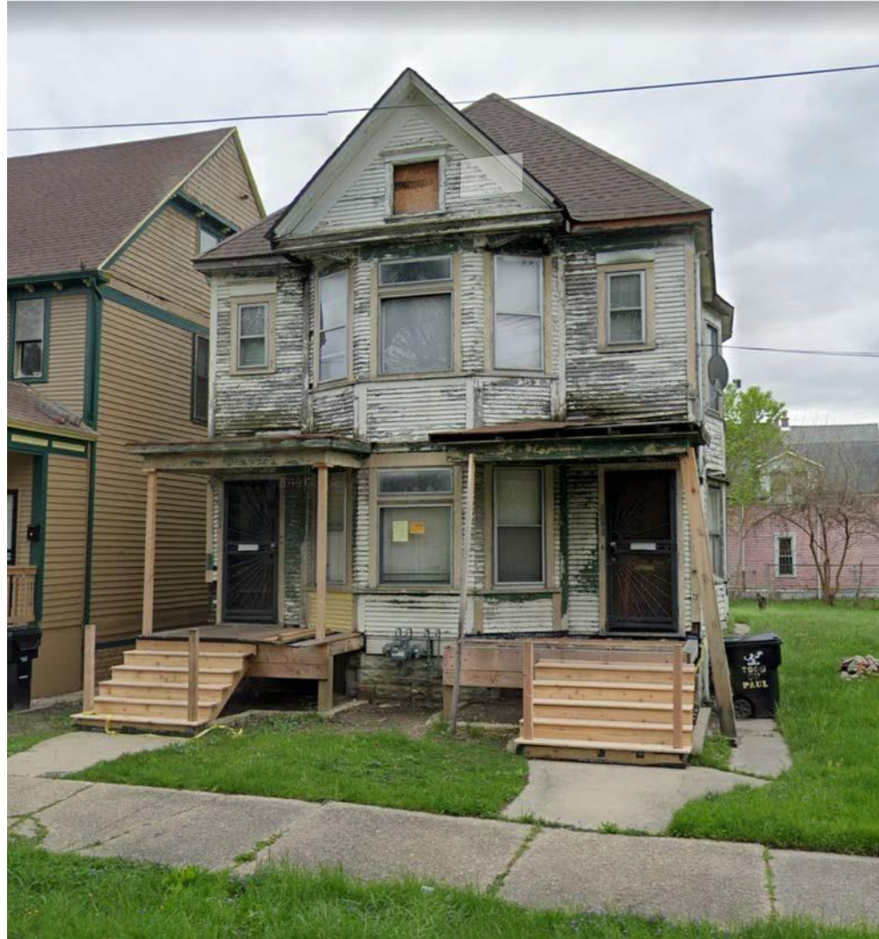
PREVIOUS CONDITION OF 7908 SAINT PAUL BEFORE SIDING AND WINDOWS WERE REMOVED; IMAGE FROM 2019 - FRONT ELEVATION
