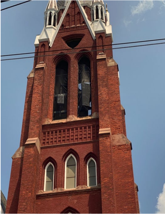
Zoom View of Antennas with new placement
