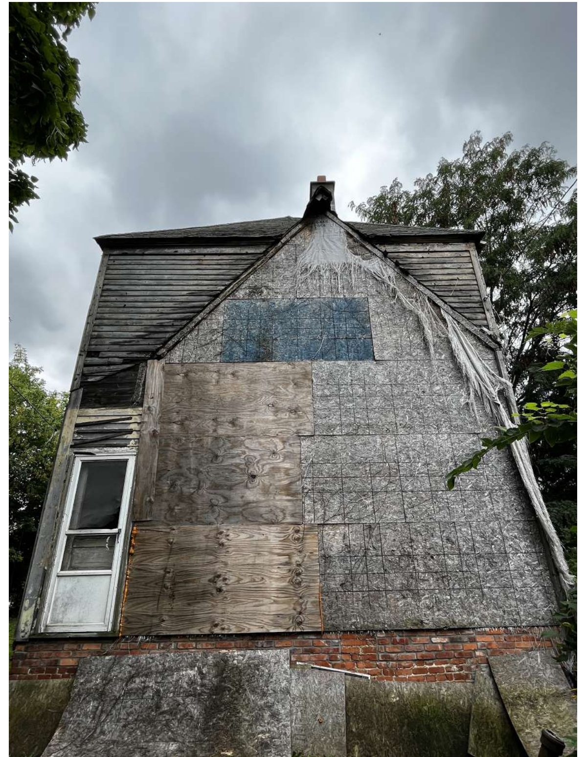
ALL EXISTING SIDING AND TEMPORARY SHEATHING AT REAR IS TO BE REMOVED AND REPLACED WITH NEW LAP-SIDING MATCHING EXISTING IN TYPE, PROFILE, AND EXPOSURE
