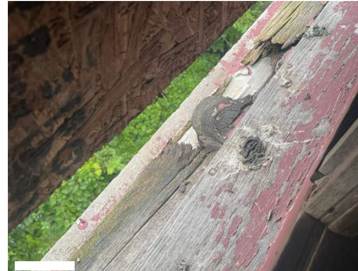
TYPICAL EXAMPLE OF FAILURE OF FINGER JOINT CONNECTION AT LOWER RAIL OF TOP SASH.
