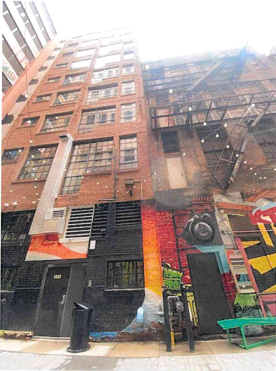
Photo 6. New aluminum replica windows on same elevation as windows in question for 1315 Broadway
