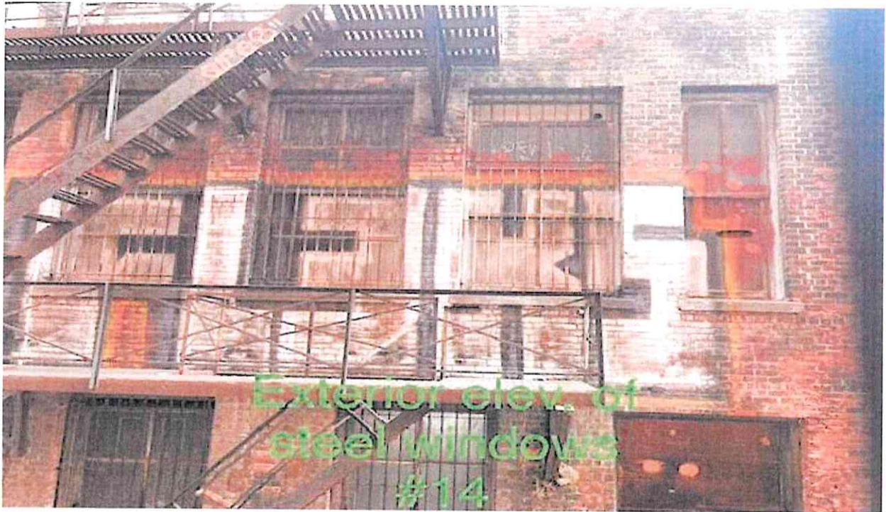
Photo 3. Typical vandalism and exterior conditions of windows
