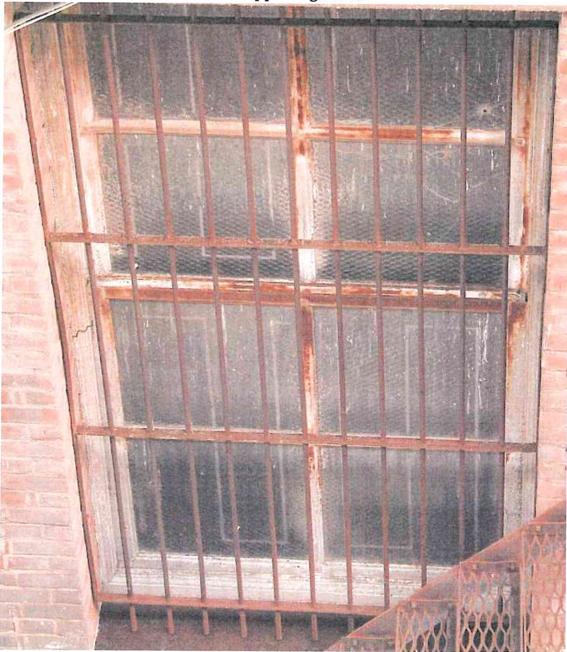
Picture 1. Exterior view of typical steel window with rust/corrosion
