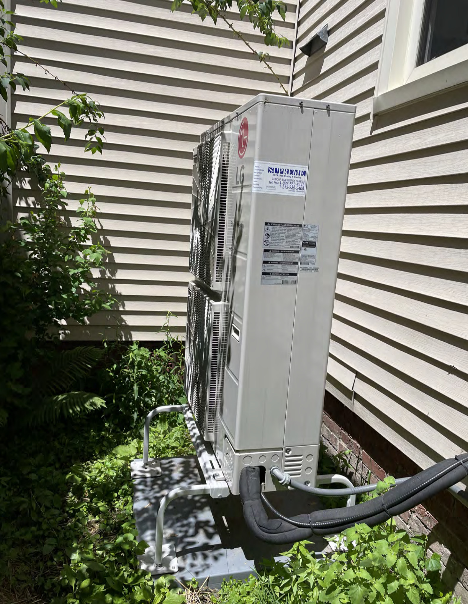
HEAT PUMP COMPRESSOR AT SOUTH END OF WEST FACADE
