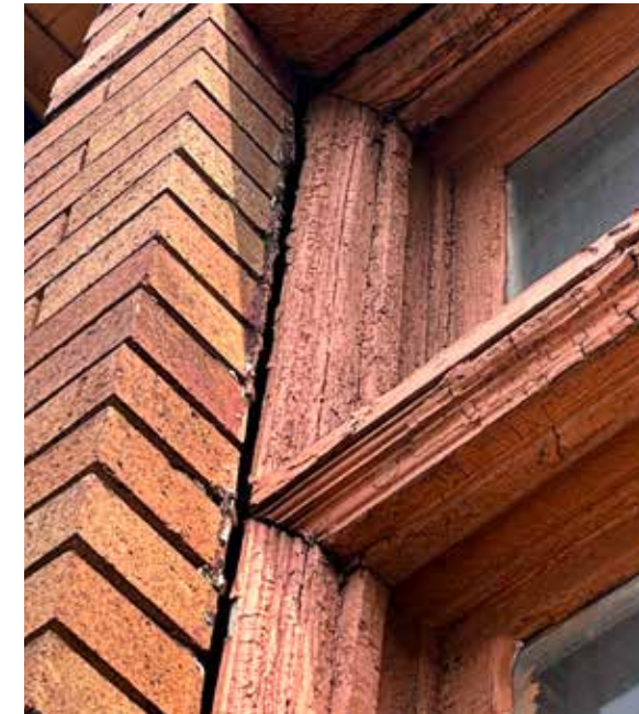
DETAIL OF DETACHED BRICK AT SECOND LEVEL EAST SIDE OF FRONT BAY
