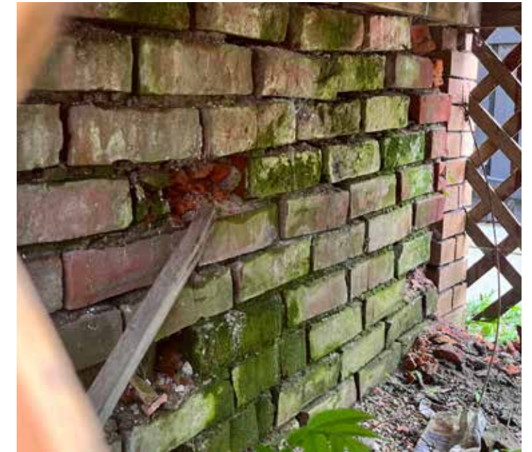
BRICK CONDITION UNDER WEST FRONT PORCH
