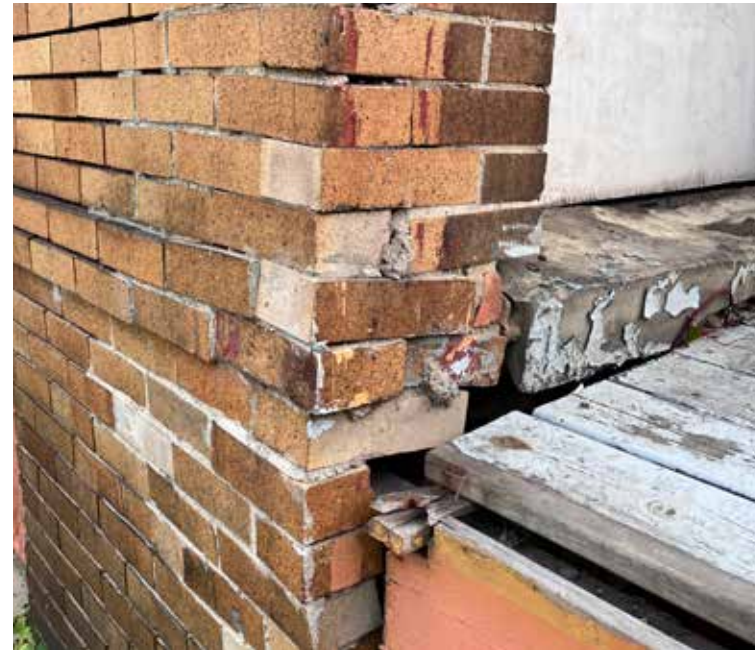
CONDITION AT LOWER PORTION OF WEST FRONT PORCH ENTRY - POOR REPAIR AND BULGING
