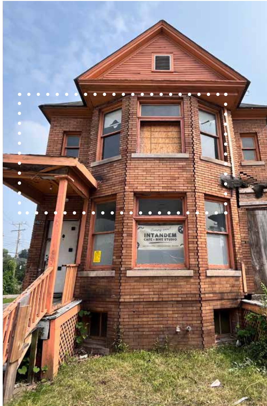
PHOTOS TO THE RIGHT DETAIL THE SECOND LEVEL AND UPPER PORTION OF THE FIRST LEVEL OF THE EAST AND MIDDLE PORTIONS OF THE FRONT FACADE
