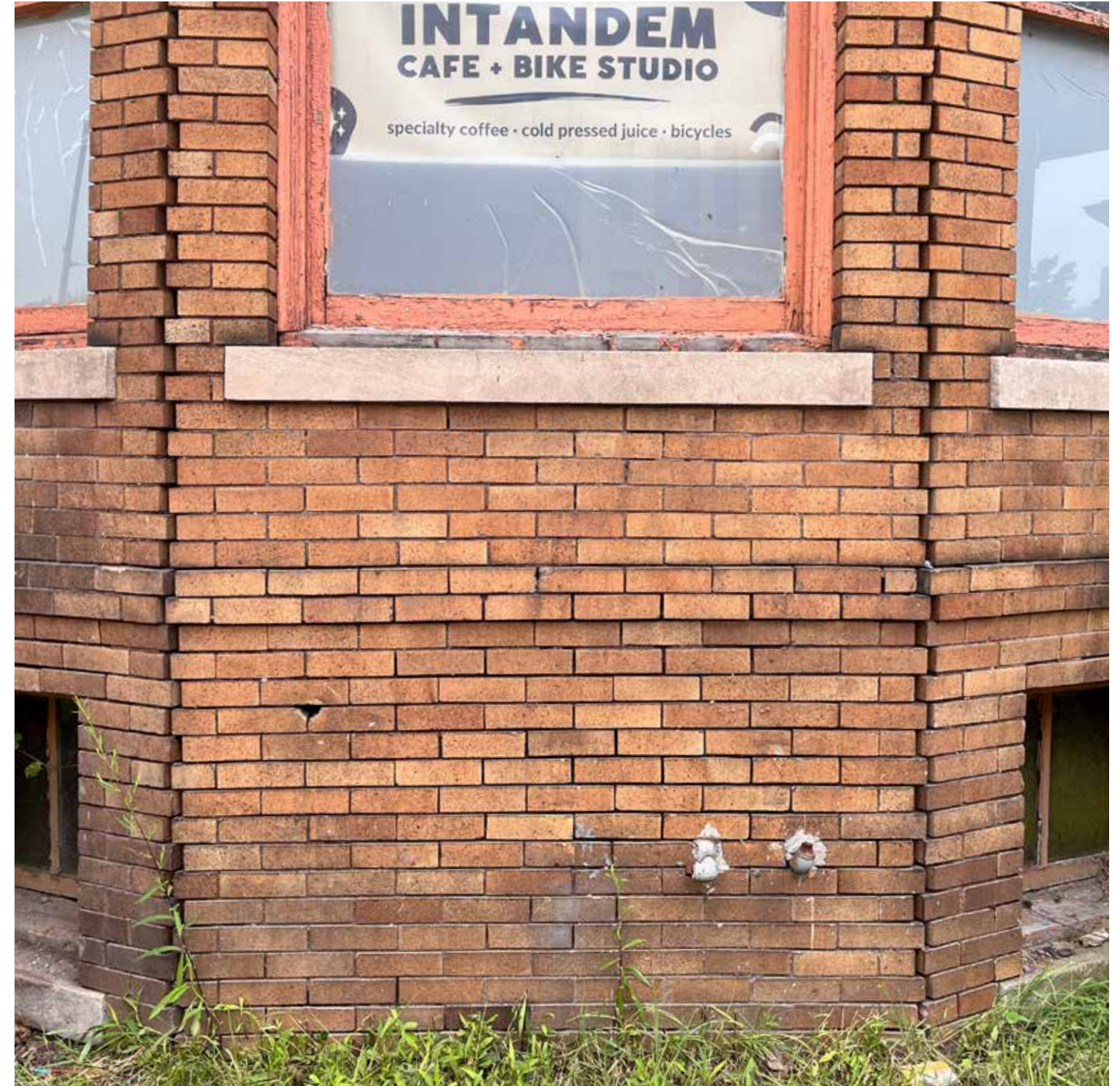
Area below large center bay window cleaned per HDC request. The left half of that brick was done twice with a non-ionic detergent and low-mid pressure washing. The right half of that brick was water blasted alone. Cleaning via these techniques made very little difference in the appearance of the brick.
