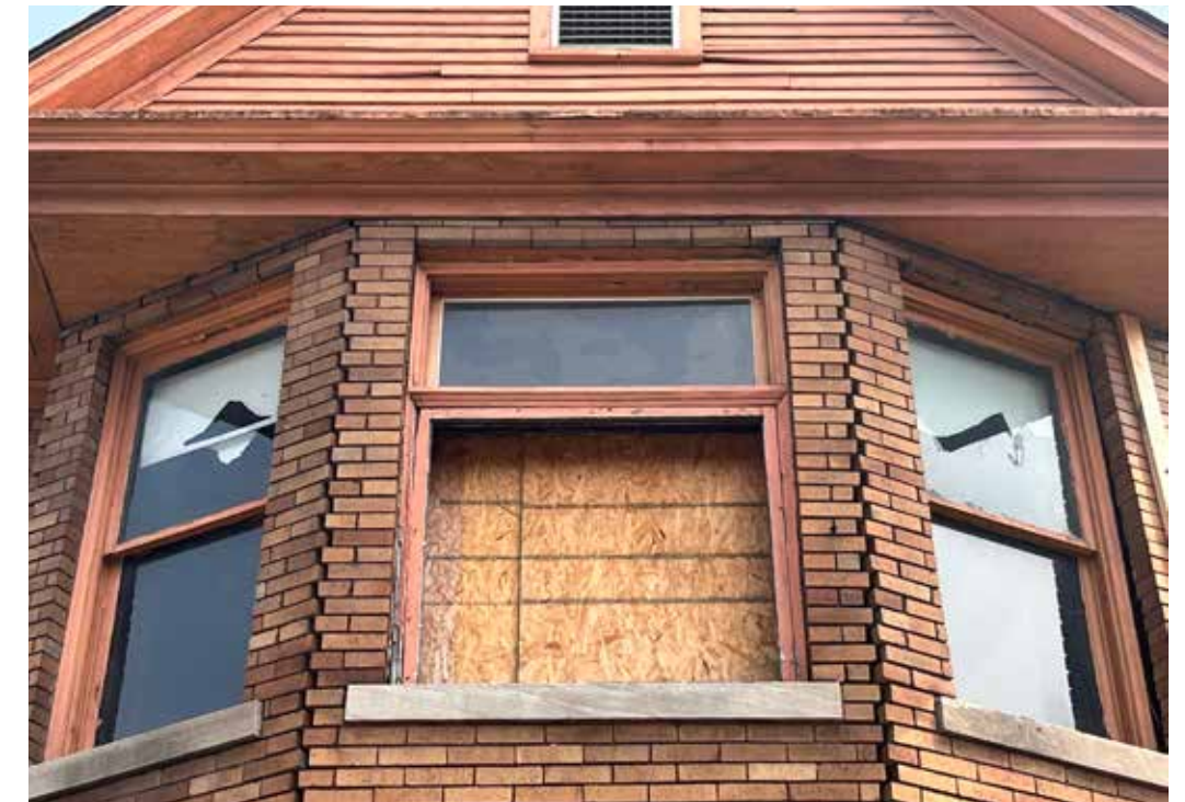
GENERAL CONNDTION AT SECOND LEVEL OF FRONT BAY
