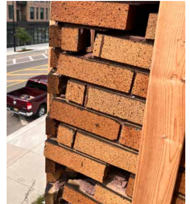
COMPLETE VENEER FAILURE
