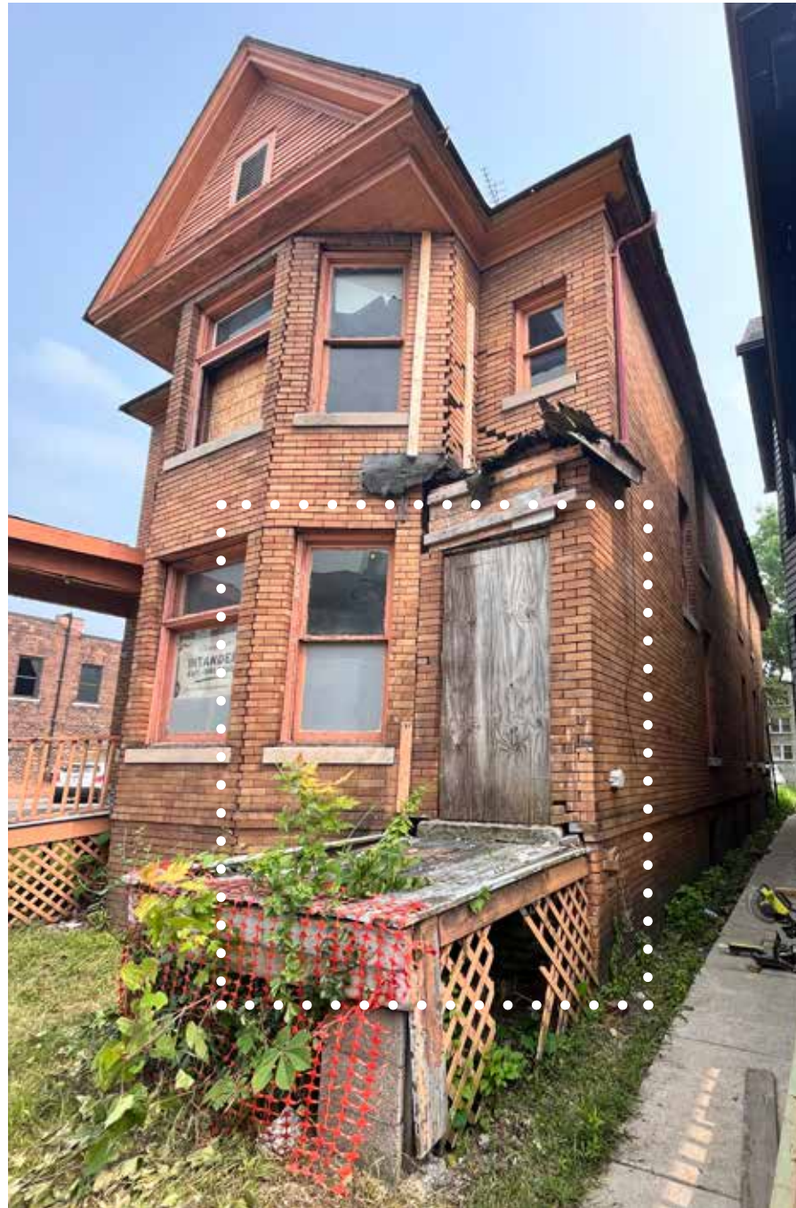
PHOTOS TO THE RIGHT DETAIL THE FIRST LEVEL BRICK CONDITION AT THE WEST SIDE OF THE FRONT FACADE.
