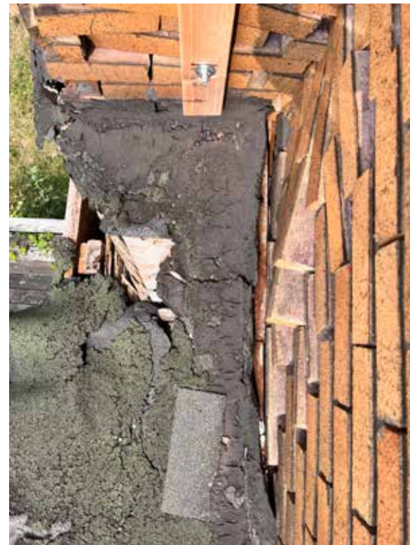
REMAINS OF WEST FRONT PORCH ROOF OPEN TO ELEMENTS
