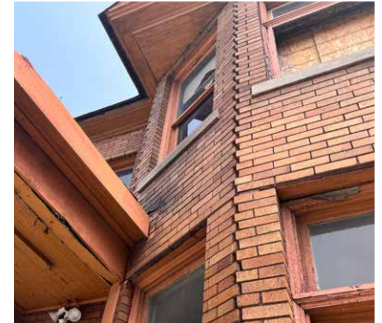
BRICK CONDITION AT UPPER LEFT BAY
