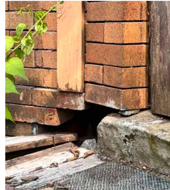
MISSING BRICKS TO LEFT OF WEST ENTRY DOOR
