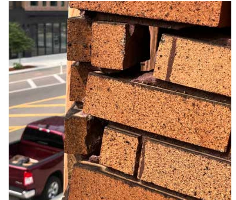
DETACHED BRICK AT SECOND LEVEL OF WEST SIDE OF MIDDLE BAY
