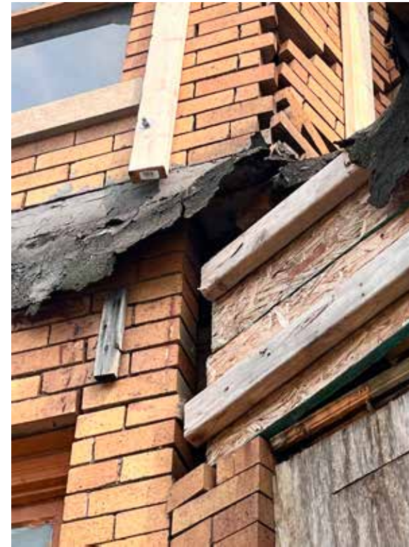
CONDITION ABOVE WEST FRONT PORCH ENTRY
