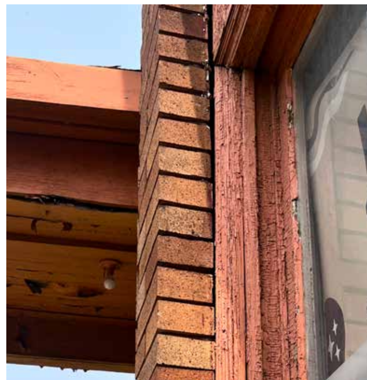
DETACHED VENEER AT EAST SIDE OF FRONT BAY AT FIRST LEVEL
