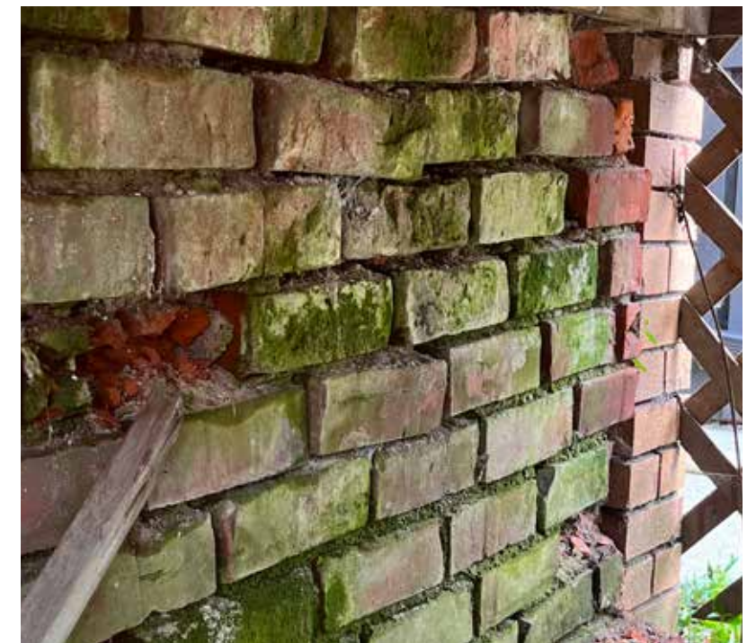
D. Common brick below West front entry porch is bowed with loose bricks and failing mortar
