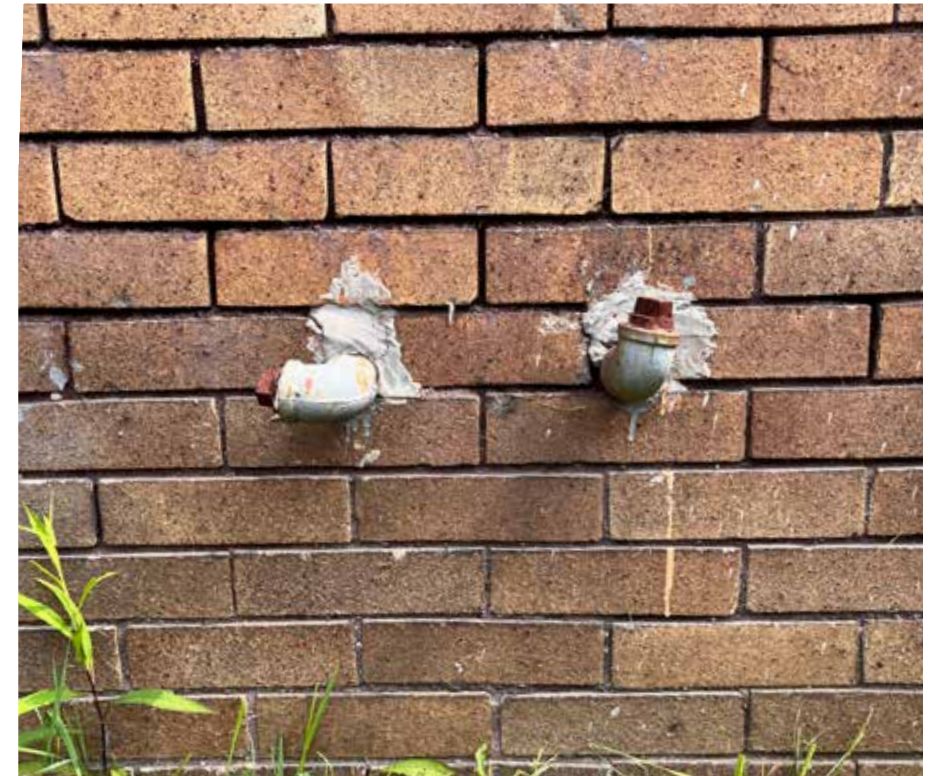
BRICK CONDITION AT MIDDLE FRONT BAY AT OLD GAS CONNECTION POINTS
