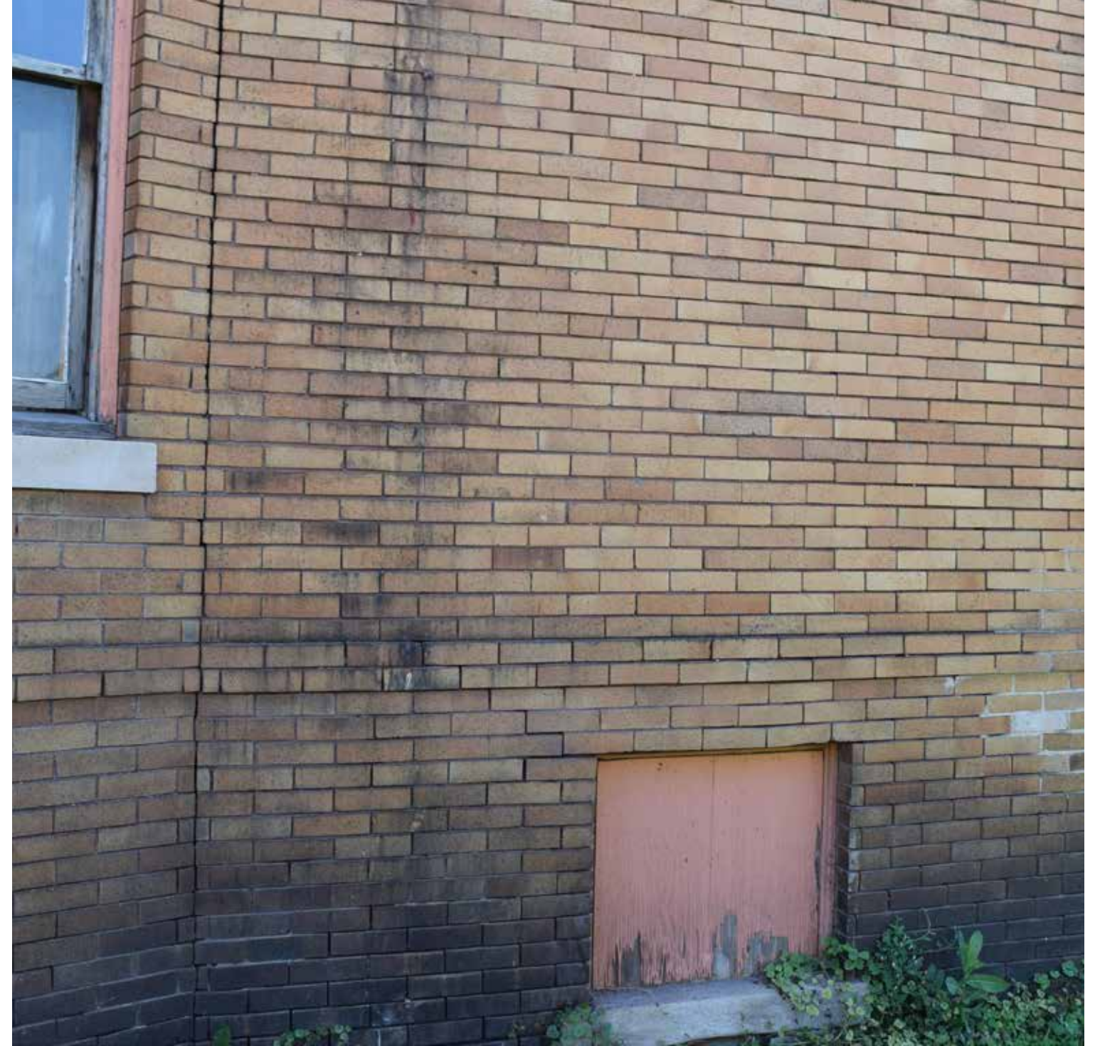
Area to the left of the basement window was cleaned via HDC request with a non-ionic detergent and low-mid pressure washing. Cleaning via these techniques made very little difference in the appearance of the brick.
