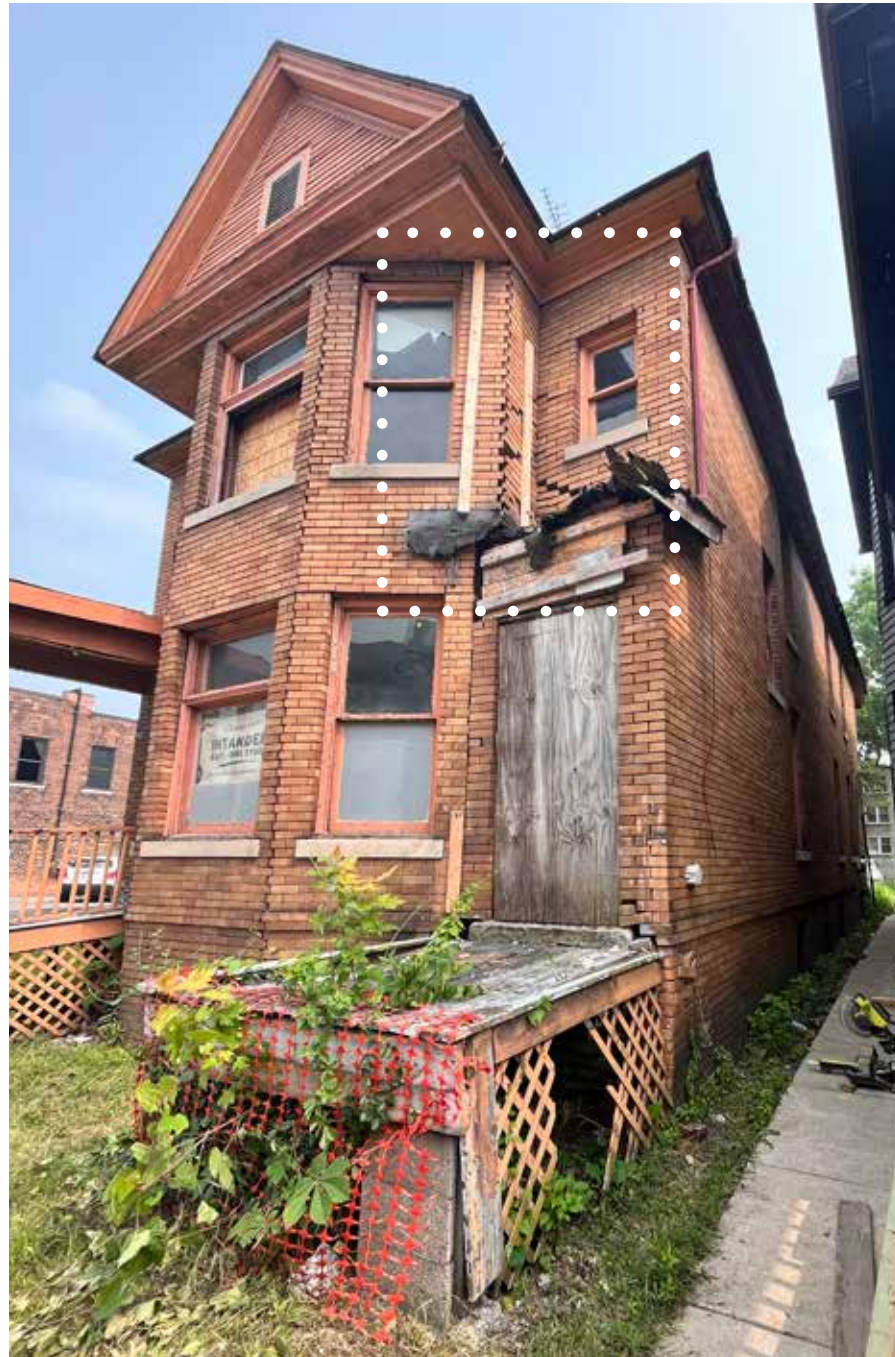
PHOTOS TO THE RIGHT DETAIL THE SECOND LEVEL BRICK CONDITION AT THE WEST SIDE OF FRONT FACADE WHERE THE POINT OF FAILURE BEGAN
