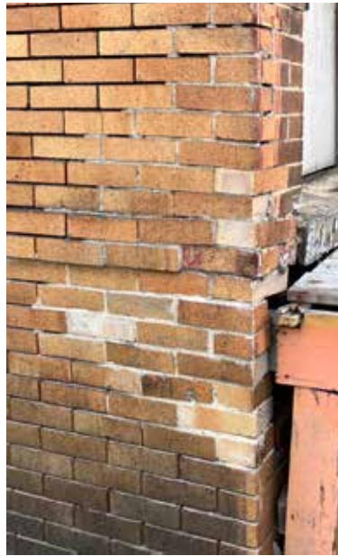
A. Poor patching of failing bricks at East front entry
