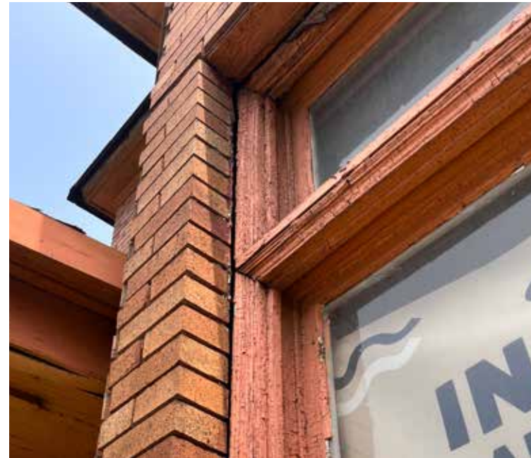
BRICK CONDITION AT SECOND LEVEL EAST SIDE OF FRONT BAY SHOWING BRICK DETACHED FROM STRUCTURE VIA GAP BETWEEN BRICKMOLD
