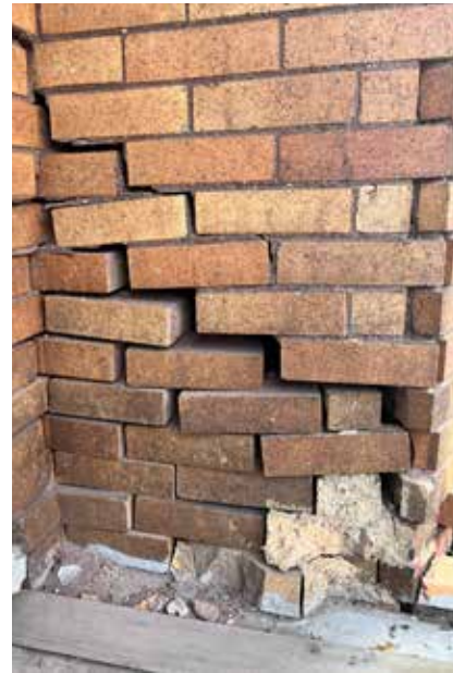
B. Loose and failing bricks at East entry/bay
