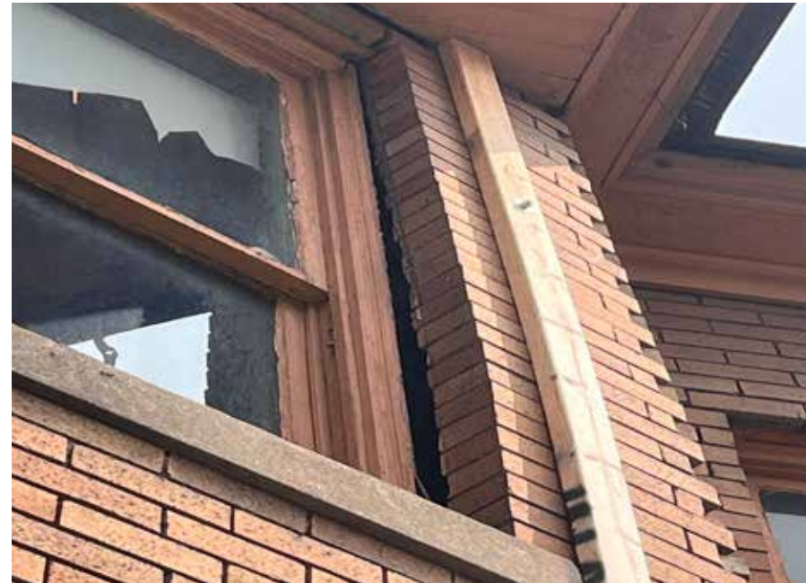
DETACHED BRICK VENEER AT WEST SIDE OF FRONT BAY
