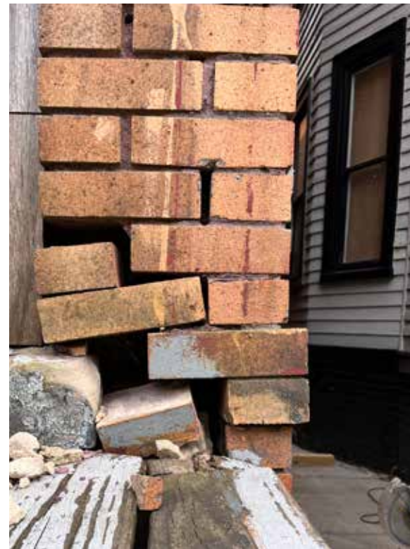
MISSING AND FAILED BRICK AT LOWER PORTION OF WEST ENTRY
