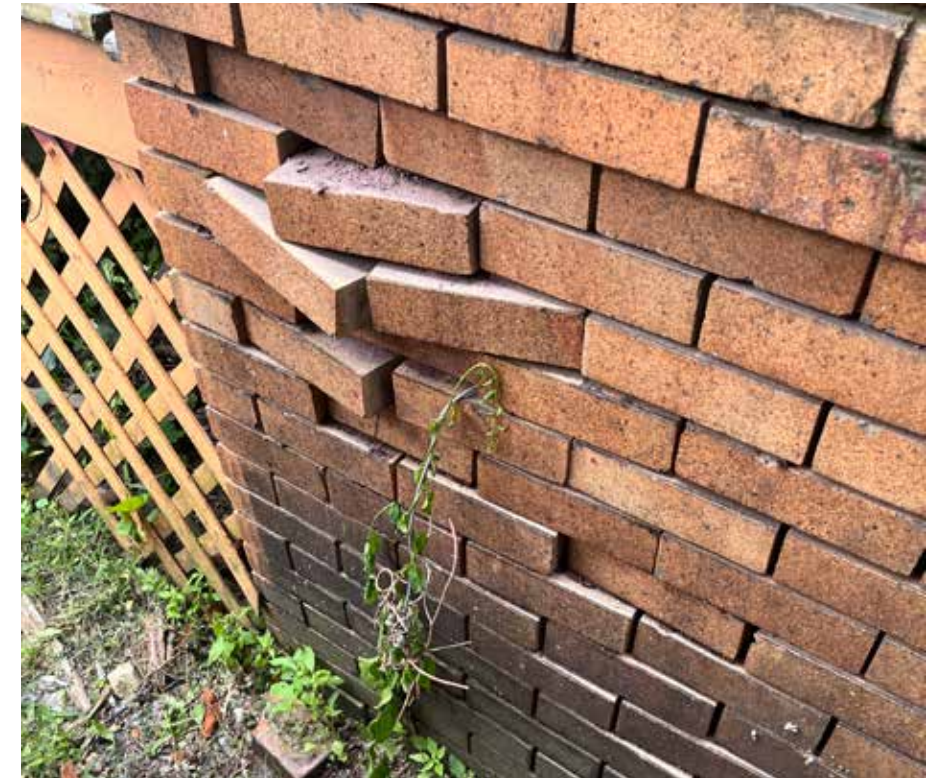
DETACHED BRICK AT FRONT OF WEST ELEVATION
