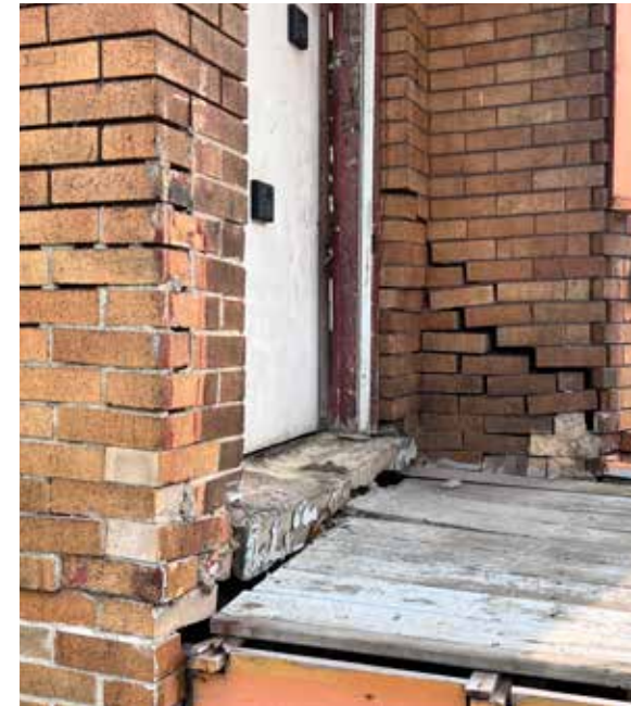
FAILING BRICK VENEER AT WEST FORNT PORCH ENTRY
