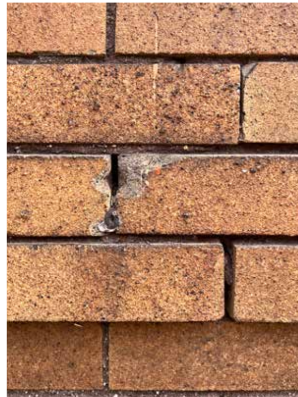
BRICK DETAIL AT MIDDLE OF FRONT BAY WITH MISSING MORTAR
