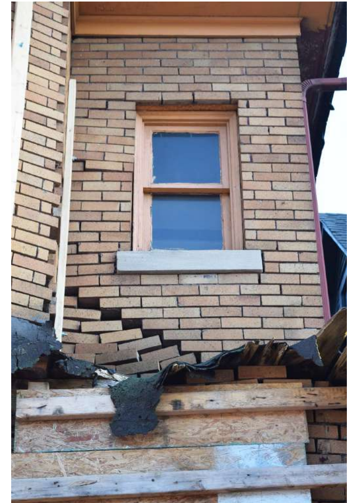
SIGNIFICANT BRICK REPAIR AND REPLACEMENT IS REQUIRED AT FRONT FACADE
