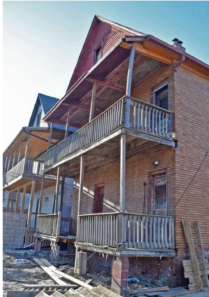
DETERIORATING STRUCTURE AT REAR PORCH AND BALCONY
