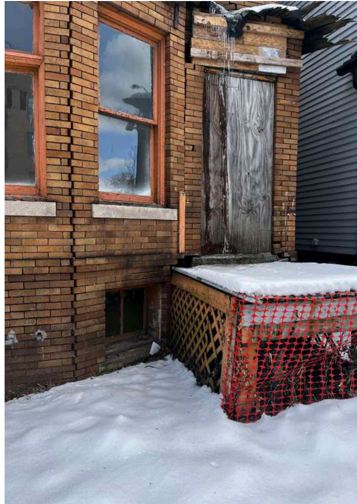
ENTRY PORCH TO SECOND LEVEL UNIT WITH MISSING STAIRS, GUARDRAIL, PORCH ROOF, DOOR AND FRAME
