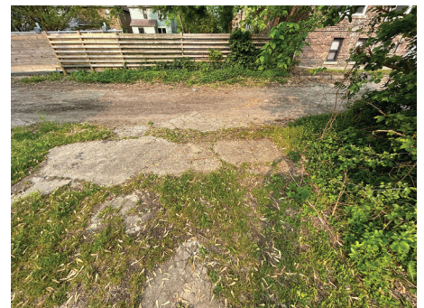
Existing dilapidated cement pad.
