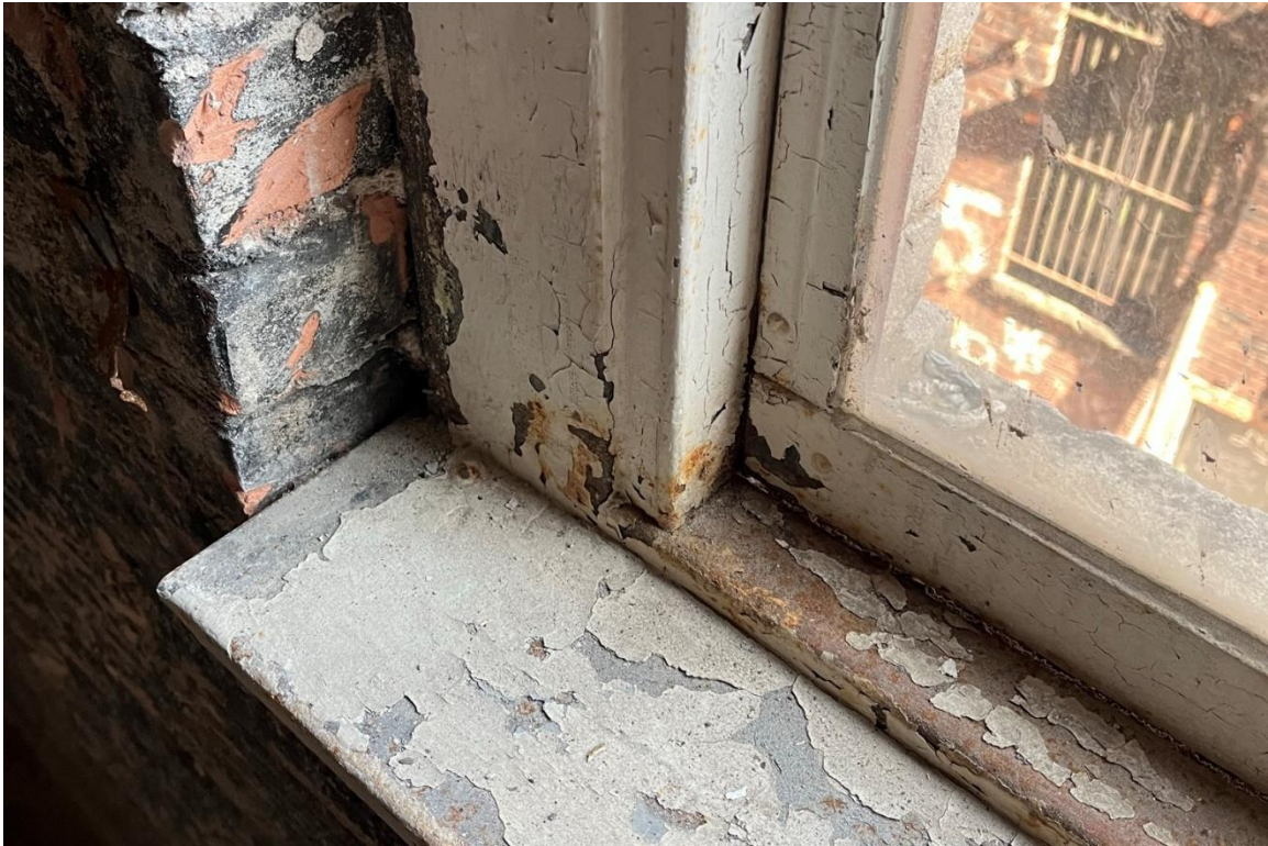
Window #32, 2 nd Floor, South elevation, 04/03/23.
