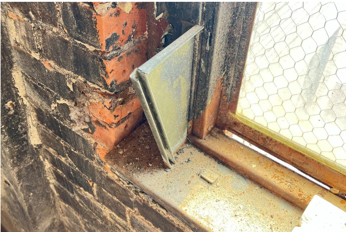
Window #11, 8 th Floor, East elevation, 04/03/23.
