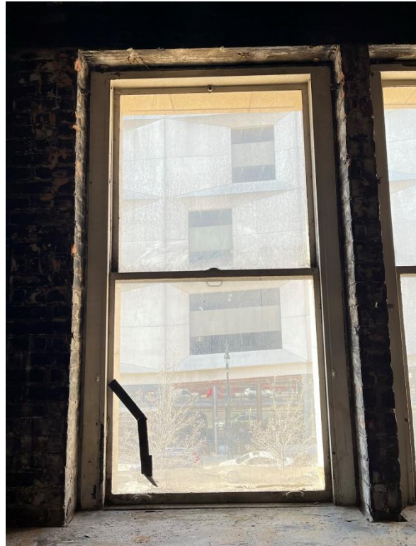
Window #32, 2 nd Floor, South elevation, 04/03/23.
