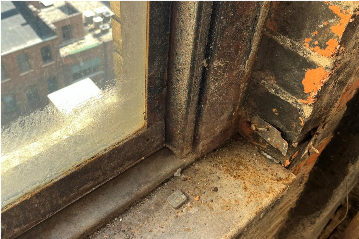
Window #2, 10 th Floor, North courtyard elevation, 04/03/23.
