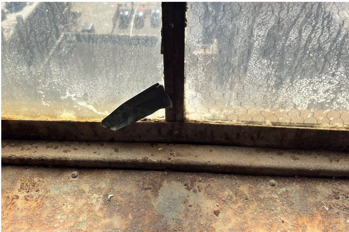
Window #6, 9 th Floor, East elevation, 04/03/23.
