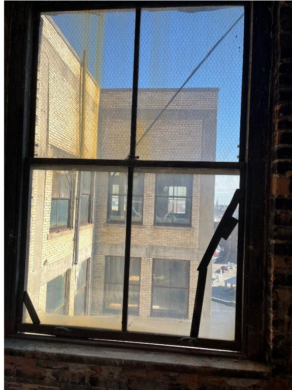
Window #2, 10 th Floor, North courtyard elevation, 04/03/23.
