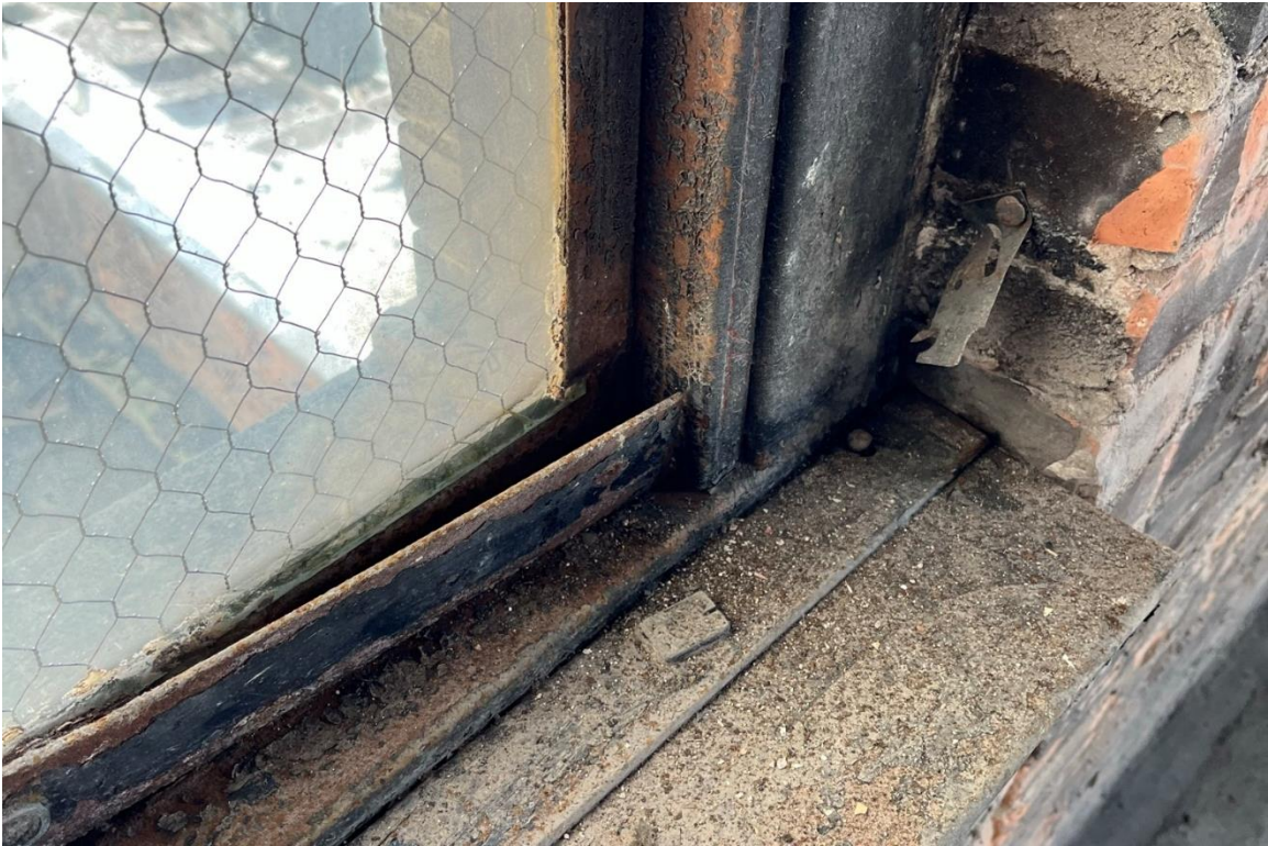
Window #23, 5 th Floor, North courtyard elevation, 04/03/23.
