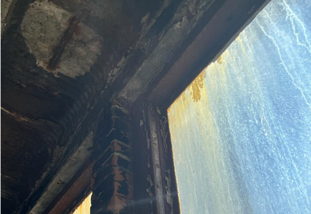
Window #6, 9 th Floor, East elevation, 04/03/23.
