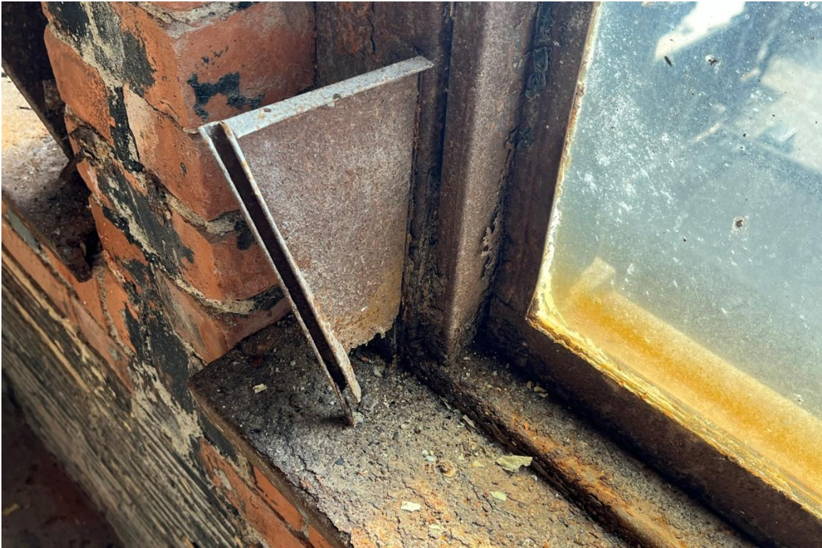
Window #6, 9 th Floor, East elevation, 04/03/23.
