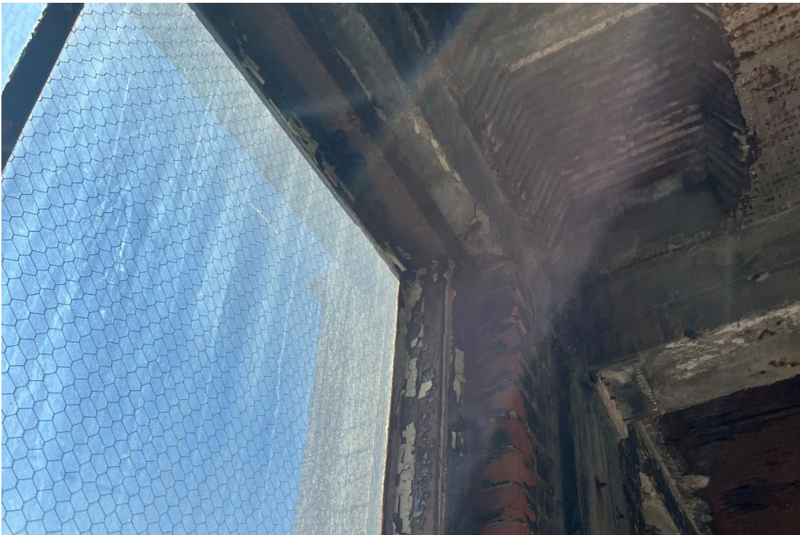
Window #6, 9 th Floor, East elevation, 04/03/23.
