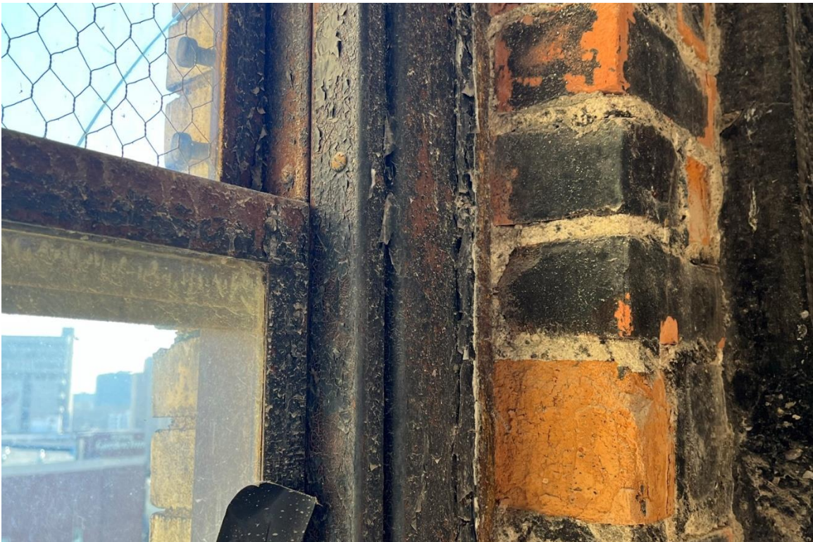
Window #2, 10 th Floor, North courtyard elevation, 04/03/23.
