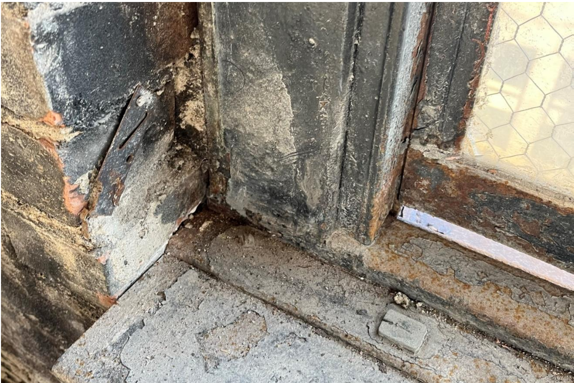
Window #15, 7 th Floor, North courtyard elevation, 04/03/23.
