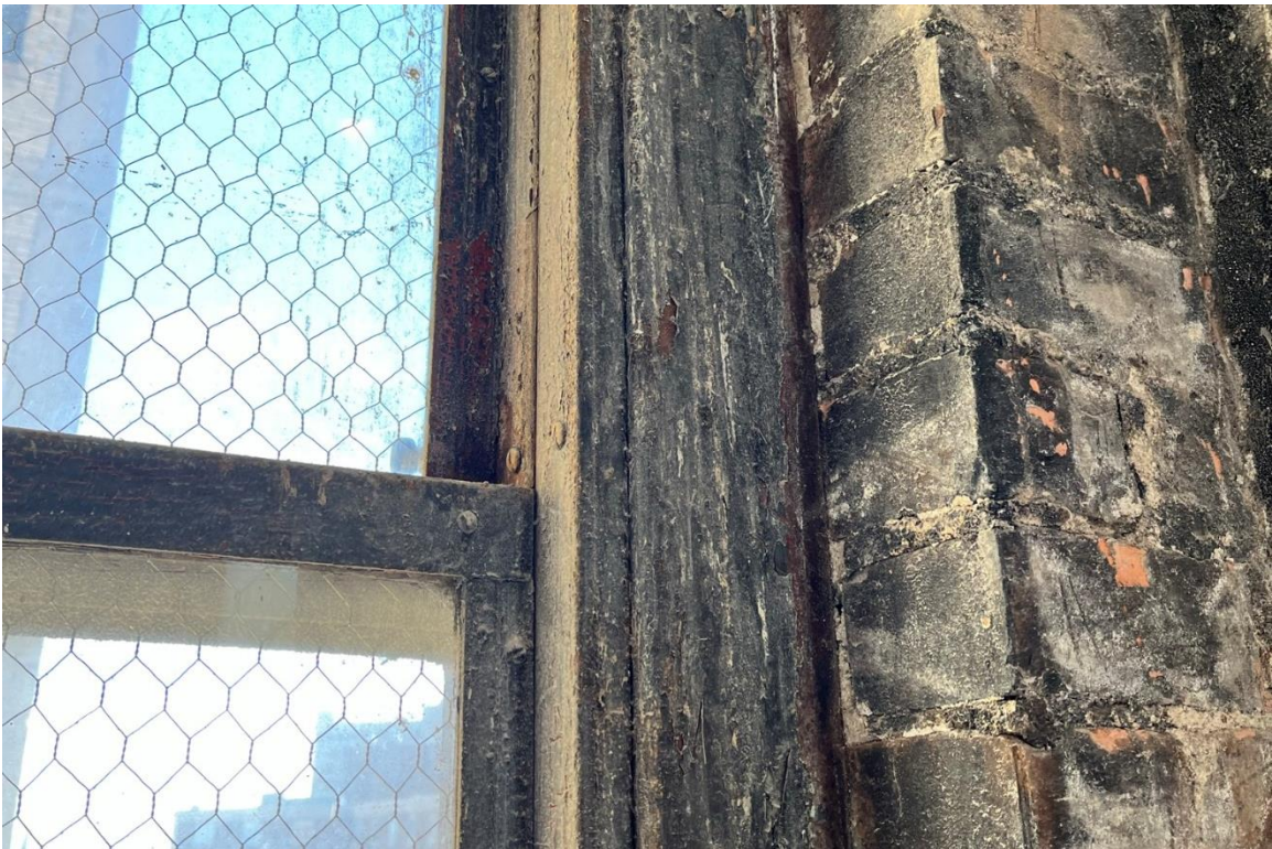
Window #15, 7 th Floor, North courtyard elevation, 04/03/23.
