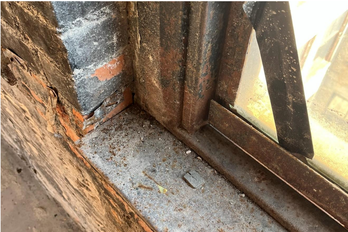
Window #2, 10 th Floor, North courtyard elevation, 04/03/23.
