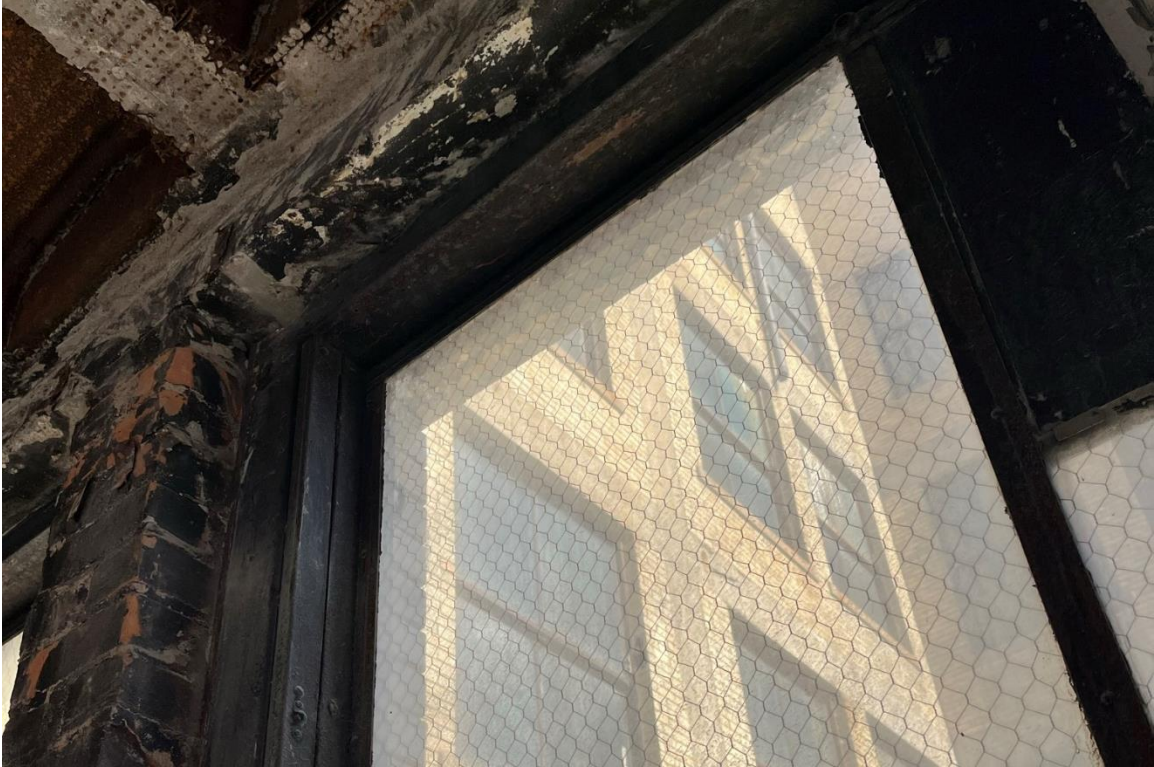
Window #15, 7 th Floor, North courtyard elevation, 04/03/23.
