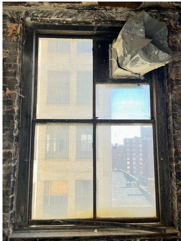
Window #15, 7 th Floor, North courtyard elevation, 04/03/23.
