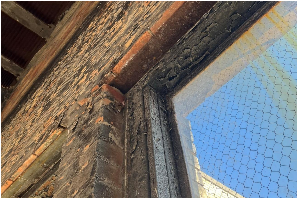
Window #2, 10 th Floor, North courtyard elevation, 04/03/23.
