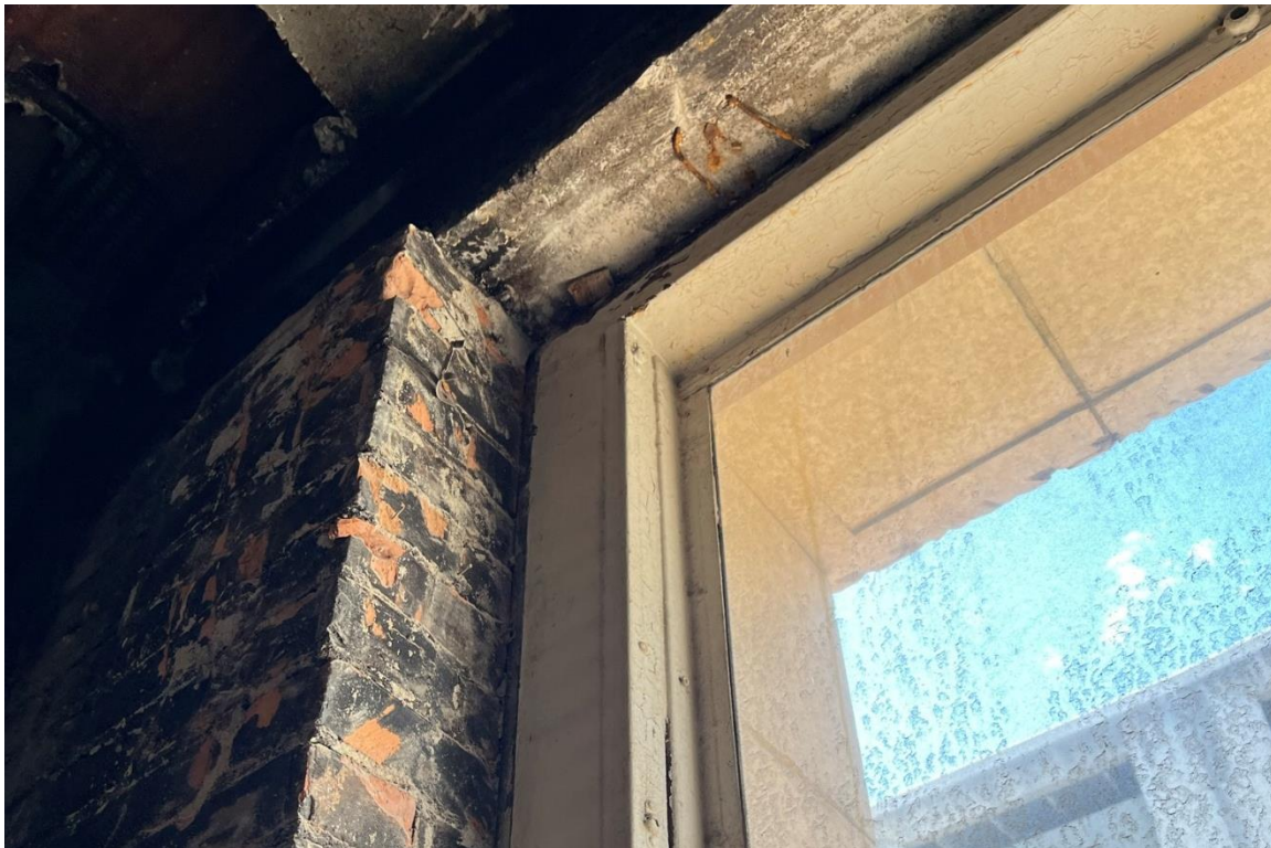
Window #32, 2 nd Floor, South elevation, 04/03/23.
