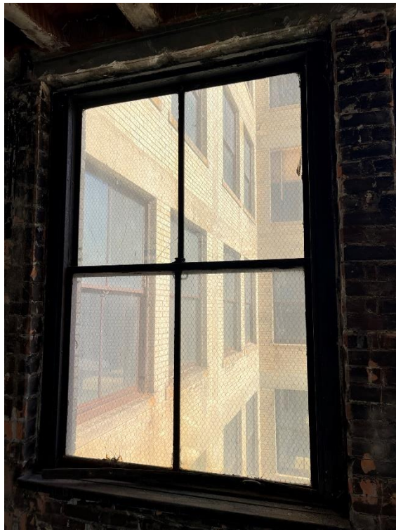
Window #23, 5 th Floor, North courtyard elevation, 04/03/23.
