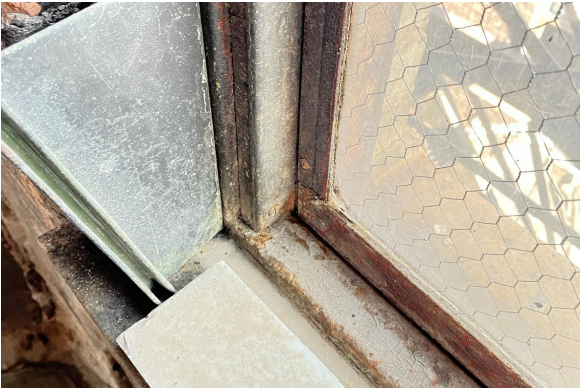
Window #28, 4 th Floor, North elevation, 04/03/23.
