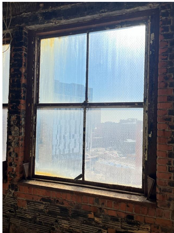
Window #6, 9 th Floor, East elevation, 04/03/23.
