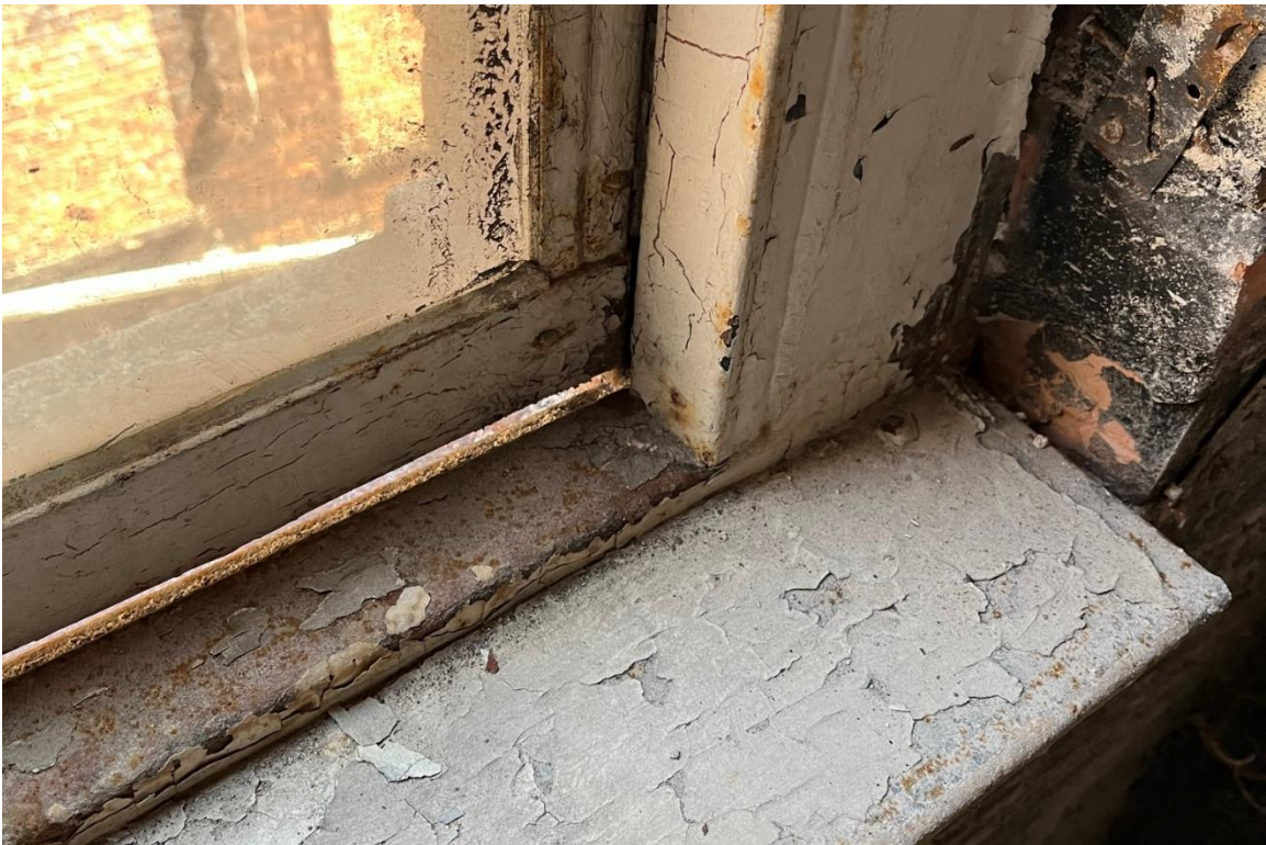
Window #32, 2 nd Floor, South elevation, 04/03/23.
