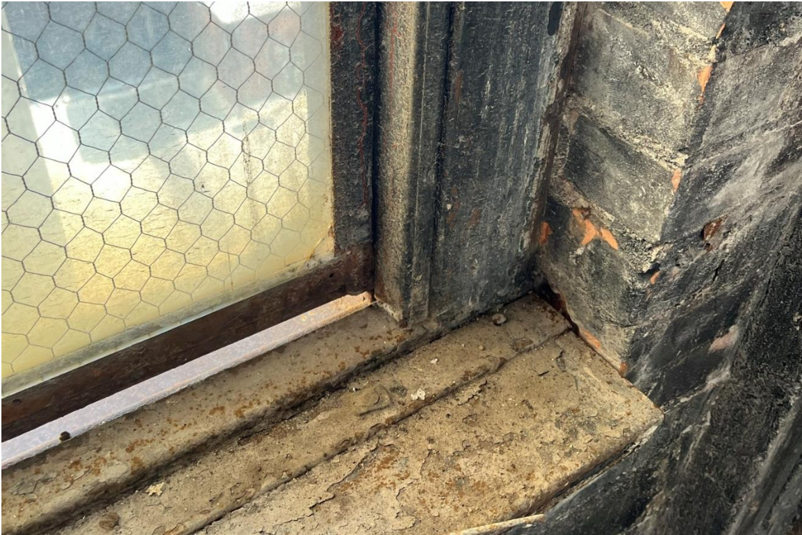
Window #15, 7 th Floor, North courtyard elevation, 04/03/23.
