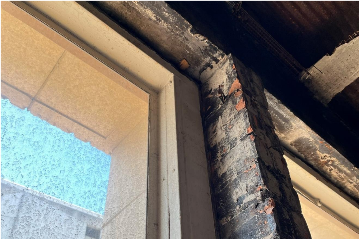
Window #32, 2 nd Floor, South elevation, 04/03/23.
