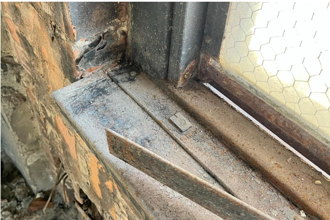
Window #23, 5 th Floor, North courtyard elevation, 04/03/23.
