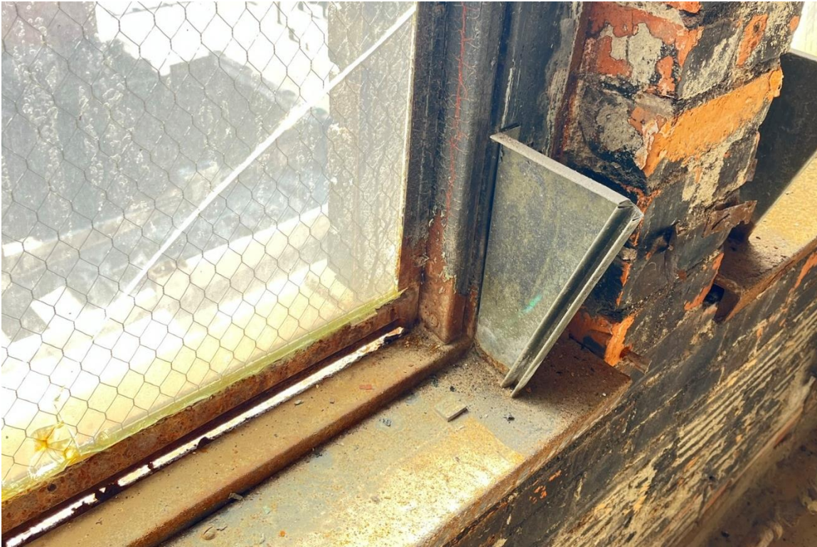
Window #11, 8 th Floor, East elevation, 04/03/23.
