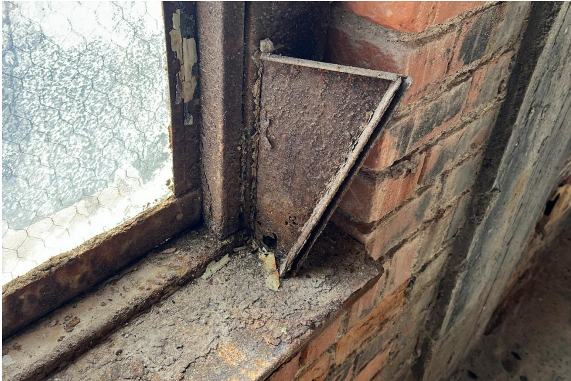
Window #6, 9 th Floor, East elevation, 04/03/23.
