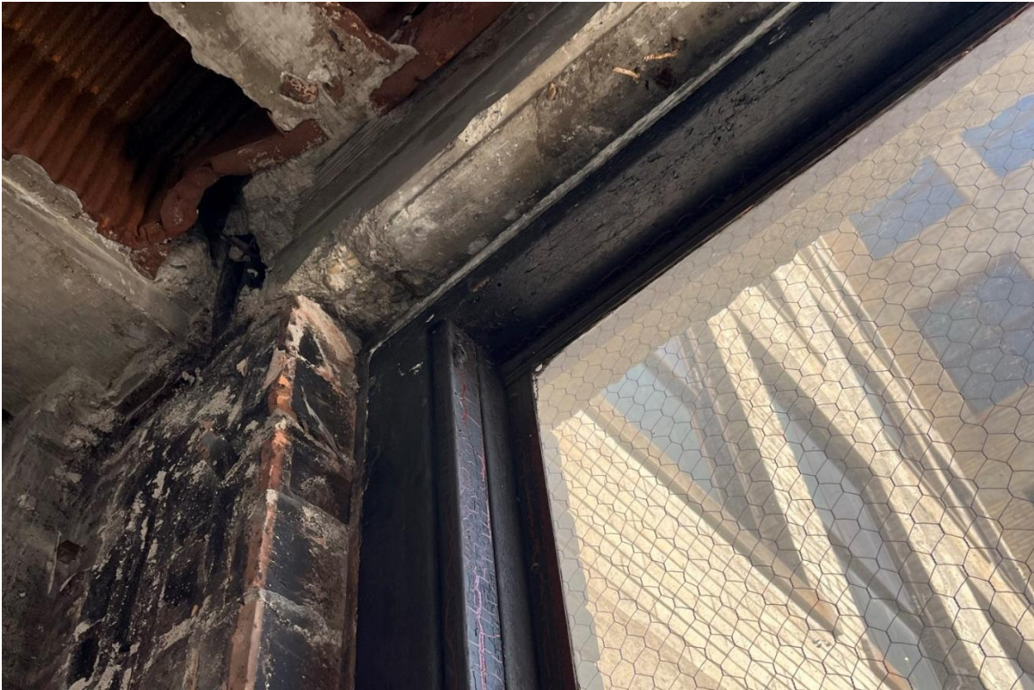
Window #23, 5 th Floor, North courtyard elevation, 04/03/23.
