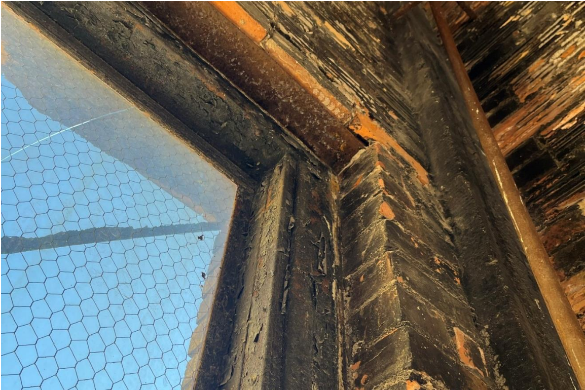
Window #2, 10 th Floor, North courtyard elevation, 04/03/23.
