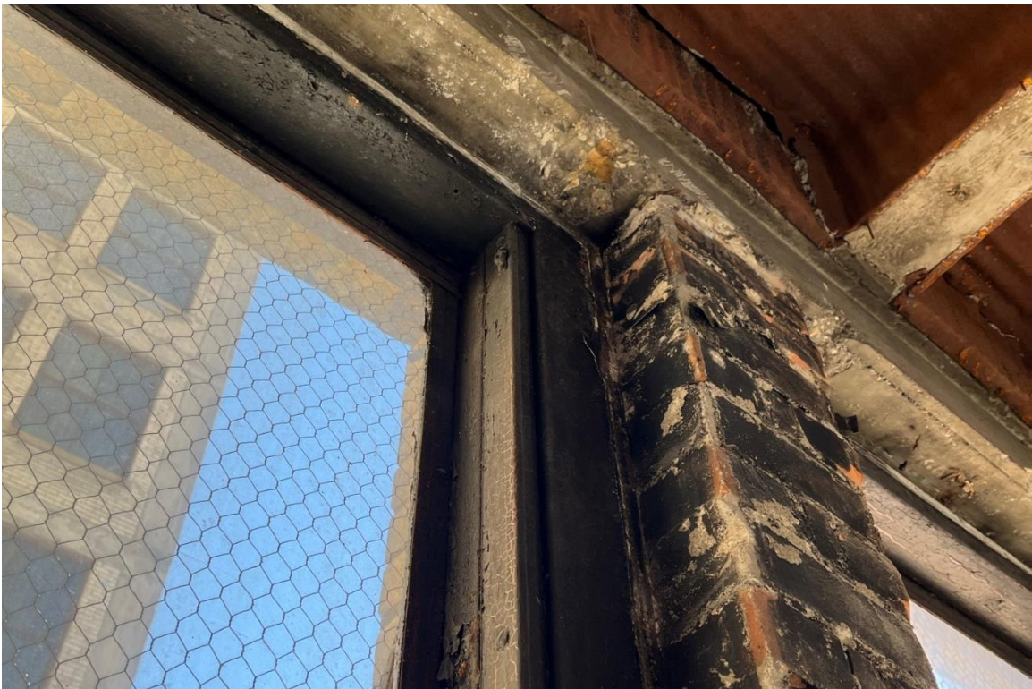
Window #23, 5 th Floor, North courtyard elevation, 04/03/23.
