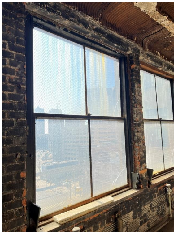
Window #11, 8 th Floor, East elevation, 04/03/23.
