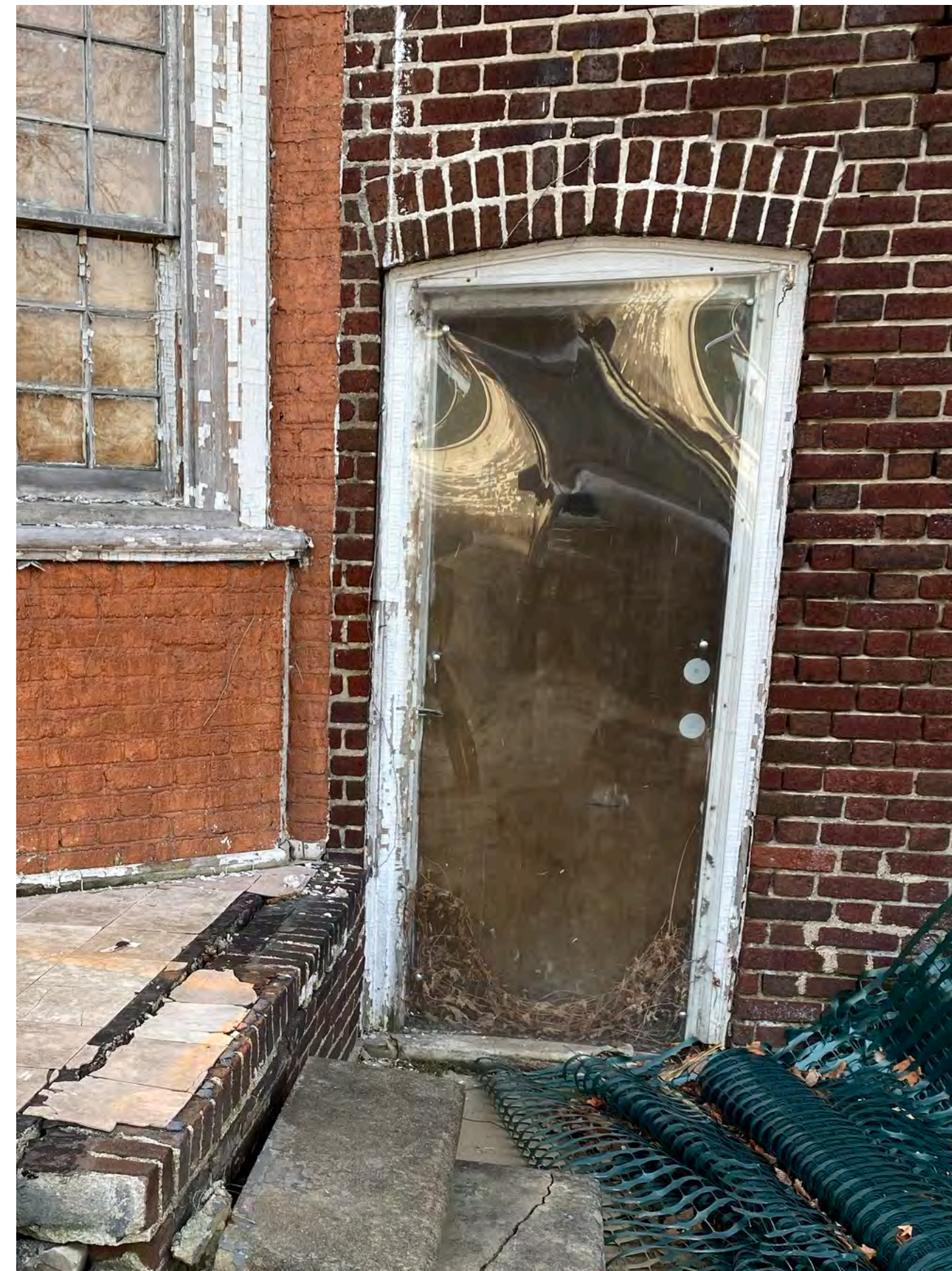
DOOR A - NEW DOOR SILL HEIGHT AND DOOR (103) FOR RESIDENTIAL TENANTS - SEE DOOR SCHEDULE FOR DETAILS
