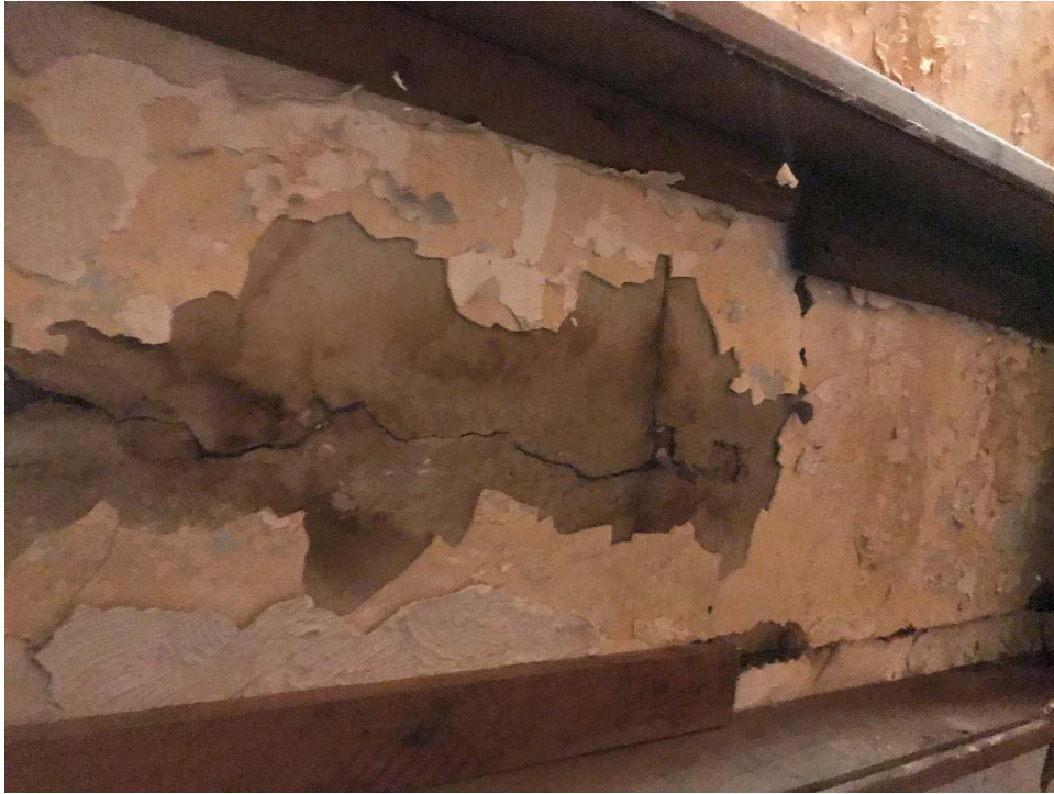
Fig 37: Basement ceiling beam with visible cracking in plaster finish
