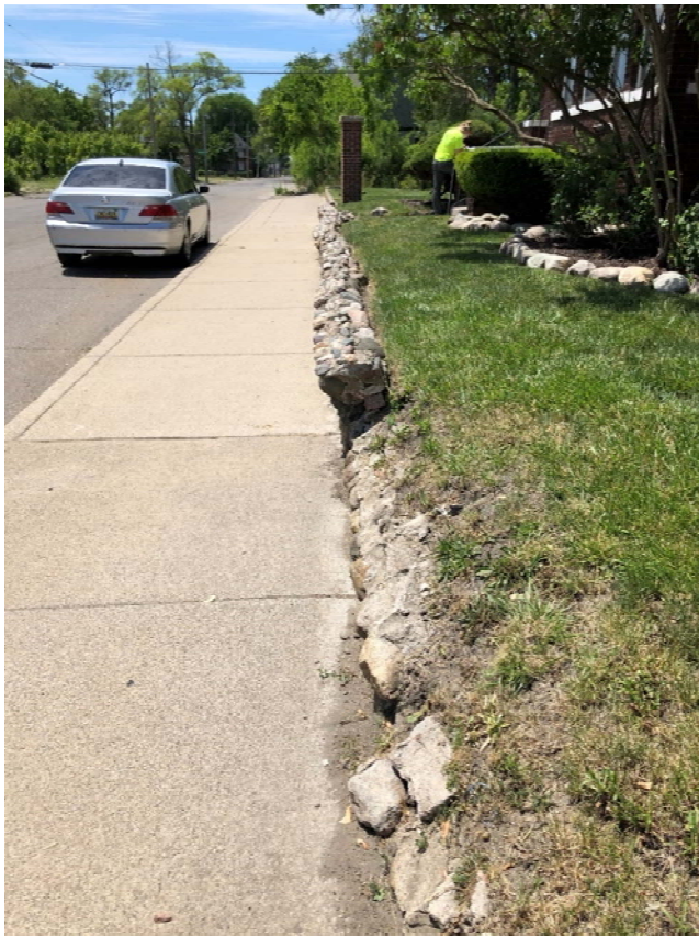
Figure 24 Retaining walls visibly rotated away from site, along Charlevoix Street
