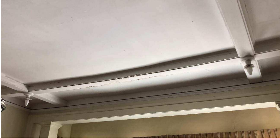
Figure 8 Sagging of second-floor framing
