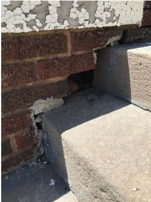
Fig 05: Dislodged masonry units adjacent to the Side Entry stair along south elevation (Charlevoix)
