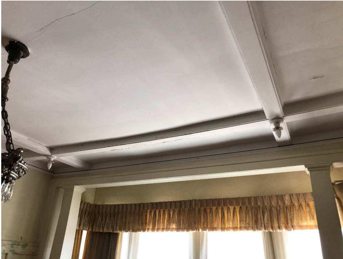
Figure 4 Ceiling and Soffit at First Floor where dining room extends toward the south
