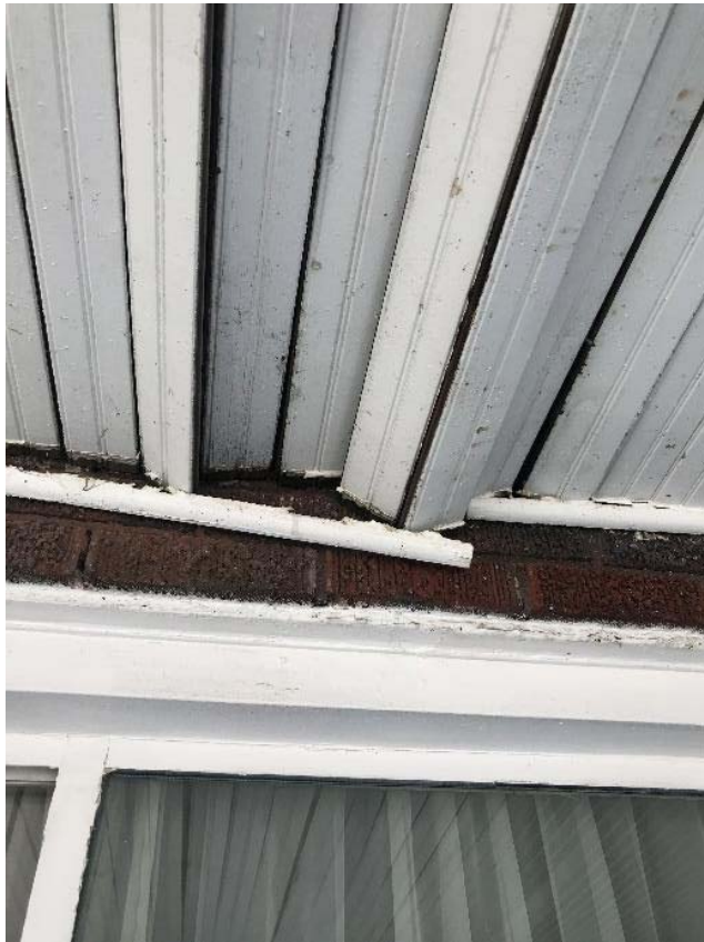
Fig 18: Typical example of beadboard ceiling condition and broken quarter round crown molding
