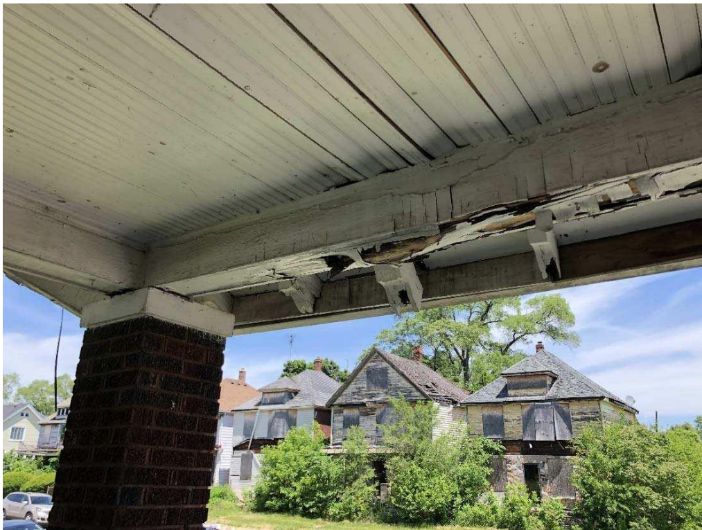
Figure 15 Deteriorated porch beam
