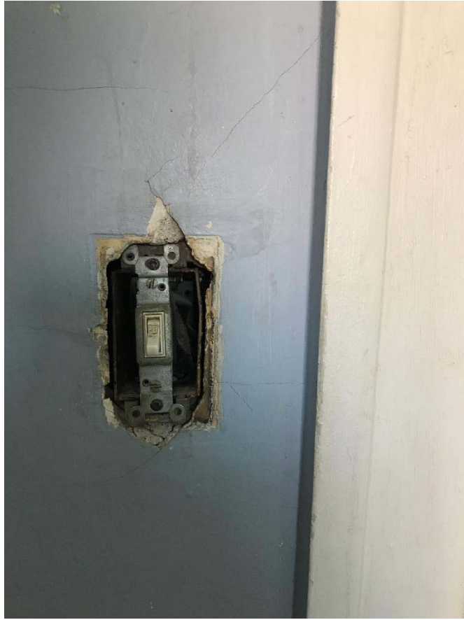
Fig 43: Typical example of missing switch plates with and adjacent damaged plaster seen throughout house
