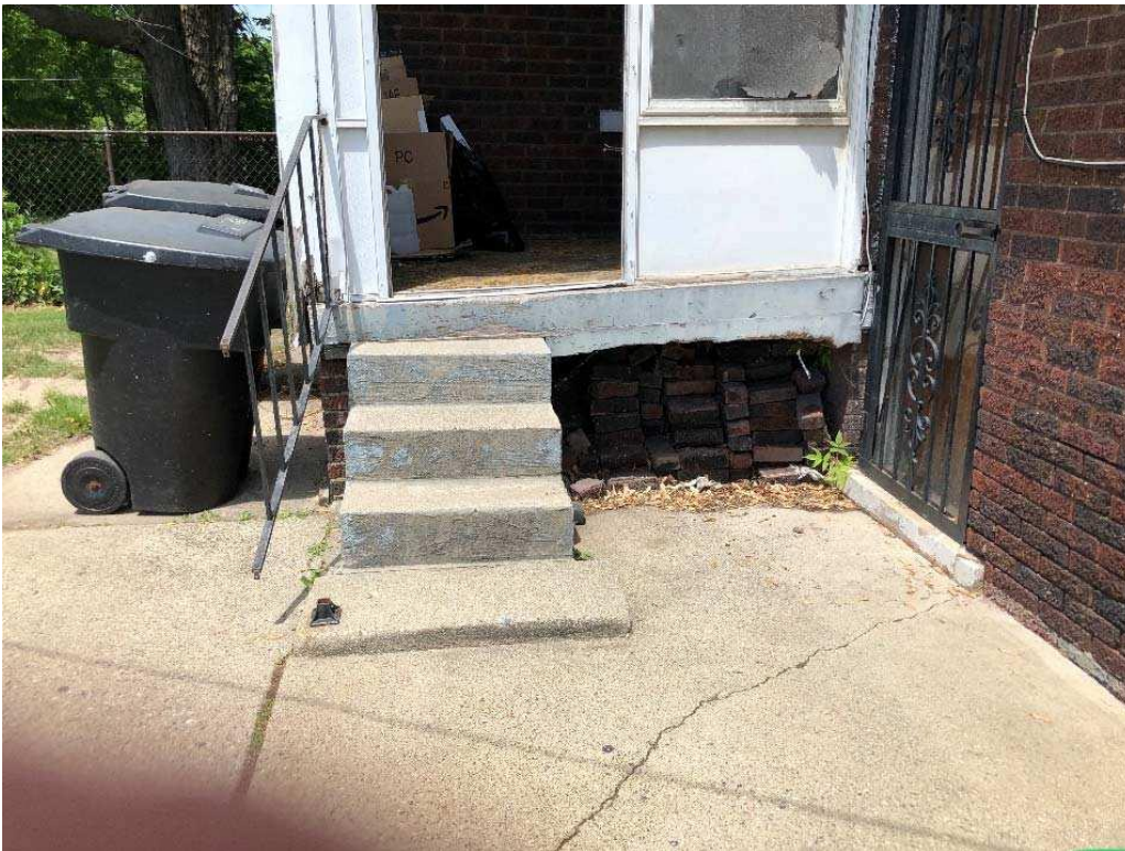
Figure 18 Landing framing at back of back porch with visible sagging toward the west
