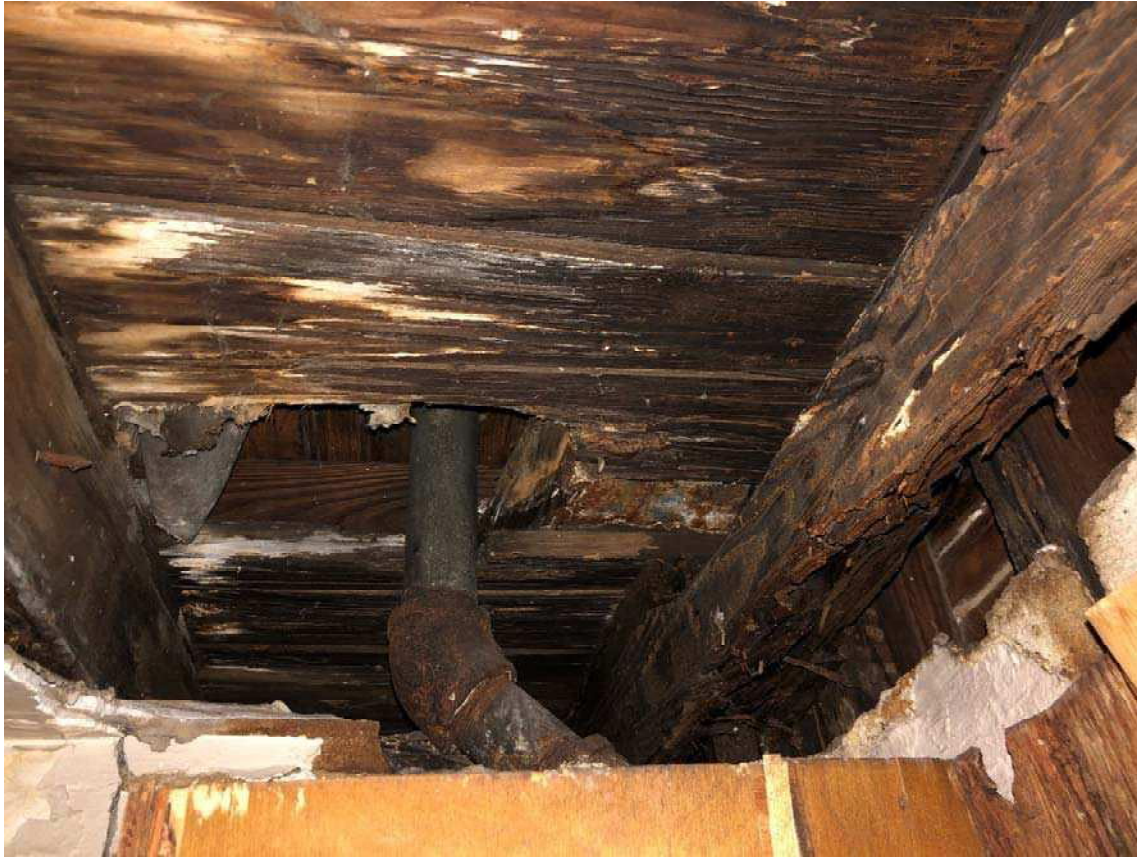
Figure 7 Water-damaged second floor beams below second floor bathroom
