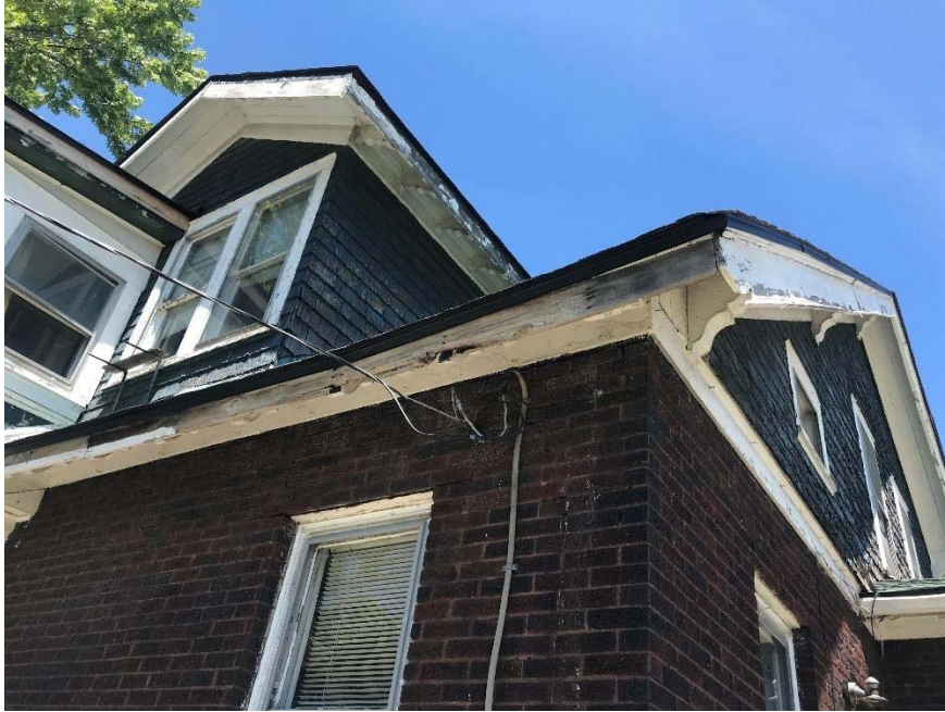
Fig 24: Missing gutter along roof edge on west elevation
