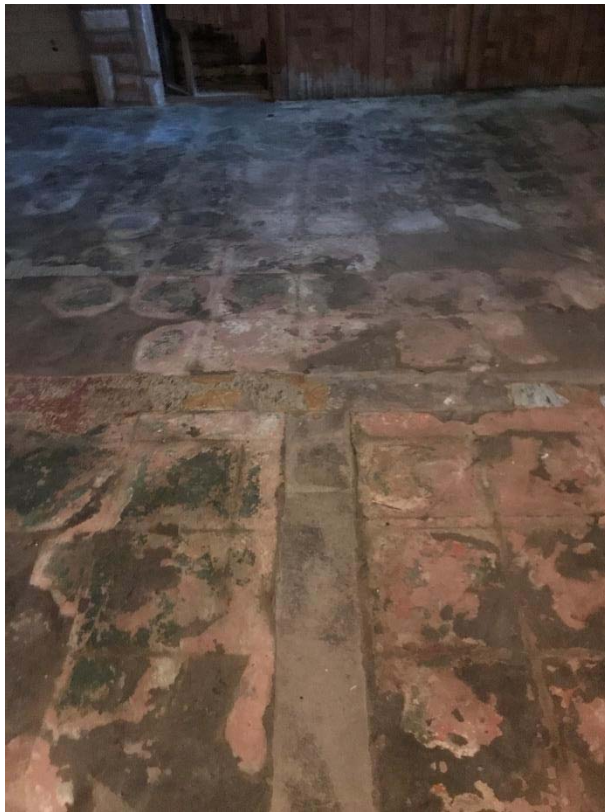
Fig 29: Remnants of vinyl tile flooring and ghost of previous walls in basement
