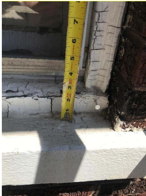
Fig 11: Typical signs of flaking paint and wood decay as well as miscellaneous nails in wood frames
