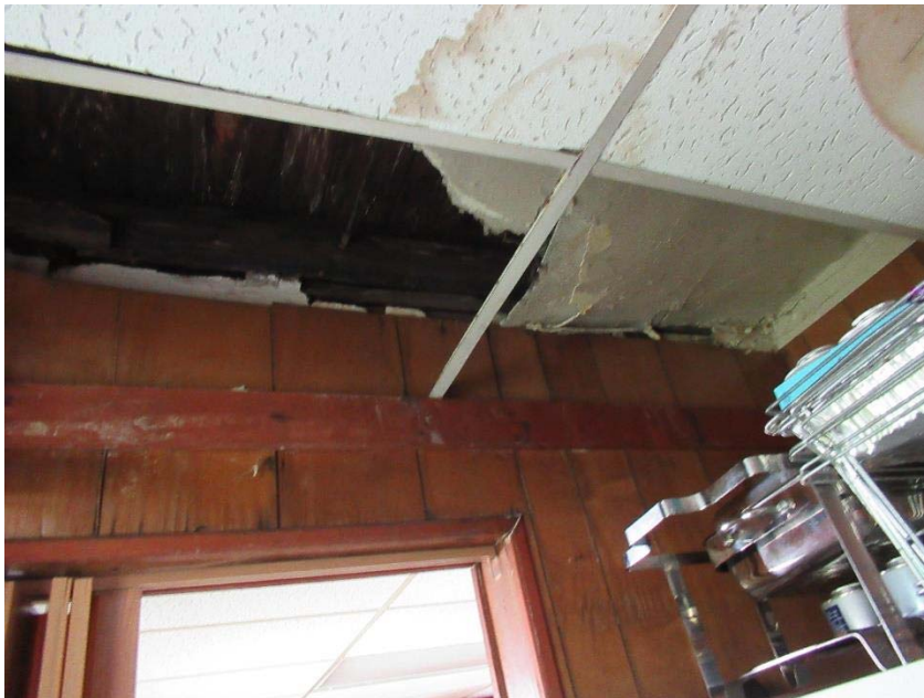
Fig 40: Damaged plaster ceiling visible above missing acoustic ceiling tiles in kitchen
