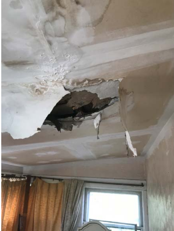
Fig 41: Extensive water damage to gypsum board walls and ceiling in second floor rear enclosed porch
