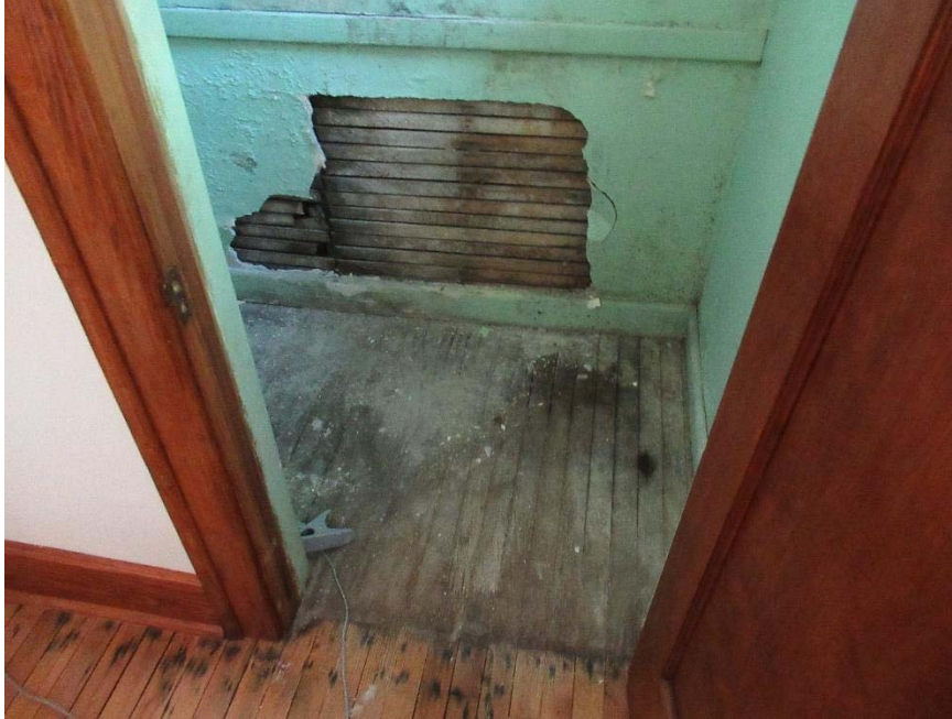
Fig 32: Exposed wood plank subfloor in closet adjacent to first floor parlor. Floor exhibits signs of water damage
