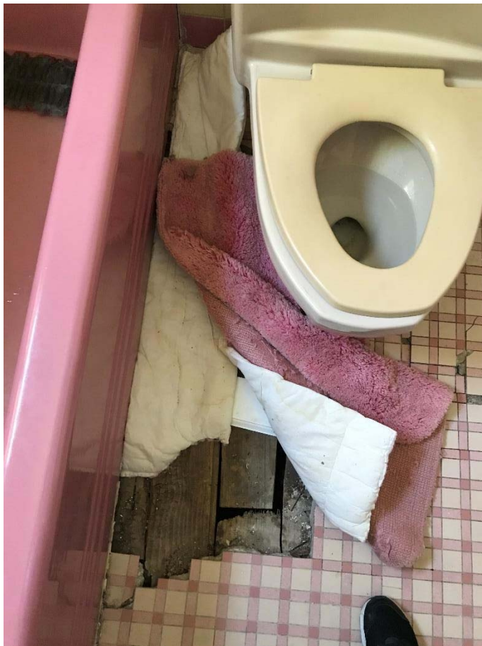
Fig 33: Missing and damaged tile and damaged wood plank subfloor in second floor bathroom
