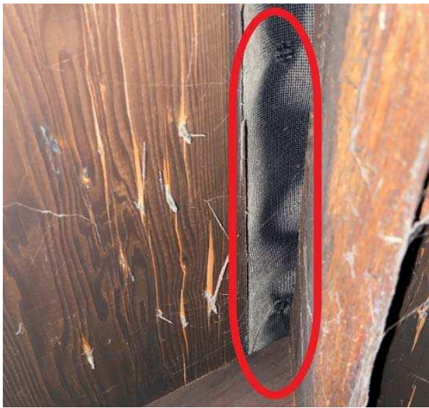
Figure 10 Unsealed roof apex
