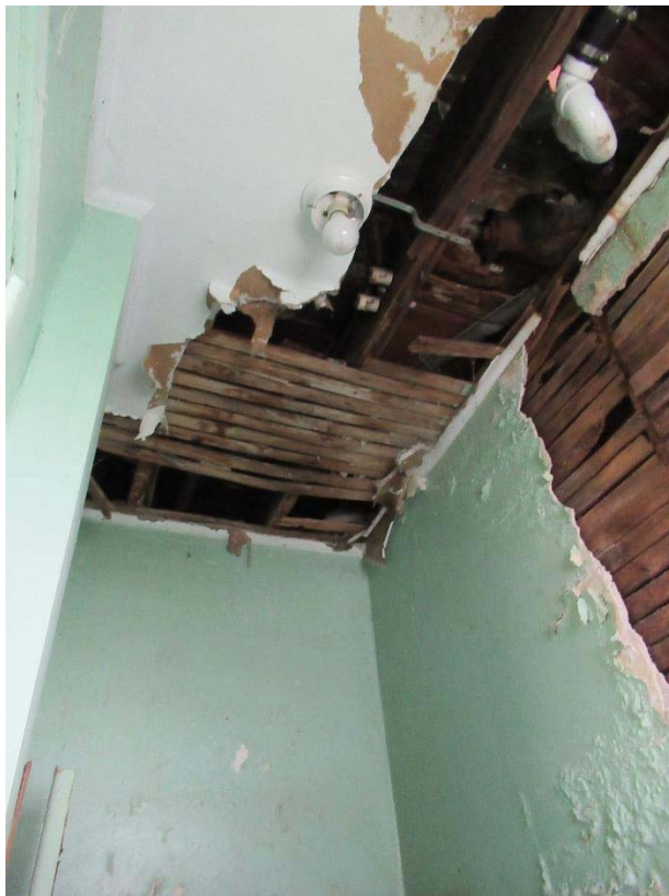
Fig 38: Water damage and subsequent structural damage in first floor parlor closet
