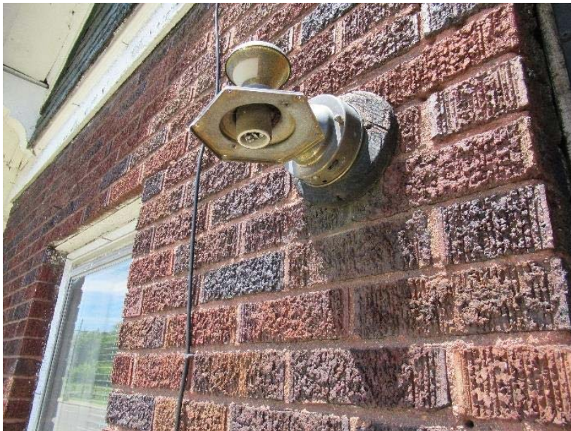
Fig 27: Exterior light fixture at side entry
