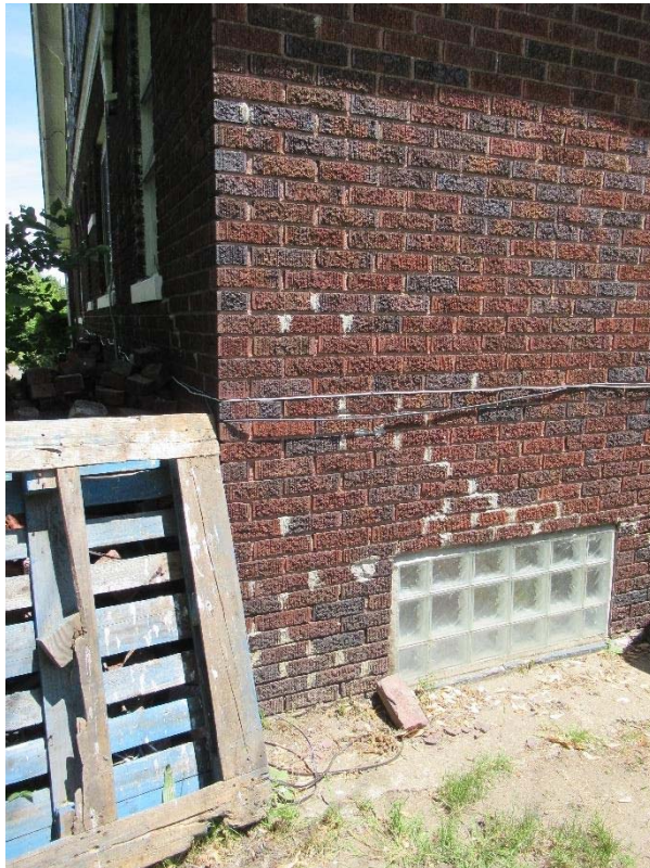
Fig 07: Typical appearance of past repointing efforts
