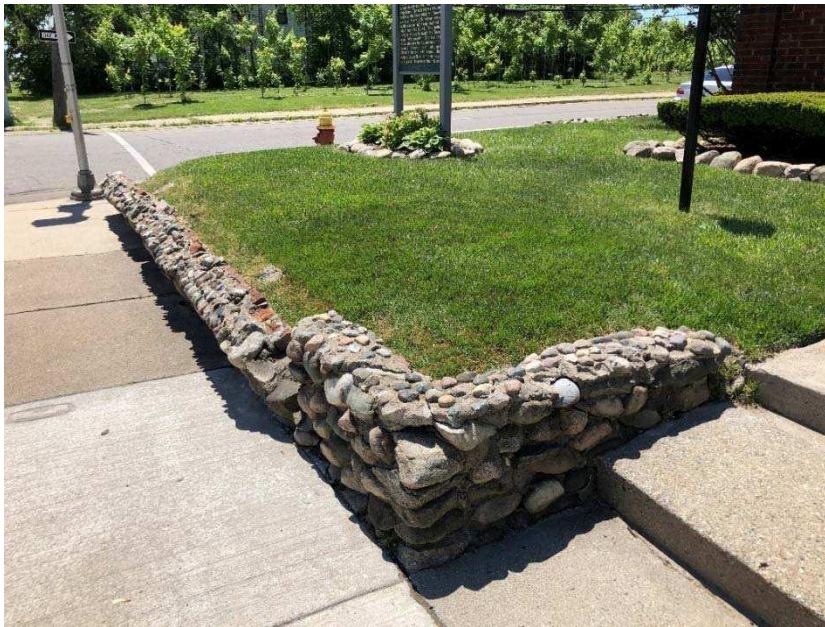
Figure 23 Retaining walls visibly rotated away from site, along Garland Avenue
