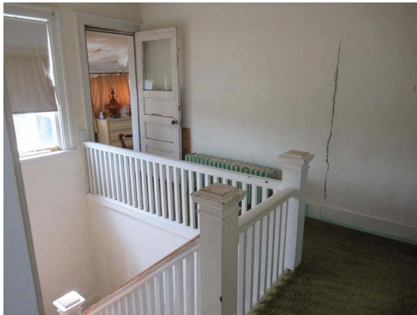
Fig 44: Cracked and bowing plaster walls visible in second floor corridor
