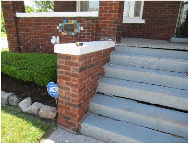
Fig 15: Front stair with large joints due to settlement
