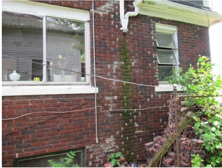
Fig 06: Efflorescence and algae growth on north elevation
