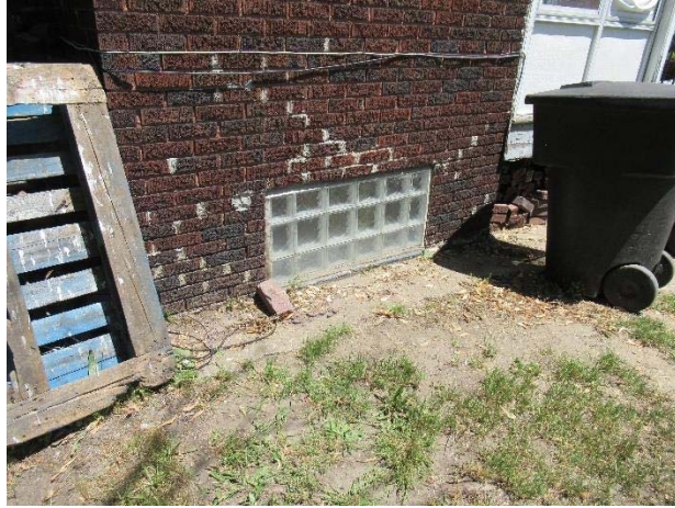
Fig 13: Glass block infill in location of former coal shoot on west elevation. Concrete sill is partially buried by concrete remnants
