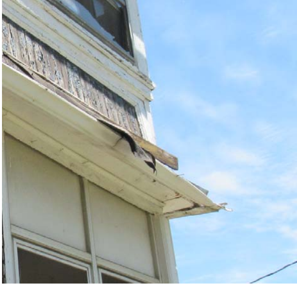
Fig 22: Loose flashing hanging over gutter edge between first and second story of rear porch
