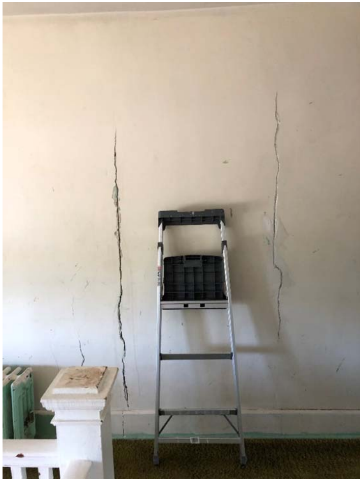
Figure 9 Vertical cracking in plaster wall behind shower/chimney stack
