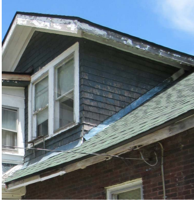
Fig 09: Weathered original fascia board along eave of second story dormer and non-original unpainted replacement fascia board in poor condition along roof eave line
