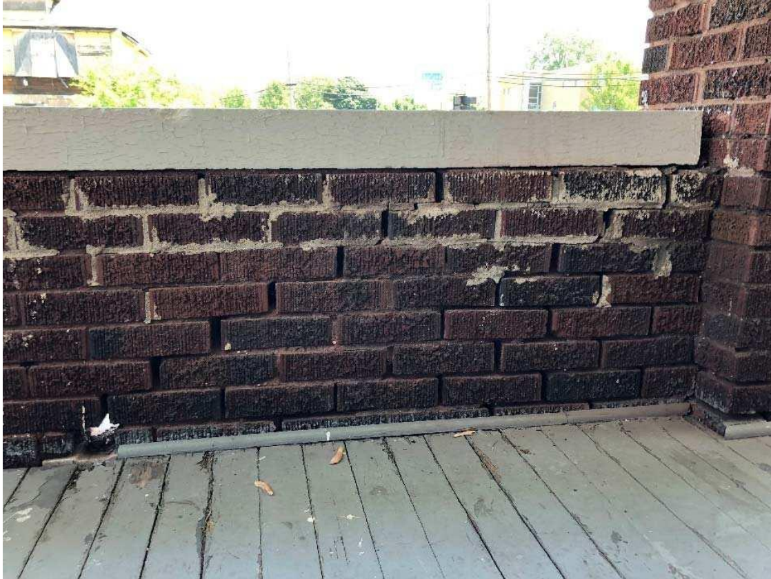
Figure 13 Step cracking and receded mortar on east porch wall (from the porch side)
