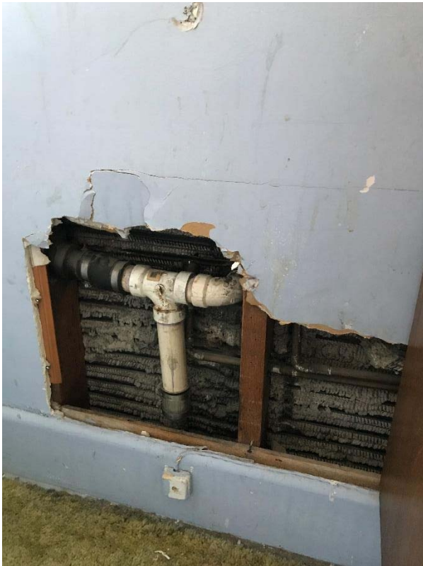
Fig 42: Missing and damaged plaster in second floor bedroom
