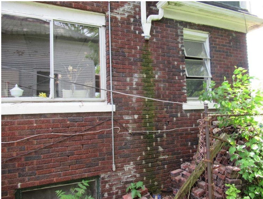
Fig 25: Missing downspout on southern half of north elevation
