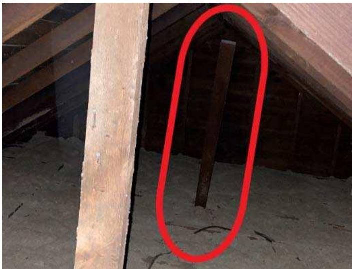
Figure 11 Dislodged framing member
