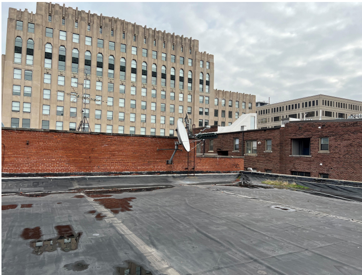
View (B): existing roofing membrane wears away of back of parapet
