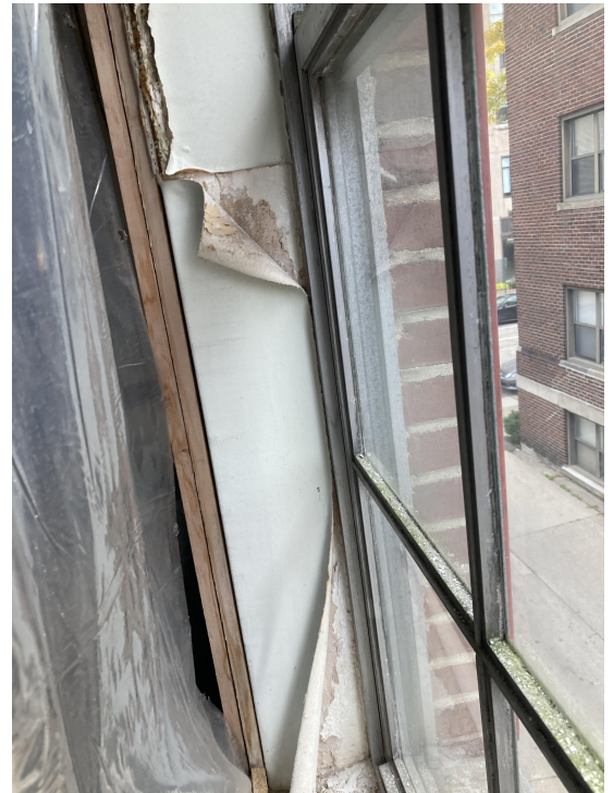
INTERIOR VIEW OF ALUMINUM WINDOWS (W3) SHOWING ADVANCED STAGES OF OXIDIZATION
