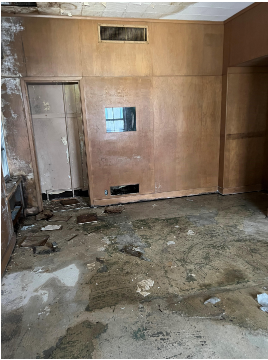
DAMAGED CEILINGS AND WALLS ON THE SECOND FLOOR BECAUSE OF ROOF LEAKS
