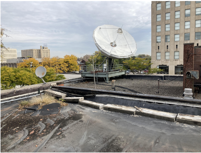
View (A) : existing roof deterioration
