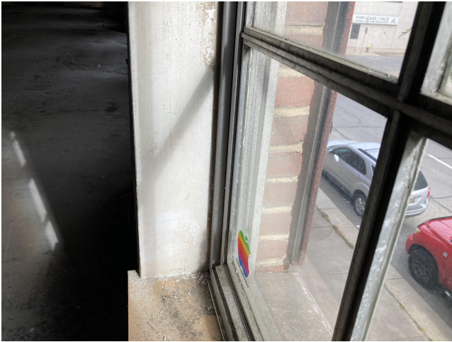
INTERIOR VIEW OF ALUMINUM WINDOW (W2) SHOWING THE INEFFICIENT SINGLE GLAZING
