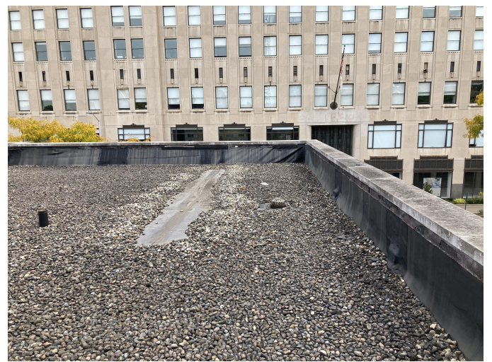
View (D): exposed membrane due to missing gravel protecting layer.
