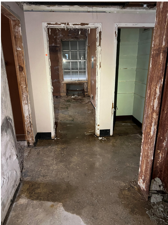
INTERIOR DAMAGES ON THE FIRST FLOOR BECAUSE OF THE LEAKING ROOF
