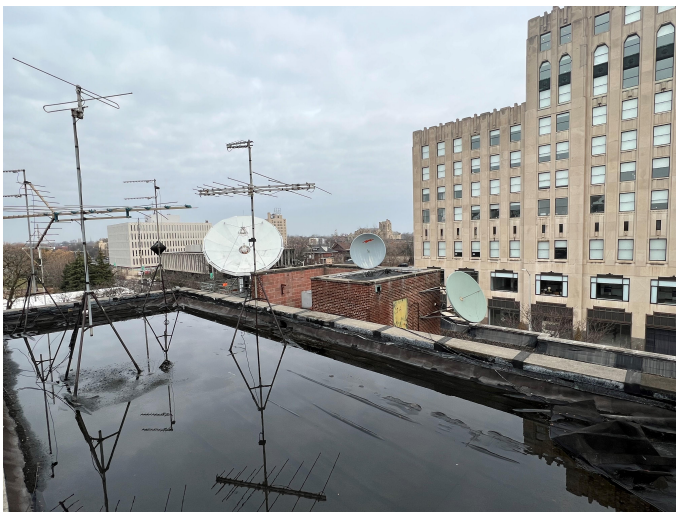
View (C): Water ponds on roof for lack of appropriate slope to drainage
