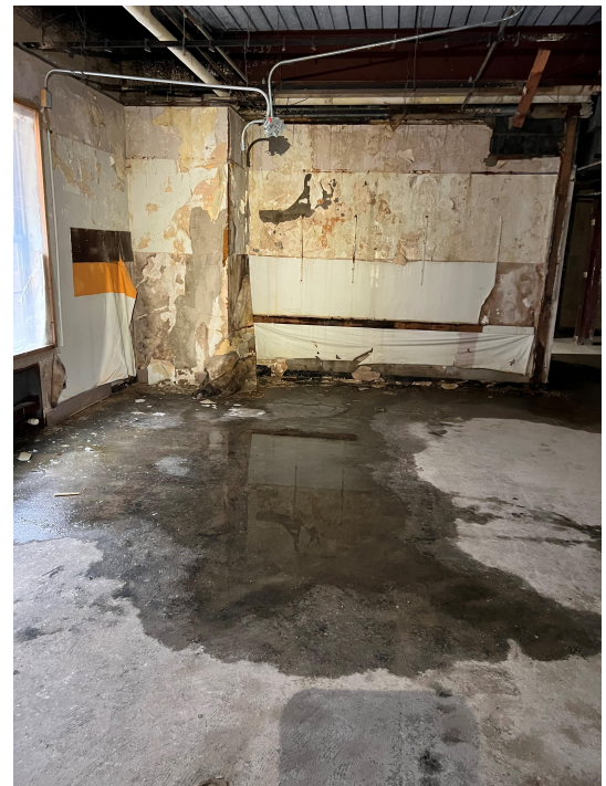
INTERIOR DAMAGES ON THE SECOND FLOOR AS A RESULT OF ROOF WATER LEAKING
