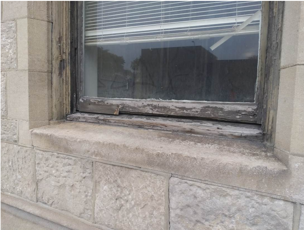
4. Typical deteriorated window sill at stone.
