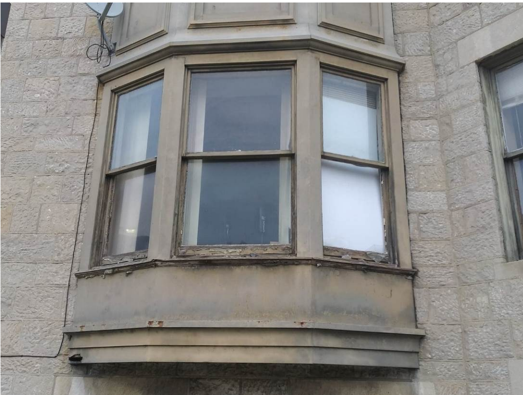
18. South bay window on West Elevation looking east at bay windows (lower).
