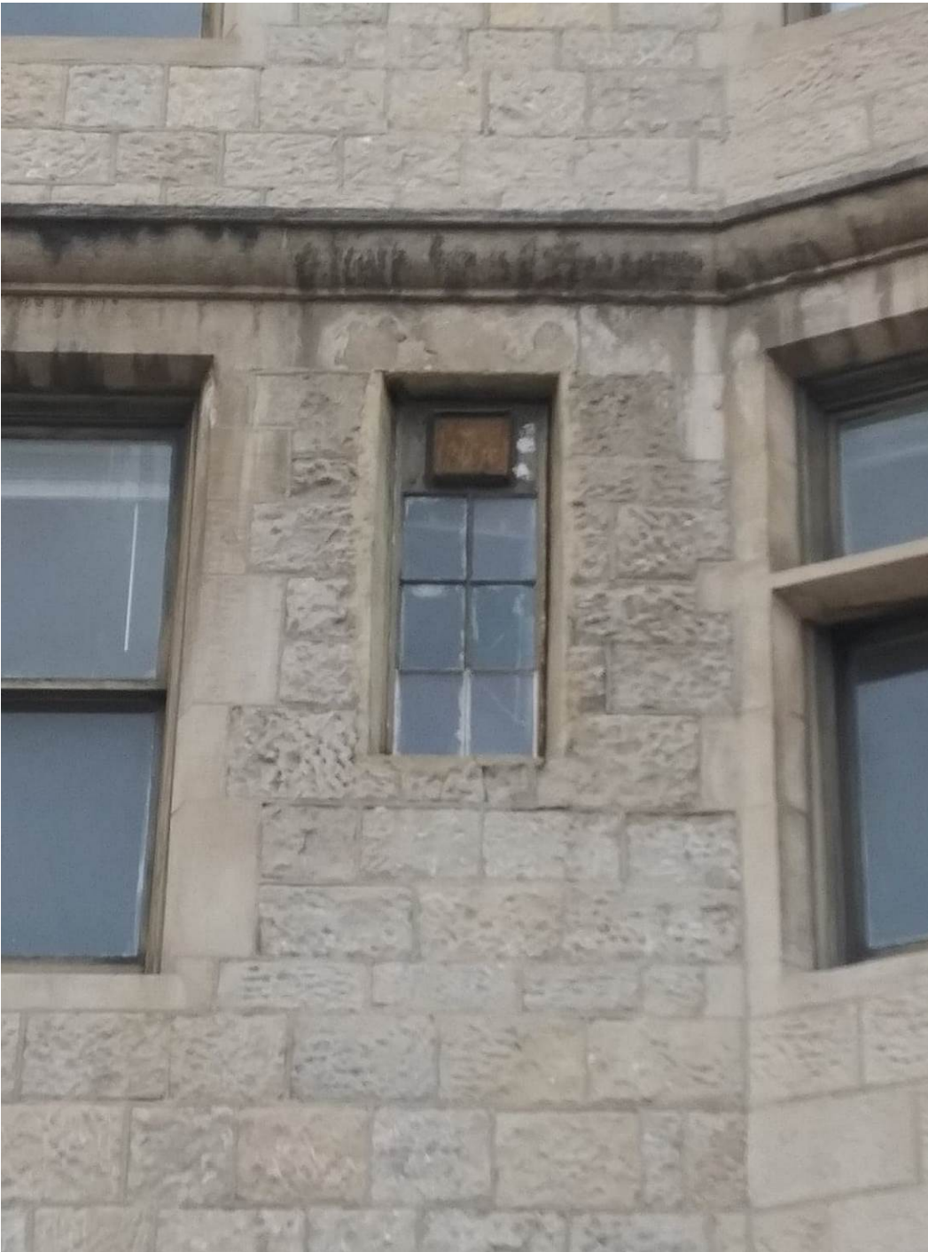
6. East elevation, steel sash window to be removed and replaced.
