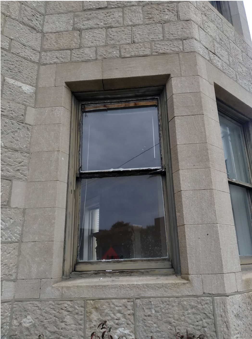
1. Typical deteriorated meeting rail at double hung wood window at stone.
