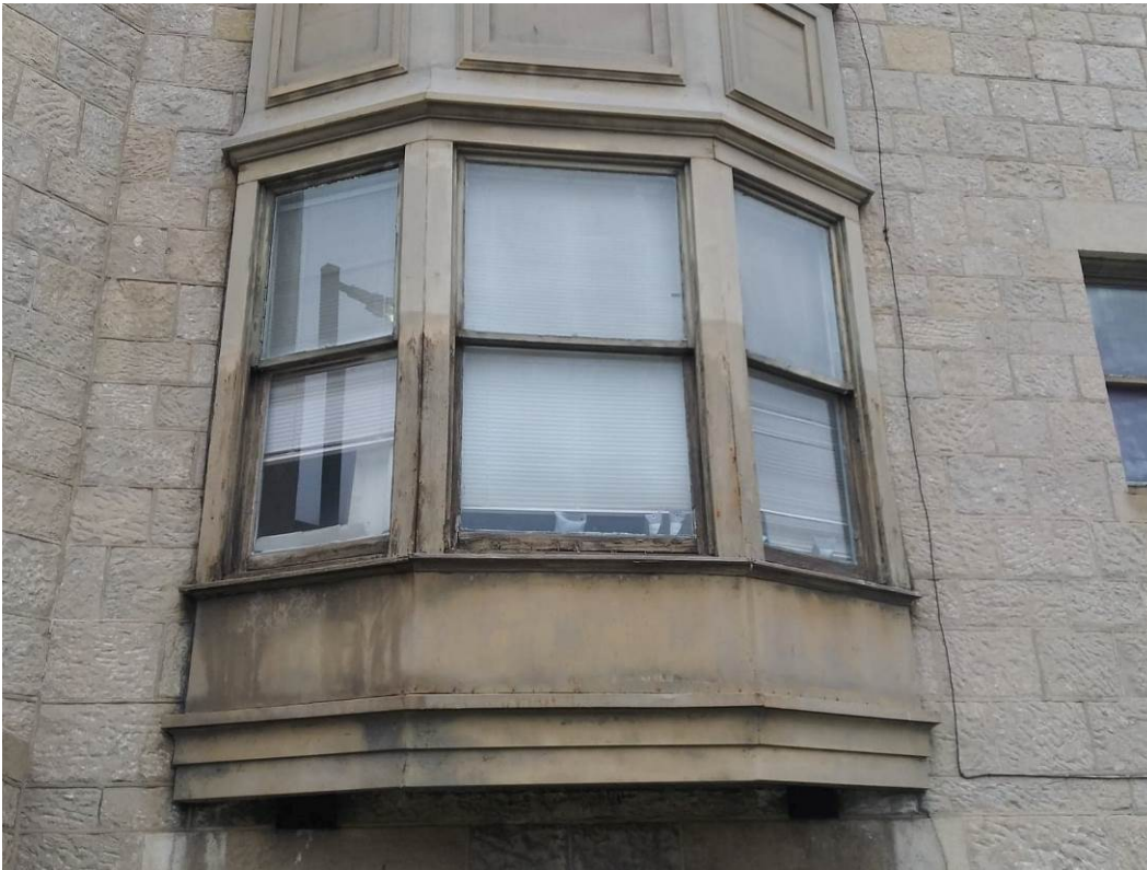
19. North bay window on West Elevation looking east at bay windows (lower).
