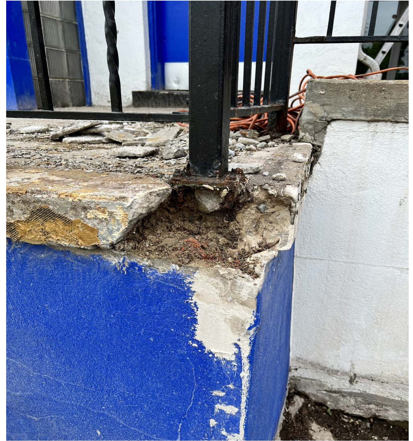
CRACKING AT EDGE OF EXISTING CONCRETE PORCH SLAB, EXPOSING CONER POST OF EXISTING GUARDRAIL
