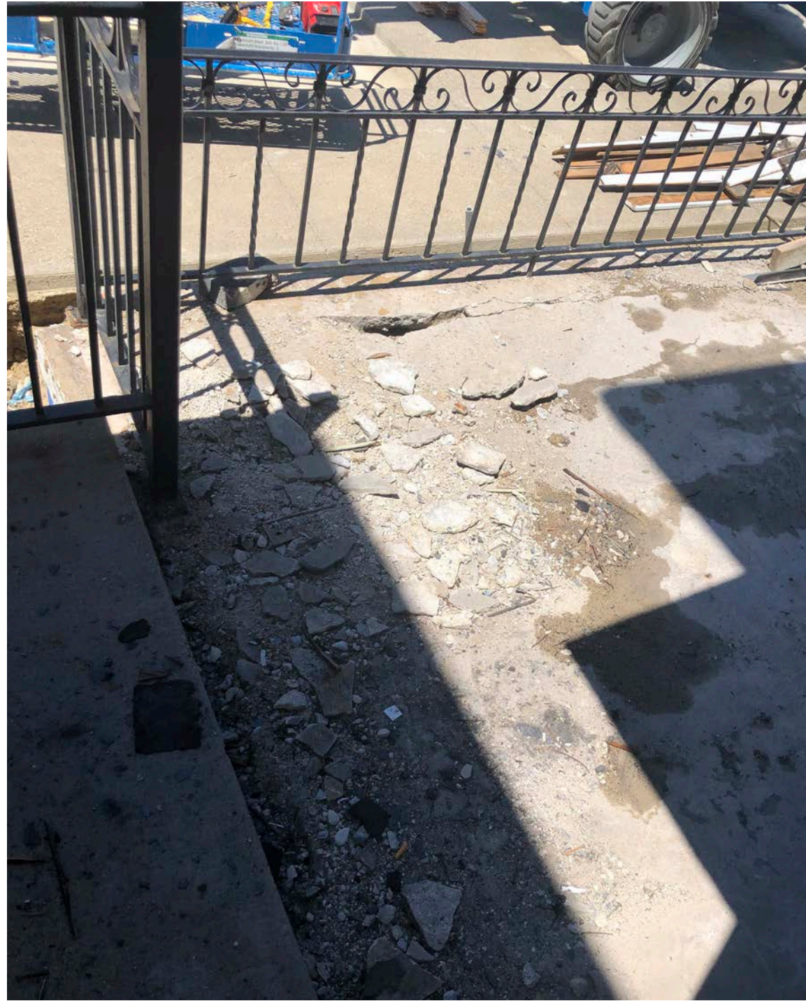
CRACKING AND HOLES AT OF TOP OF EXISTING CONCRETE PORCH SLAB
