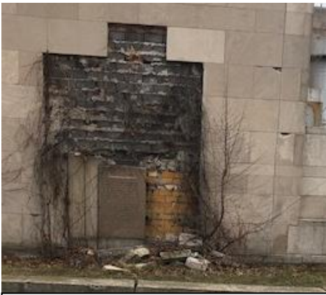
Area of wall identified as needing new limestone panels installed at existing building elevation to remain
