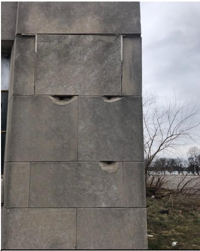
Typical area exhibiting limestone spalls, joint failure, as well as stones in need of being reset
