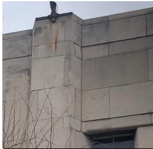
Typical area exhibiting limestone joint failure as well as stones in need of being reset
