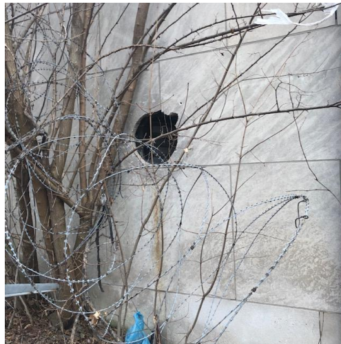
Area beyond repair, new stone will be furnished and installed to match existing
