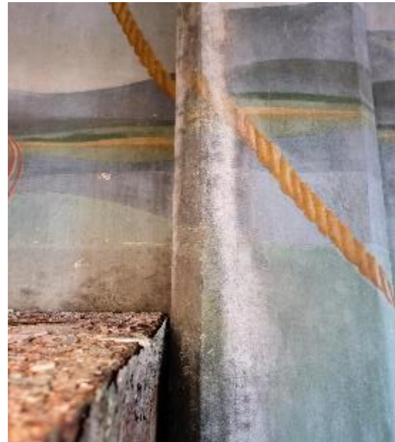
Detail of the lower right-hand portion of the mural. The water damage has caused some surface discoloration, flaking paint, and losses. There also may be some mold growth.
