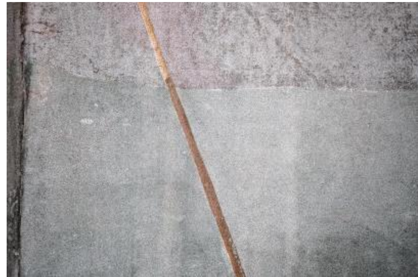
Detail of the lower right portion of the mural. There is some moderate to heavy surface discoloration.
