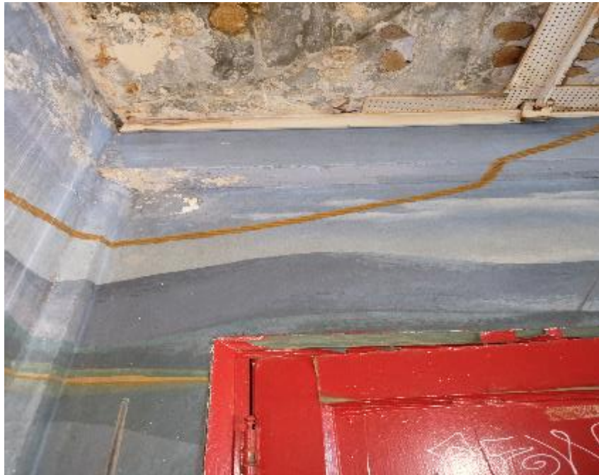
Detail of the upper left-hand portion of the mural. The water damage has caused some surface discoloration, flaking paint, and losses.
