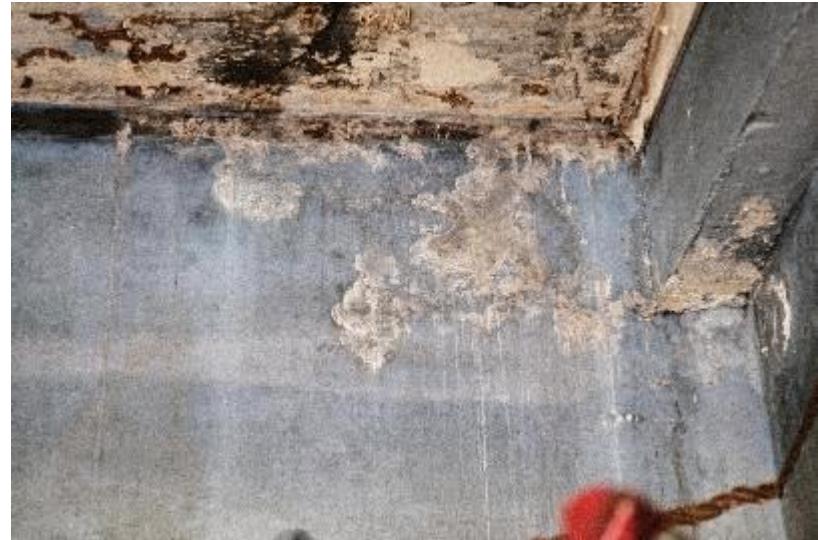
Detail of the upper right-hand corner. The water infiltration has caused heavy tide marks, efflorescence, and some mold growth.
