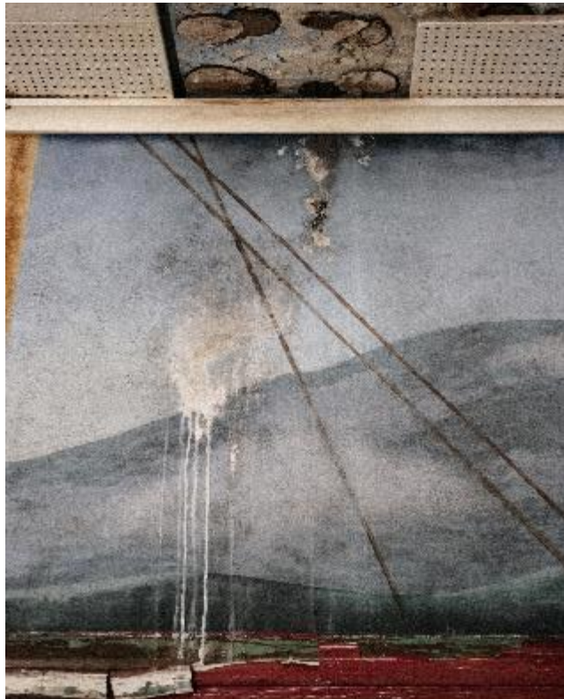
Detail of the area above the door surround. The water infiltration has caused heavy tide marks, efflorescence, and some mold growth.
