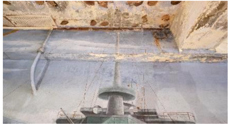
Detail of the center top portion of the mural. The water damage has caused some surface discoloration, flaking paint, and losses.
