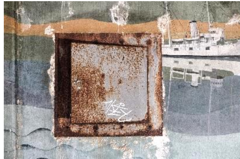
Detail of the right hand portion of the mural. There is moderate water damage and efflorescence from the moisture.
