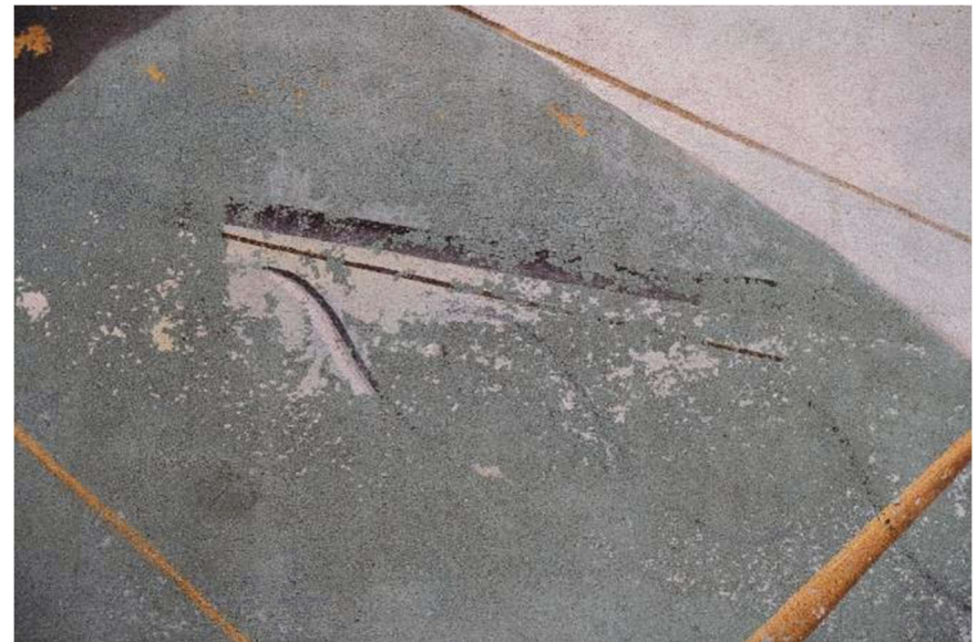
Detail of flaking paint has exposed some of Yaeger's earlier design.
