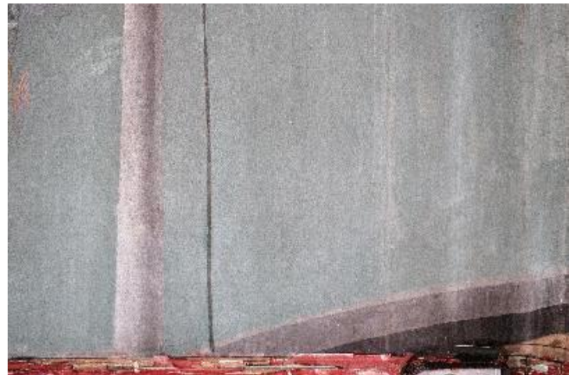
Detail of the lower right-hand portion of the mural. The water infiltration has caused some surface discoloration and active flaking paint.
