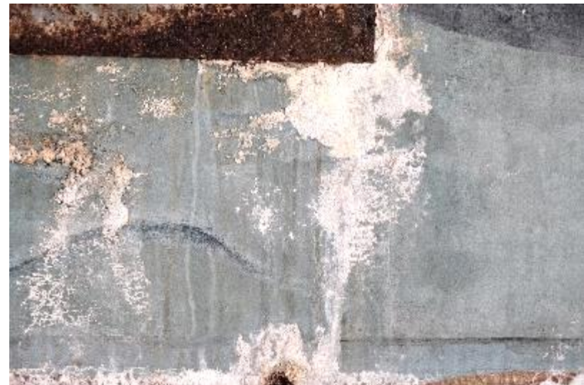
Closer detail below the metal hatch showing the extent of water damage.
