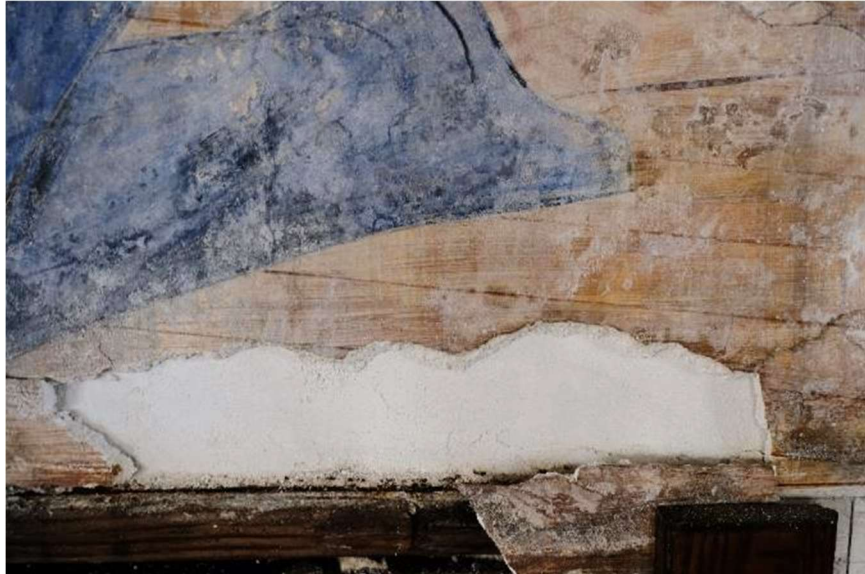
Detail showing the loss at the bottom of panel WN5.
