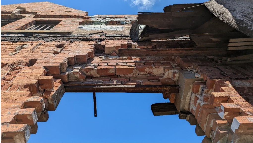
Picture 5: Missing Lintel at Opening in South Wall.
