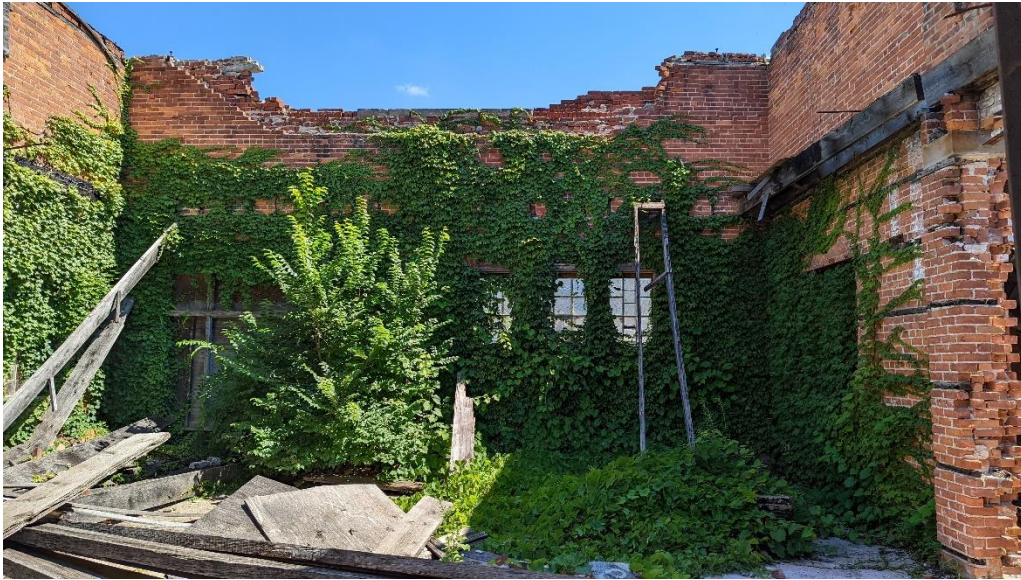
Picture 3: East Wall of Carriage House with Collapsed Gable
