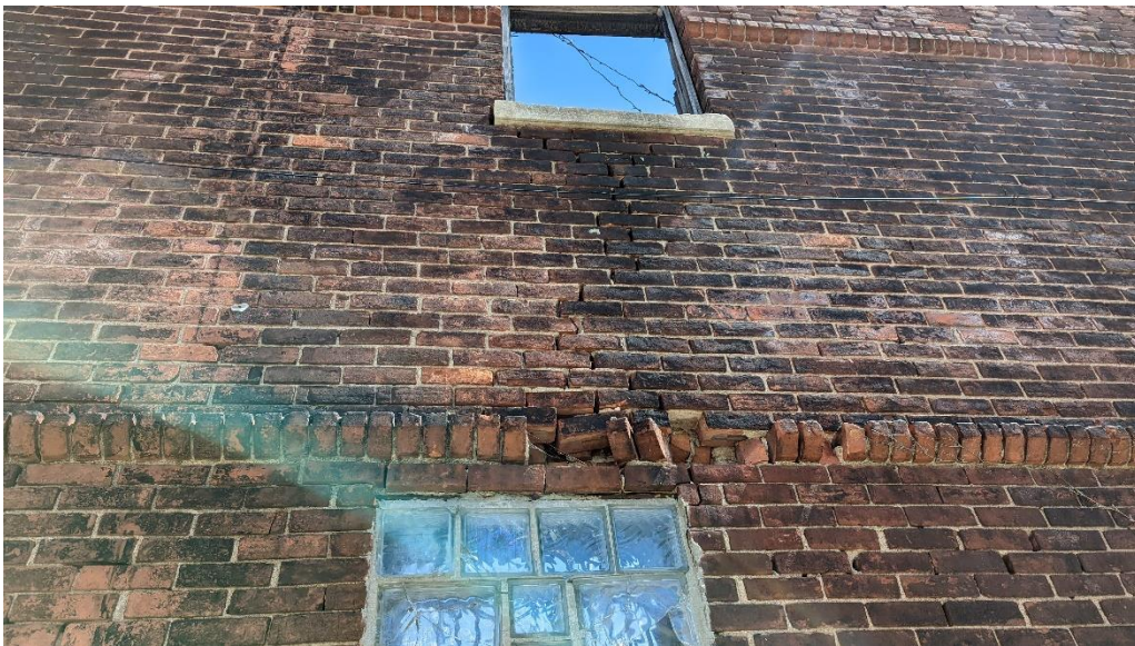
Picture 8: Crack Between Windows in West Wall
