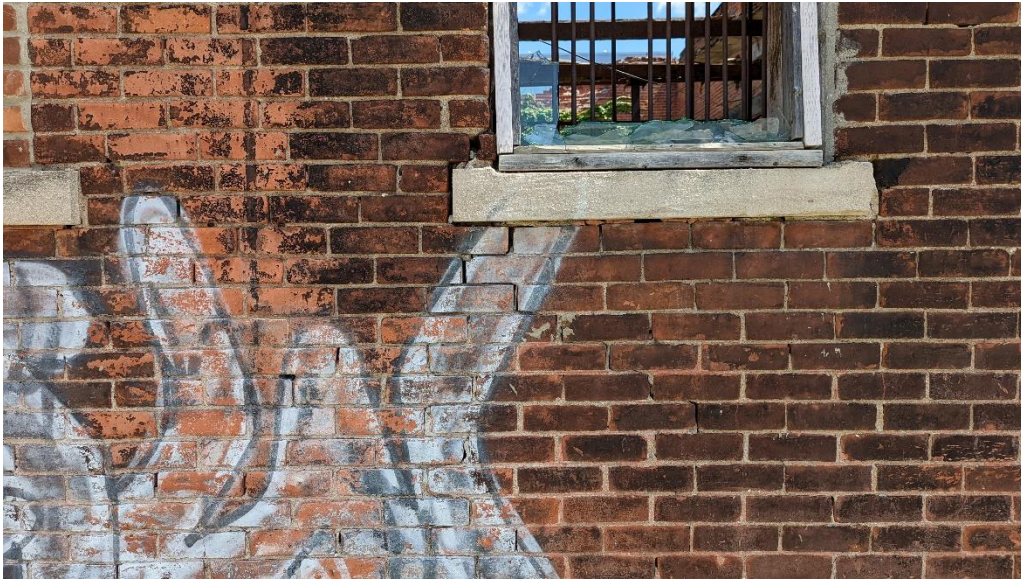
Picture 7: Crack Below Window in West Wall
