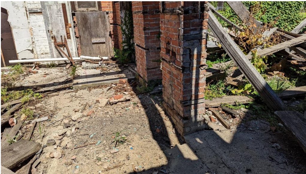
Picture 14: Loss of Soil at Foundation of the Center Wall.
