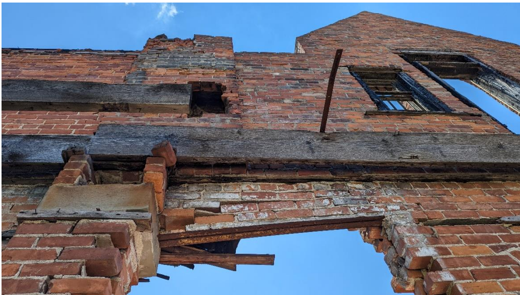
Picture 6: Missing Lintel at Opening in South Wall.
