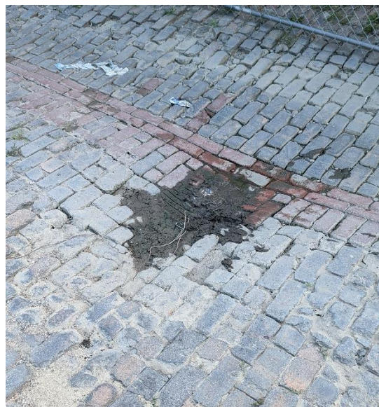
Picture 15: Sinkhole in Alley.
