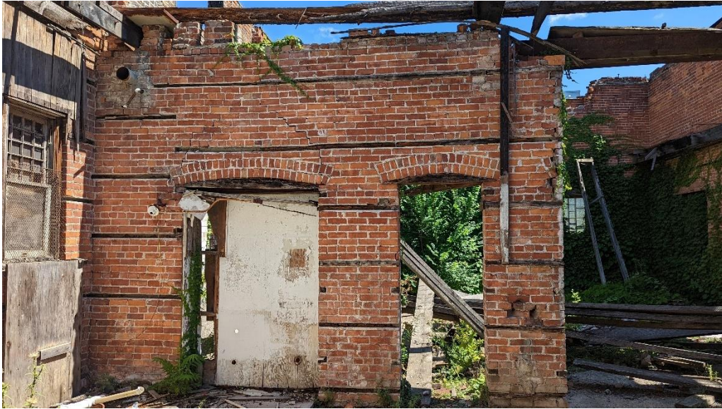
Picture 16: Wall in Center of Building Missing Lintels.
