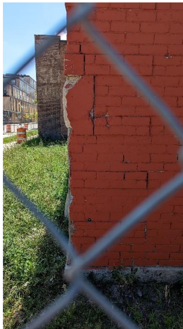
Picture 13: Crack Along Intersection of Walls at Northeast Corner.
