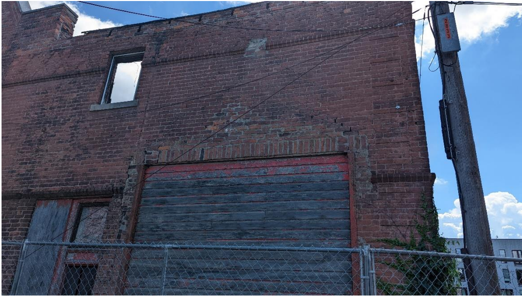
Picture 9: Crack Above Window in North Wall
