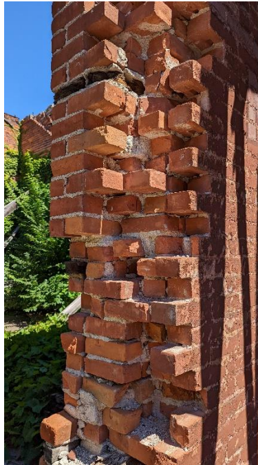
Picture 18: Loose Brick at Opening in South Wall.
