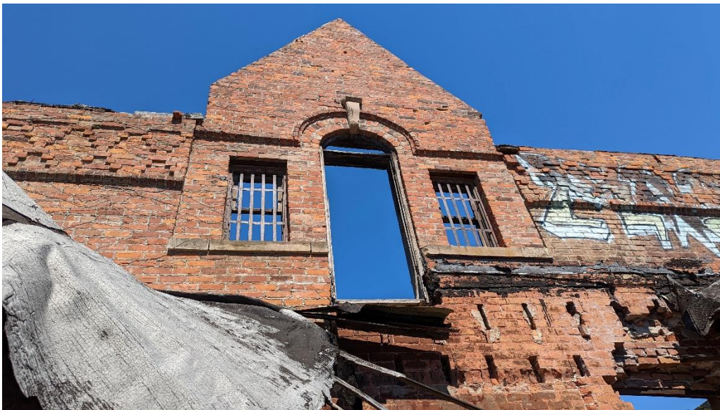
Picture 4: Leaning Gable in South Wall.
