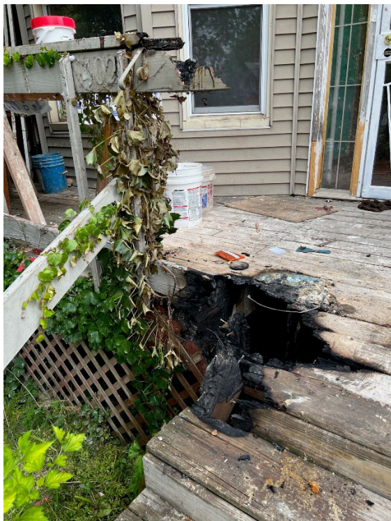
Porch after small fire
