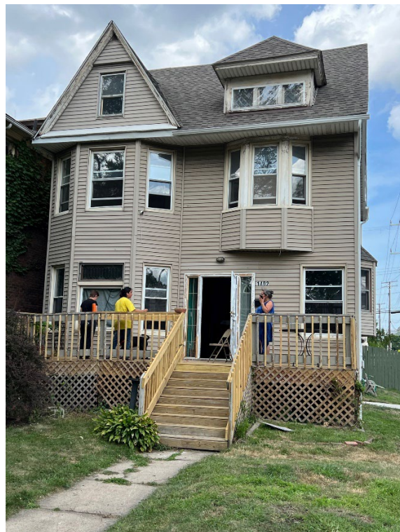
Repair porch with unpainted wood
