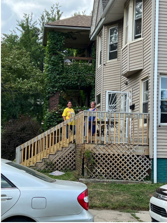
Side view porch needing painting
