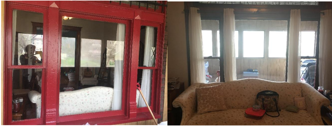
3 windows to be replaced inside covered porch on front of house (Northeast Side)
