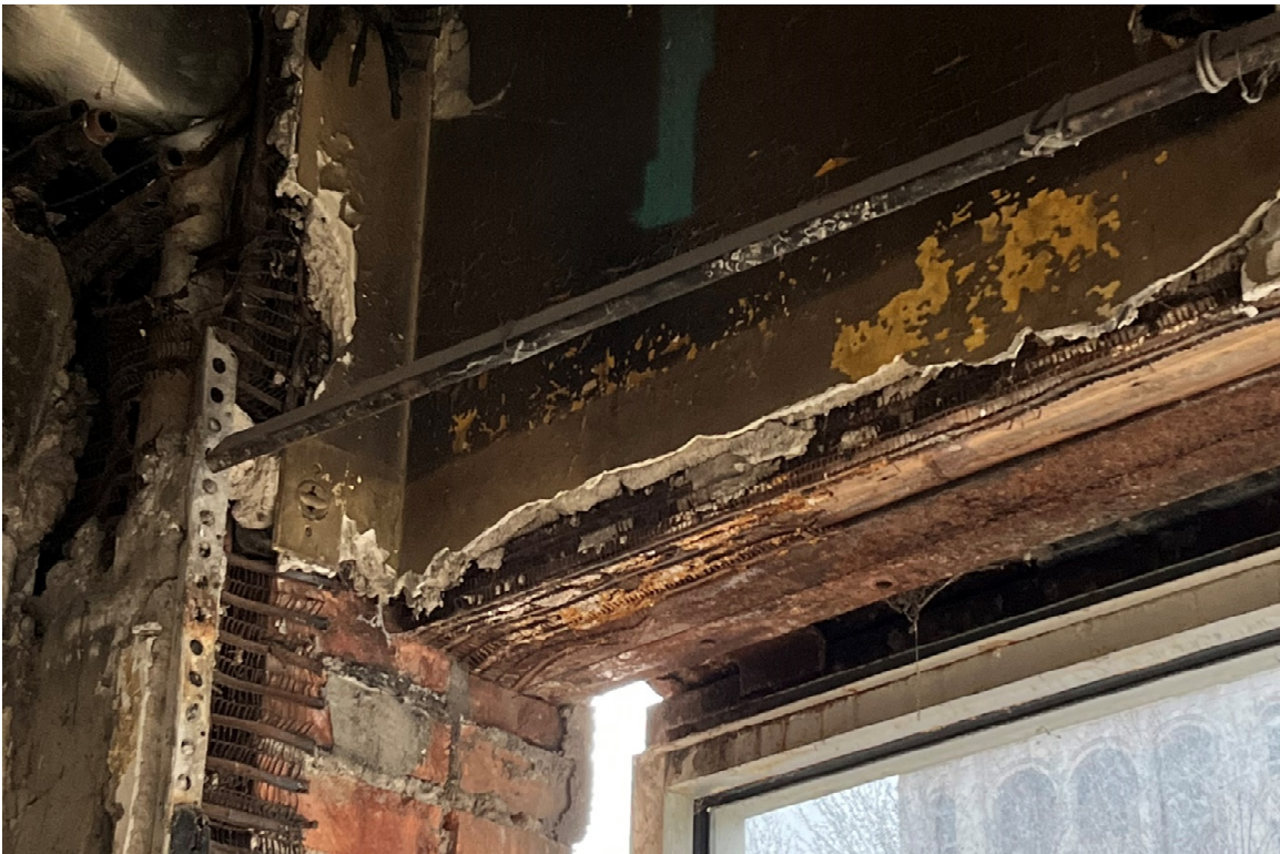
Figure #11: 1st Floor, Storefront Header. 04/01/22.
