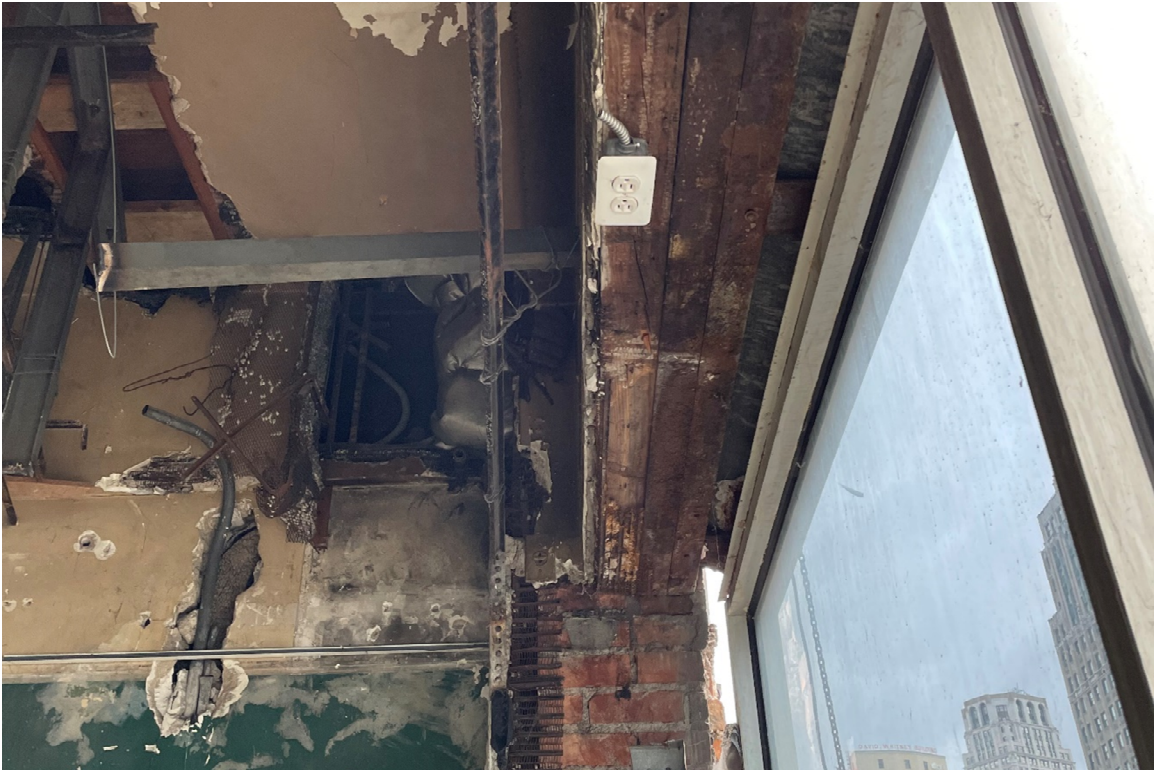
Figure #10: 1st Floor, Storefront Header. 04/01/22.
