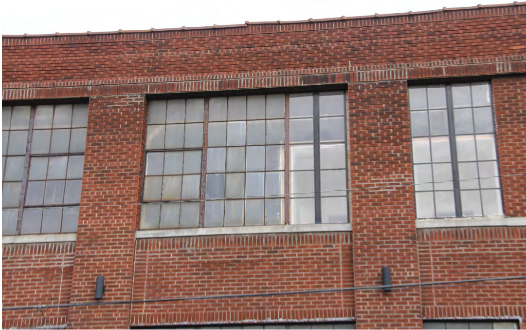
Exterior View of Original Steel Windows Next to Incorrect Replication
