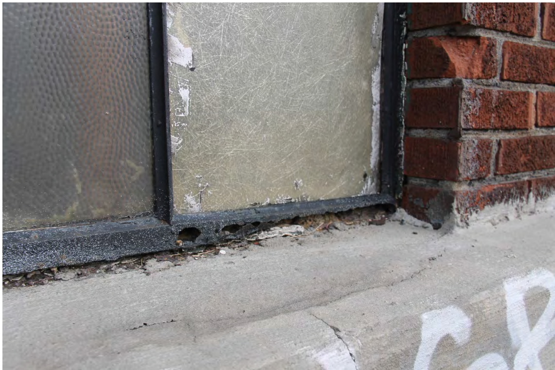
Typical Bottom Rail Condition, Exterior View
