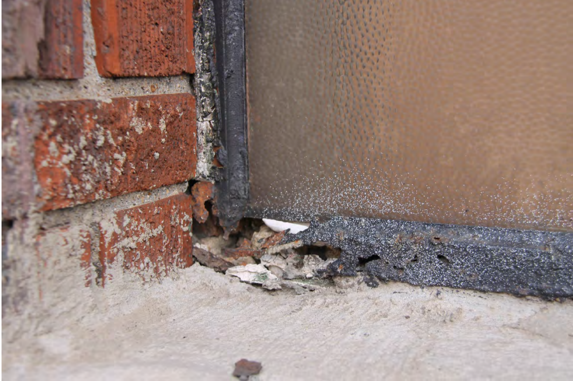
Typical Bottom Rail Condition, Exterior View
