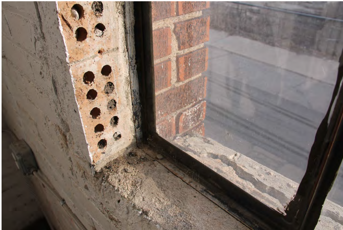
Interior View of Replica Steel Window, Shows Altered Masonry Opening Changing Window Size
