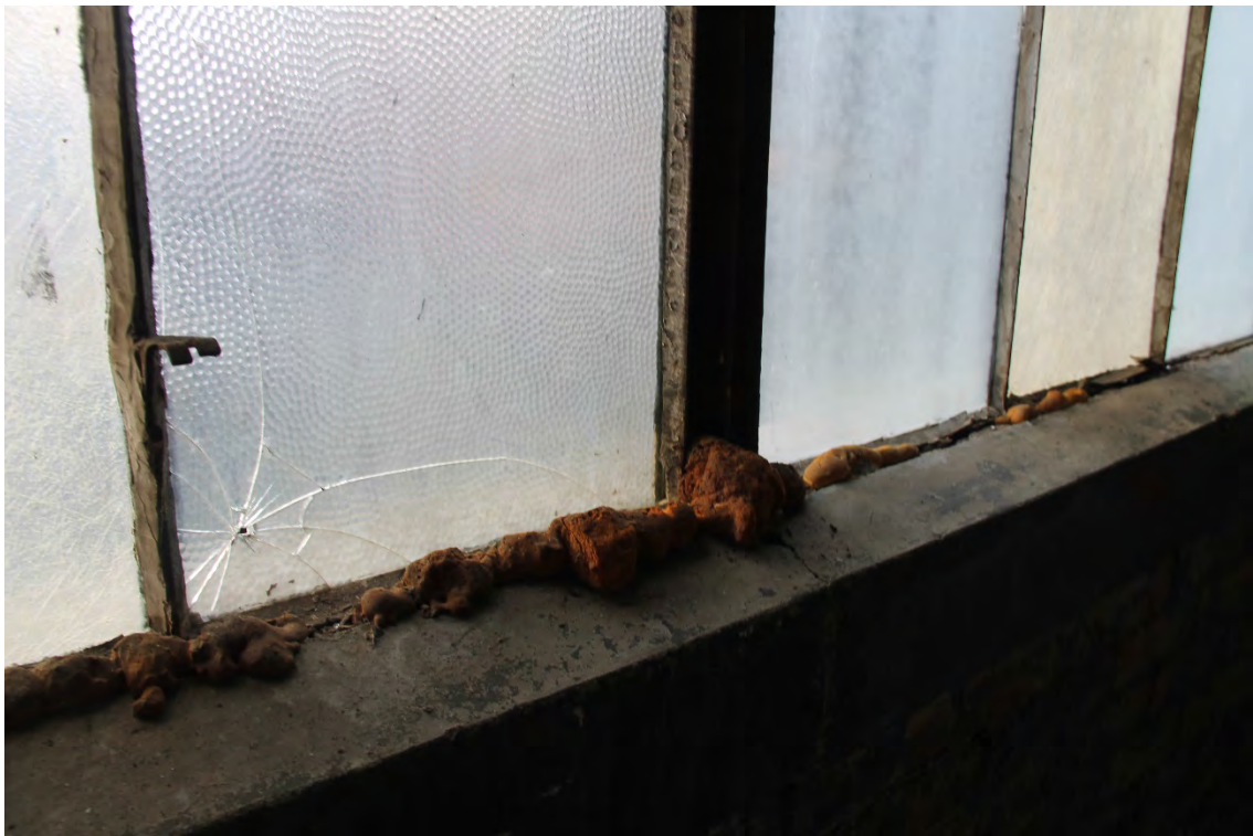
Typical Mullion and Bottom Rail Condition of Existing Steel Window, Interior View
