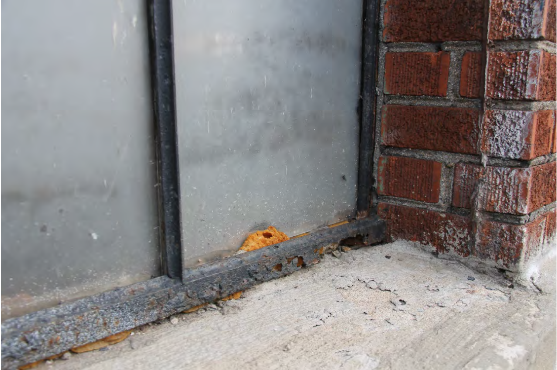
Typical Bottom Rail Condition, Exterior View
