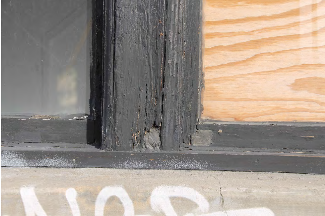
Exterior View of Failed Mullion Assembly and Bottom Sash
