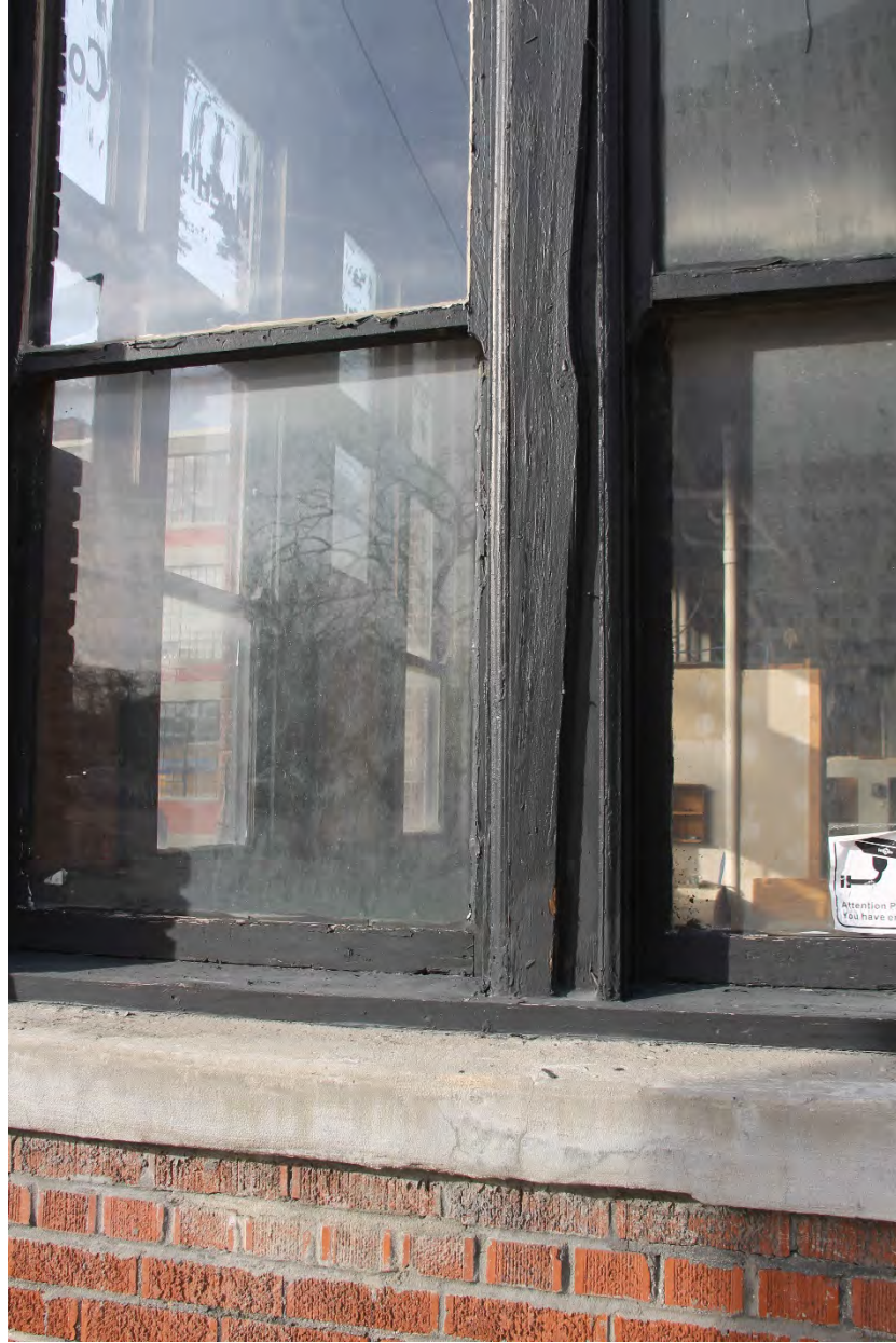
Exterior View of Broken Mullion Cover Allowing Water Penetration
