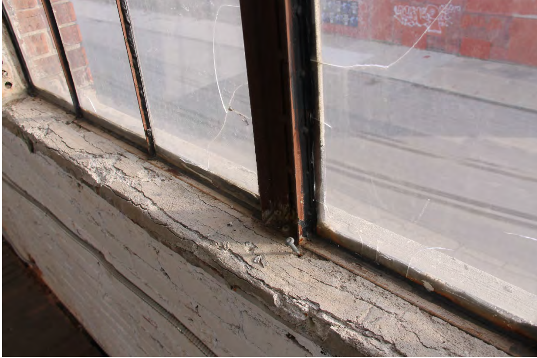
Interior View of Replica Steel Windows, Mullion, and Glazing with Incorrect Glazing Install
