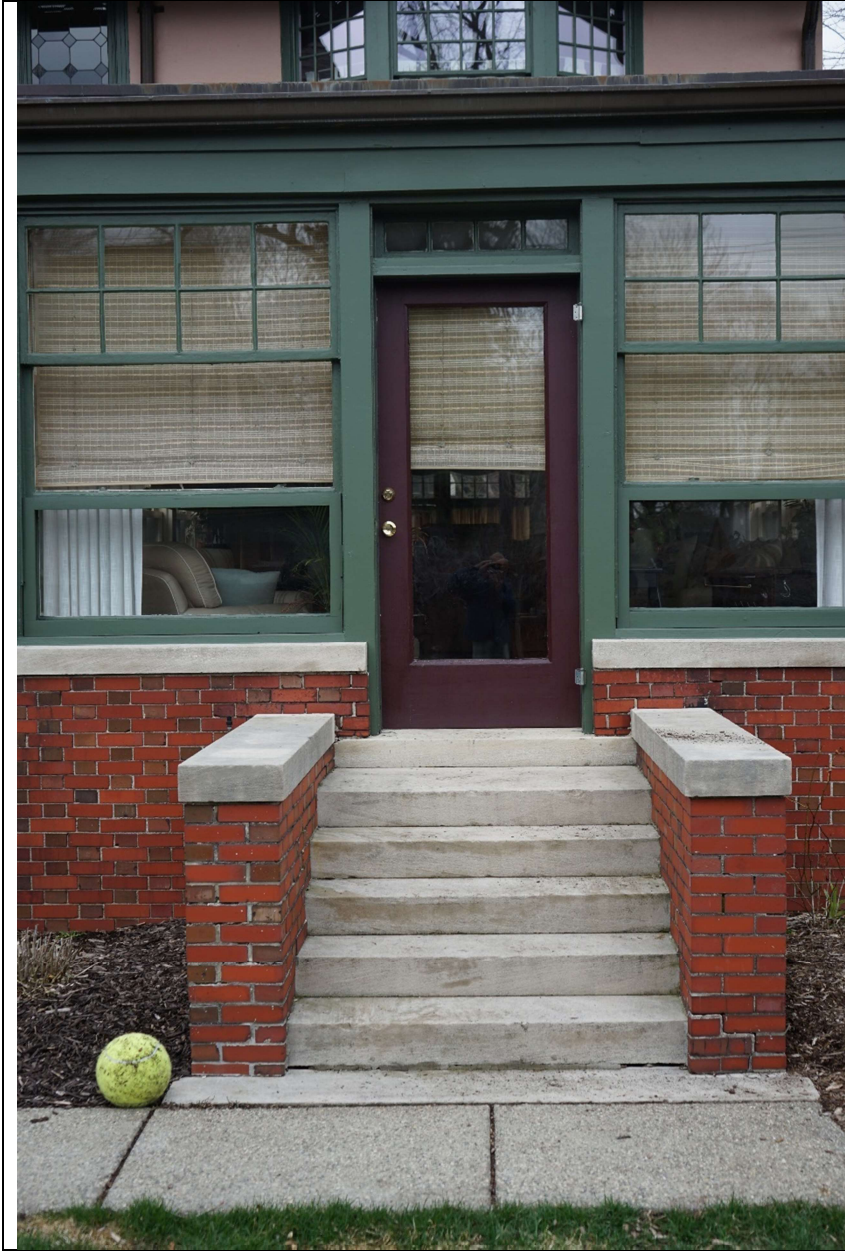
Photo 4 Original Stair case to sunroom door, Stairs are limestone and brick wing walls include limestone caps
