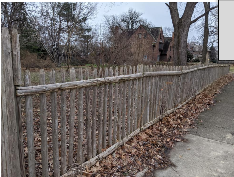
Deteriorating fence along Burns
