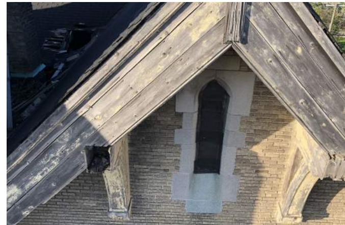
FIGURE A4.24 WEATHER AND FADED FASCIA BOARDS; DECAYED HOLLOWED WOODEN SUPPORT BRACKET
