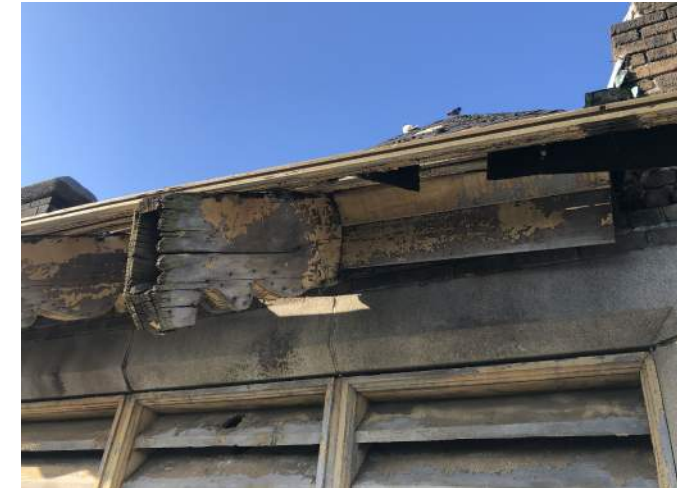
FIGURE A3.8 ROTTED DECORATIVE WOOD RAFTER TAIL AND DETACHING FRIEZE BOARD TRIM
