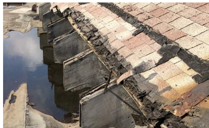
FIGURE A2.13 DECORATIVE WOOD EAVE SHOW SIGNS OF DECAY AND ROT; SIGNIFICANT DETERIORATION OF THE ROOF PERIMETER EDGE; WITH POOLS OF WATER GATHERING UNDER THE EAVES
