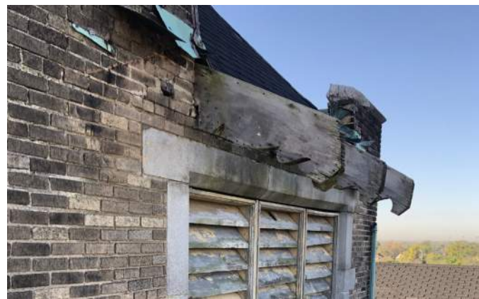
FIGURE A3.6 DIFFERENTIAL BRICK MOVEMENT UNDER EAVES; REMNANTS OF THE ORIGINAL STEPPED COPPER FLASHING; (NORTH ELEVATION)
