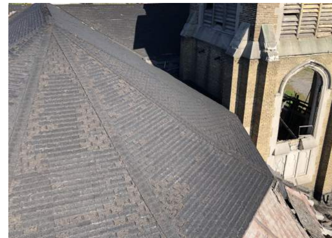
FIGURE A2.10 UPPER TIER OF HEPTAGON ROOF; WORN, MISSING CURLED, DISCOLORED, AND FRAYED ASPHALT SHINGLES
