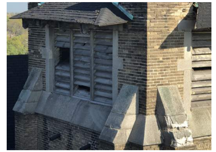
FIGURE A3.12 SOUTH WEST ELEVATION OF BELL TOWER; CRUMBLING STONE AT THE COLUMN CAP; BRICK MOVEMENT DIRECTLY UNDER THE ROOF
