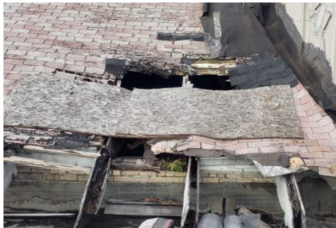
FIGURE A2.7 COMPLETE DETERIORATION AND DECAY OF THE DECORATIVE WOOD EAVES AND DECORATIVE RAFTER TAILS; THE LEVEL OF DETERIORATION MAY REQUIRE LOCALIZED REPAIRS TO ADJACENT ELEMENTS SUCH AS THE BRICK WALL BELOW
