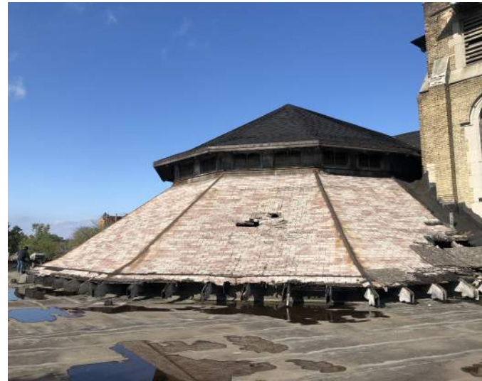
FIGURE A2.1 OVERVIEW OF THE TWO TIERED HEPTAGON ROOF; ROOF DECAY AND WATER INFILTRATION, WORN AND MISSING ASPHALT TILES, WEATHERED AND ROTTED DECORATIVE EAVE OUTRIGGERS/RAFTER TAILS.
