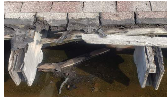
FIGURE A2.8 SIGNIFICANT DETERIORATION AT THE PERIMETER (TERMINATION OF DECORATIVE EAVES); EXTENSIVE WOOD ROT OF THE DECORATIVE EAVE OUTRIGGERS/RAFTER TAILS; PONDING WATER BELOW
