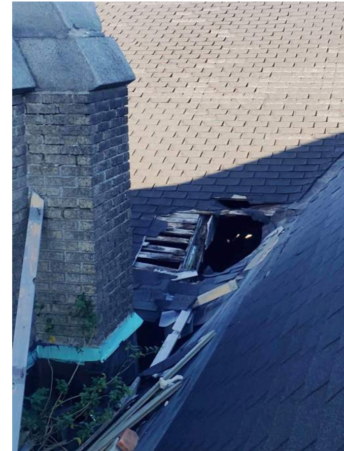
FIGURE A4.17 LARGE HOLE IN THE ROOF; DETERIORATED SHINGLES, WOOD DECKING AT THE ROOF VALLEY; FALLEN WOOD DECKING FROM THE BELL TOWER ROOF ABOVE
