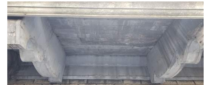
FIGURE A4.3 DECORATIVE WOOD EAVE IN FAIR CONDITION; (NORTH ELEVATION)
