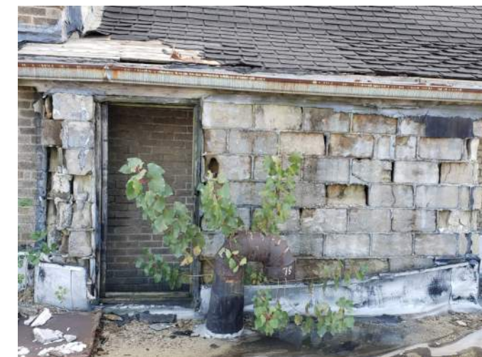
FIGURE A4.23 EXTENSIVE EXTERIOR MASONRY DETERIORATION AT ROOFTOP STAIR ENTRY/EXIT; MISSING AND DETERIORATED MORTAR JOINTS; DETACHED ROOFTOP STAIR ENTRY DOOR; DAMAGED DOOR FRAMING. DETACHED FLASHING AT THE UPTURN OF THE NORTH MEMBRANE ROOFING
