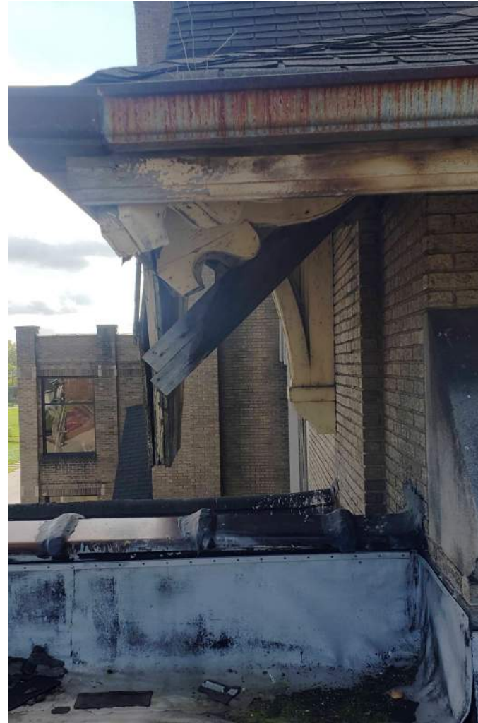
FIGURE A4.12 WEATHERED, FADED EAVES; RUSTED GUTTER (EAST ELEVATION)
