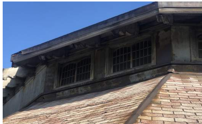
FIGURE A2.11 THE UPPER TIER OF THE POLYGONAL ROOF; VISIBLE RUST ON THE METAL WINDOW FRAMING AND ROOF HIPs; METAL FLASHING IS CORRODING AND DETACHING FROM THE FASCIA BOARD AND HEAD OF LOWER ROOF
