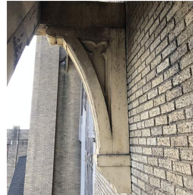
FIGURE A4.15 UNDERSIDE OF THE EAVES; PAINTED WOODEN BRACKET EAVE SUPPORT; (EACH BRACKET SHOULD BE INDIVIDUALLY EVALUATED)
