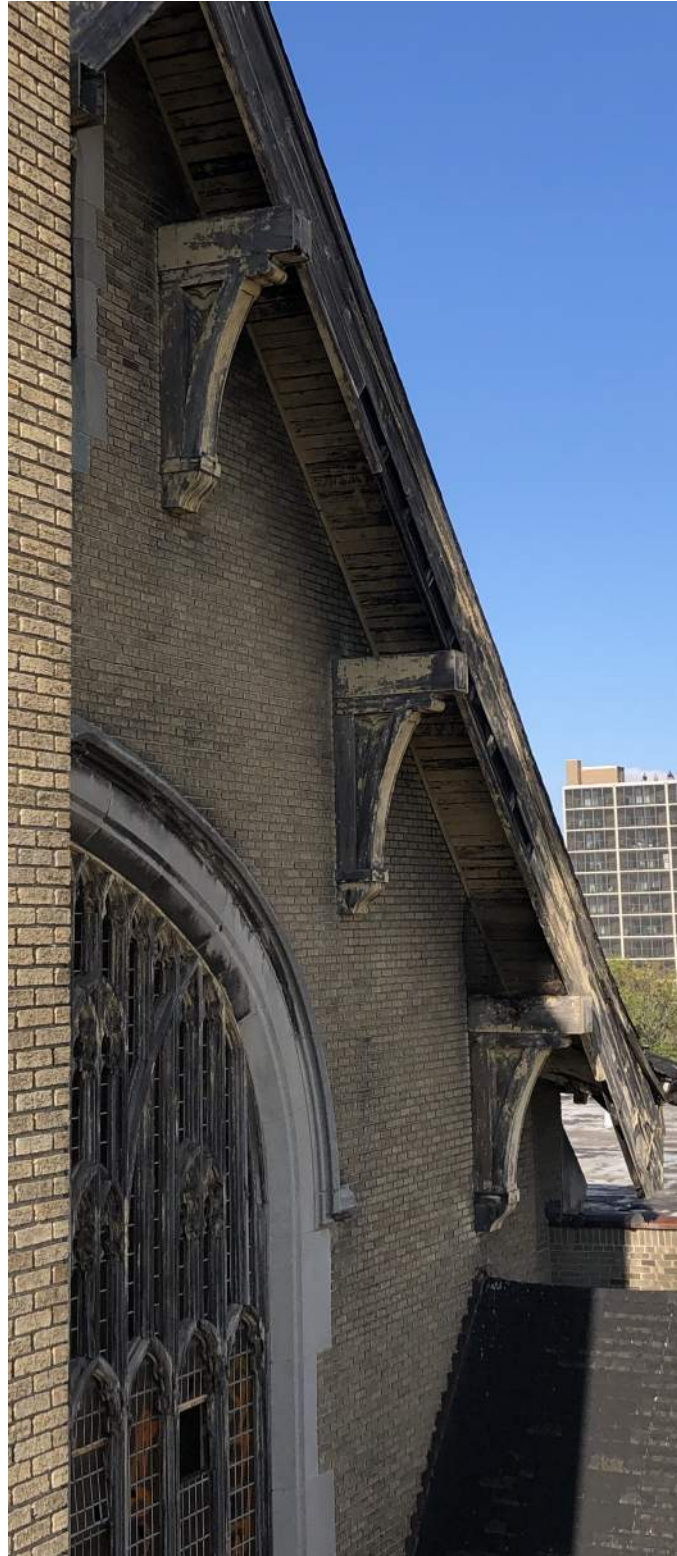
FIGURE 4.22 WEATHER AND FADED FASCIA BOARDS, FADED WOOD DECKING AT THE UNDERSIDE OF THE EAVES ON THE EAST ELEVATION AT THE MAIN ENTRANCE
