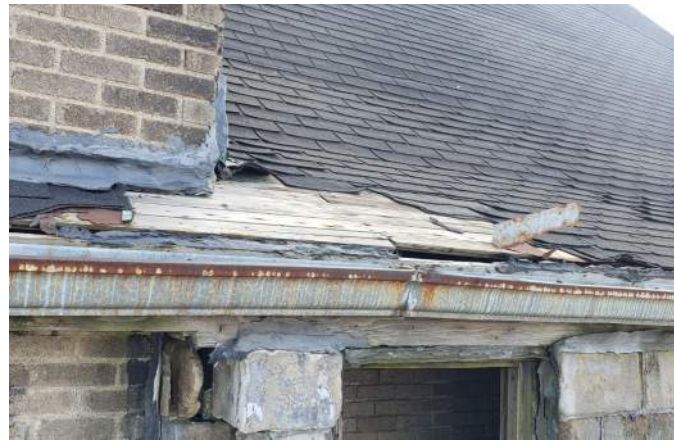
FIGURE A4.9 WEATHERED FASCIA BOARD; DECAYED WOOD DECKING; CURLLED, FRAYED AND MISSING ASPHALT SHINGLES ABOVE ROOFTOP STAIR ENTRY.
