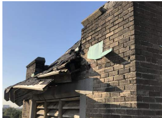
FIGURE A3.4 DECORATIVE WOOD OVERHANGS COLLAPSING AND OPEN AT ENDS TO INTERIOR; BRICK MASONRY SHOWS SIGNS OF DIFFERENTIAL MOVEMENT; REMAINING STEPPED COPPER FLASHING (EAST ELEVATION)
