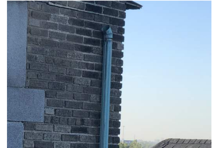
FIGURE A3.11 DETACHED COPPER DOWNSPOUT AND MISSING ASSOCIATED COPPER GUTTER
