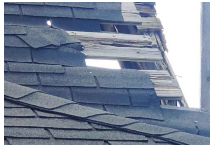
FIGURE 4.1 DETERIORATED WOOD DECKING, MISSING/FALLEN SHINGLES AT THE EAVE (WEST ELEVATION)
