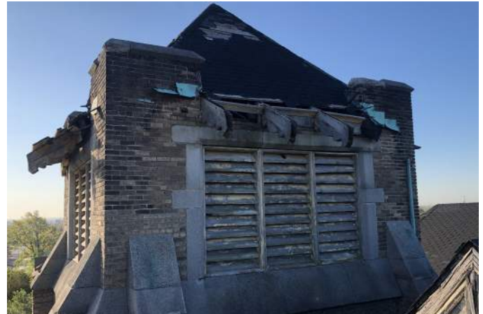
FIGURE A3.10 OVERVIEW OF THE BELL TOWER'S ROOF AND DECKING; THE DECKING ON TOP OF THE DECORATIVE EAVE HAS COMPLETELY DECAYED AND DETACHED FROM THE ROOF ASSEMBLY (NORTH ELEVATION)
