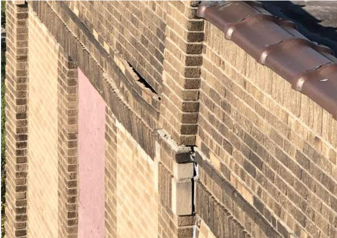
FIGURE A1.22 "ROLLING" BRICK DISPLACEMENT AT THE EXTERIOR PARAPET; BUCKLING AT PIER COLUMN
