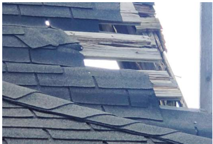
FIGURE 4.1 DETERIORATED WOOD DECKING, MISSING/FALLEN SHINGLES AT THE EAVE (WEST ELEVATION)
