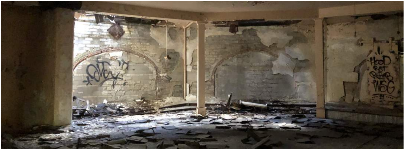
FIGURE INT.1.6 FAILED FINISHES AND DEBRIS IN CLASSROOMS OVER SANCTUARY; OPENINGS THRU ROOFS TO DAYLIGHT ABOVE
