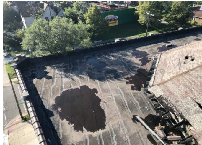
FIGURE A1.3 EAGLE VIEW OF THE SOUTH FLAT ROOF; VARIOUS AREAS OF STANDING WATER
