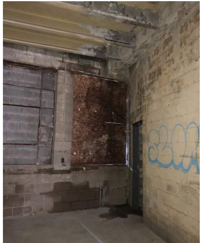
FIGURE INT 1.11 BOARDED UP FORMER WINDOW OPENINGS
