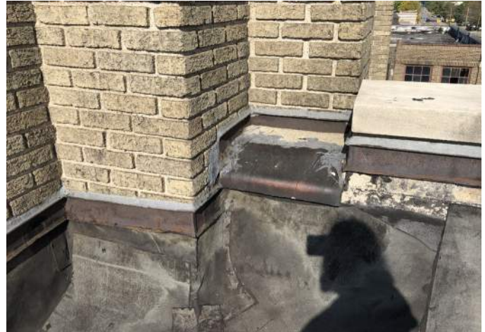
FIGURE A1.12 RUSTED FLASHING; WEATHERED SEALANTS, FLASHING MISSING AT THE UNDERSIDE OF THE COLUMN CAP
