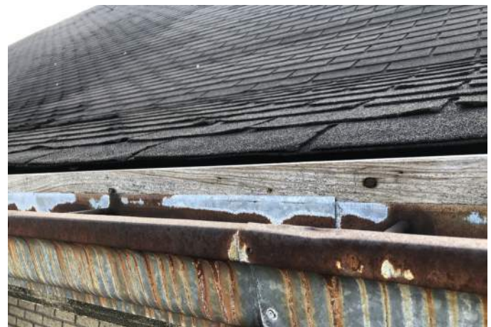
FIGURE A4.5 RUSTED GUTTER, CURLLED AND FRAYED ASPHALT SHINGLES
