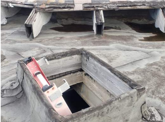
FIGURE A1.5 EXISTING ROOF HATCH WITH DETACHED ROOF HATCH CAP
