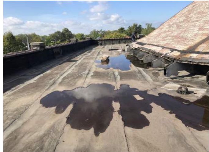
FIGURE A1.1 OVERVIEW LOOKING WEST AT VARIOUS POOLS OF STANDING WATER; FRAYED WARPED ROOFING MEMBRANE SEAMS; NO INDICATION OF ROOF INSULATION OR TAPERING
