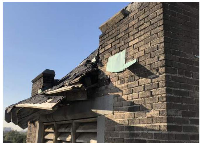
FIGURE A3.4 DECORATIVE WOOD OVERHANGS COLLAPSING AND OPEN AT ENDS TO INTERIOR; BRICK MASONRY SHOWS SIGNS OF DIFFERENTIAL MOVEMENT; REMAINING STEPPED COPPER FLASHING (EAST ELEVATION)
