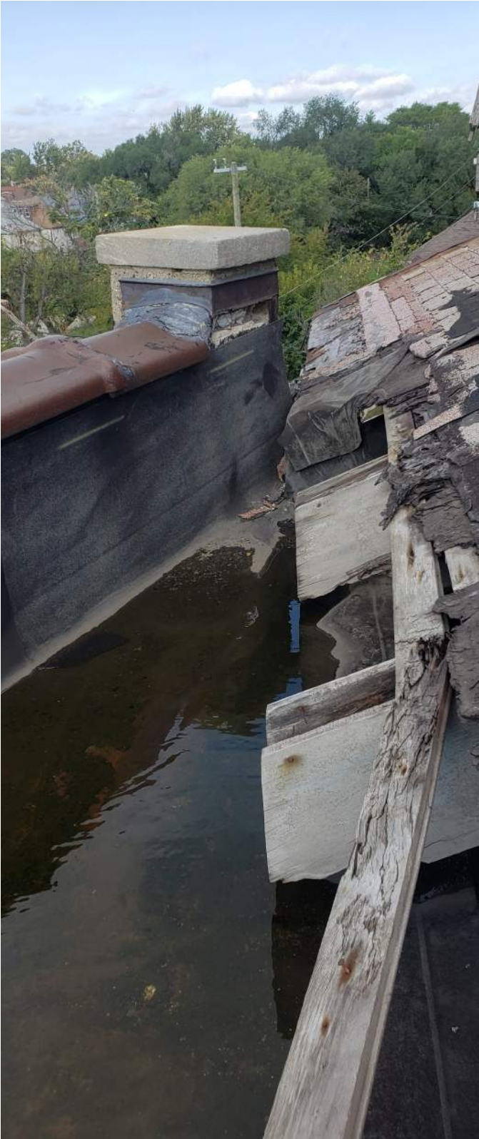
FIGURE A1.15 DETERIORATING CORNER COLUMN, UNFLASHSED MASONRY AT PIER COLUMN; 3" OR MORE PONDING WATER AT SOUTHWEST CORNER
