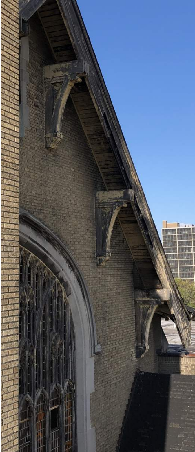
FIGURE 4.22 WEATHER AND FADED FASCIA BOARDS, FADED WOOD DECKING AT THE UNDERSIDE OF THE EAVES ON THE EAST ELEVATION AT THE MAIN ENTRANCE
