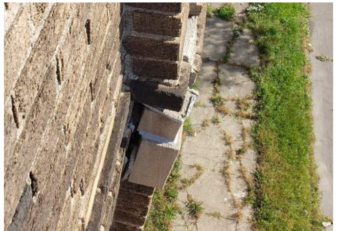
FIGURE A1.16 "ROLLING" BRICK DISPLACEMENT AT THE EXTERIOR PARAPET PIER COLUMN
