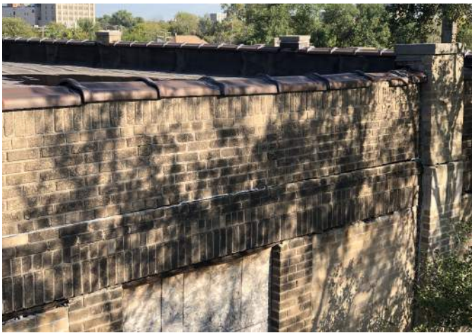
FIGURE A1.23 CORRODED AND EXPANDING LINTELS; "ROLLING" BRICK DISPLACEMENT AT THE EXTERIOR PARAPET
