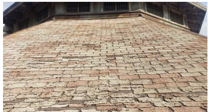
FIGURE A2.2 SURFACE DEPRESSIONS ALONG THE ROOF; CURLED, DISCOLORED AND FRAYED ASPHALT SHINGLES; RUSTED METAL FLASHING UNDER THE UPPER WINDOWS
