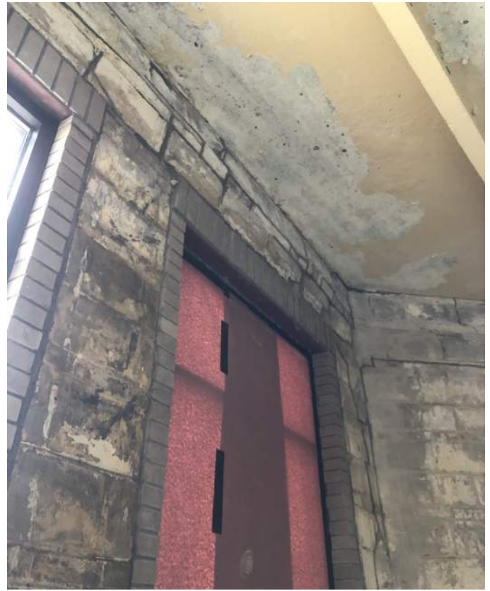
FIGURE INT 1.10 BUCKLING AND CRACKED MASONRY EXTERIOR WALLS
