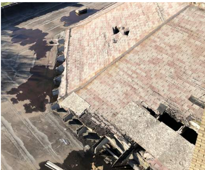
FIGURE A2.12 OVERVIEW OF THE HEPTAGON ROOF ABOVE, SHOWS THE EXTENT OF THE ROOF DETERIORATION WITH VARIOUS HOLES ALONG THE SURFACE
