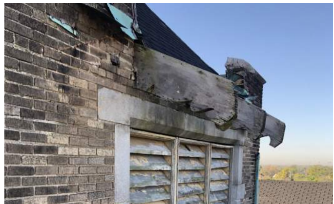
FIGURE A3.6 DIFFERENTIAL BRICK MOVEMENT UNDER EAVES; REMNANTS OF THE ORIGINAL STEPPED COPPER FLASHING; (NORTH ELEVATION)
