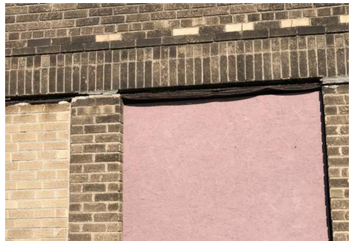
FIGURE A1.21 CORRODED AND EXPANDING STEEL LINTEL ABOVE THE WINDOWS ON THE THIRD FLOOR
