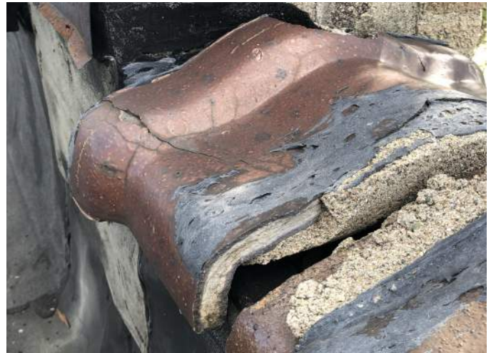
FIGURE A1.9 CRACKED AND DETACHED CLAY TILES AT THE PARAPET
