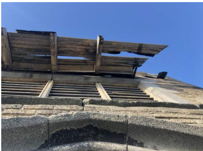
FIGURE A3.9 UNDERSIDE OF THE PAINTED DECORATIVE OVERHANGS; WEATHERED DETERIORATED WOOD DECKING (EAST ELEVATION)
