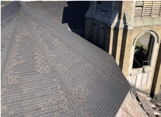
FIGURE A2.10 UPPER TIER OF HEPTAGON ROOF; WORN, MISSING CURLED, DISCOLORED, AND FRAYED ASPHALT SHINGLES
