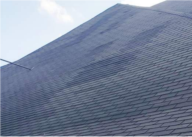
FIGURE A4.6 OVERVIEW OF NORTHERN ROOF; CURLLED, DISCOLORED, AND FRAYED ASPHALT SHINGLES; SHOW SIGNS OF DEPRESSIONS AND UNEVEN SURFACES ALONG THE ROOF
