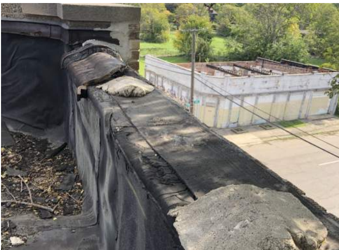
FIGURE A1.8 MISSING AND DAMAGED PARAPET CLAY TILES (SOUTHEAST CORNER)
