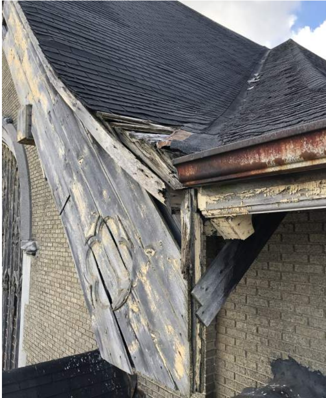
FIGURE 4.13 DECORATIVE FASCIA BOARDS ARE WEATHERED AND FADED; THEY ARE DETACHING FROM THE SUBSTRUCTURE. WOOD DECKING AT VALLEY TERMINATION IS EXPOSED, DECAYED WITH MISSING SHINGLES
