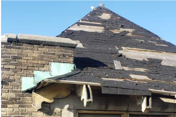
FIGURE A3.7 HIP ROOF IS IN VERY POOR CONDITION; WEATHERED AND DECAYED WOOD DECKING, MISSING/FALLEN SHINGLES AND EXPOSED DECKING AND ORIGINAL STEPPED COPPER FLASHING (EAST ELEVATION)
