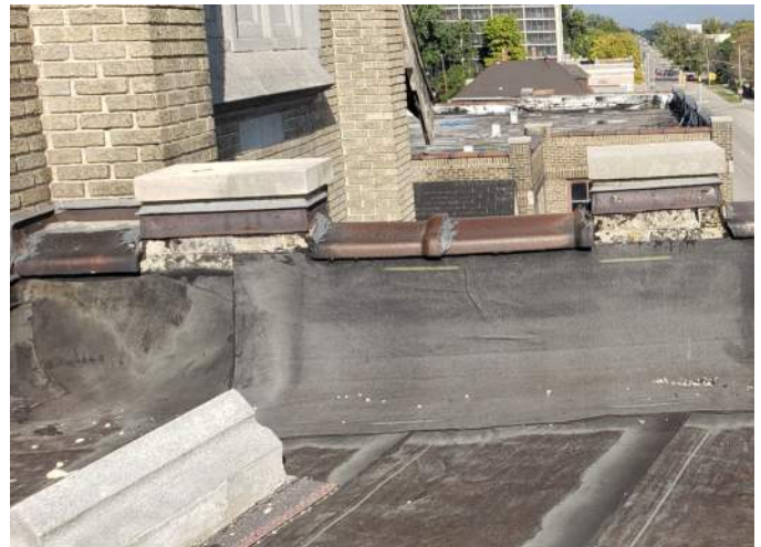
FIGURE A1.11 FLASHING MISSING UNDER COLUMN CAP
