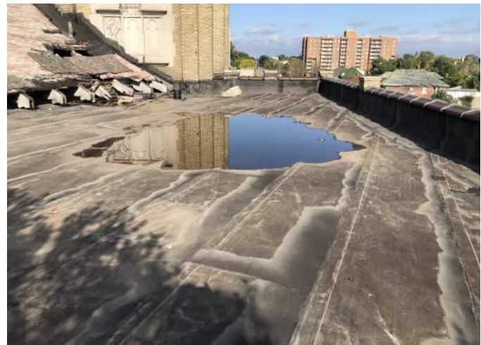
FIGURE A1.2 OVERVIEW LOOKING NORTH AT THE FLAT ROOF WITH STANDING WATER; FRAYED RUBBER ROOF SEAMS; PARAPET FLASHING
