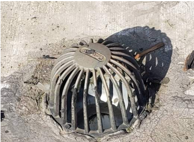
FIGURE A1.6 EXISTING ROOF DRAIN CAP BODY
