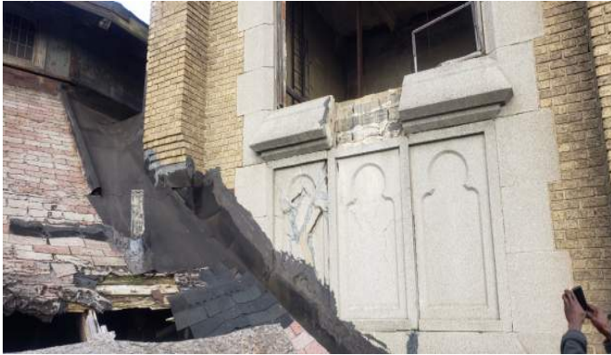
FIGURE A2.6 FAILURE OF THE FLASHING AT THE INTERSECTION WHERE THE POLYGONAL ROOF INTERSECTS WITH THE BELL TOWER; STAINING OF THE DECORATIVE STONE BY FLASHING SEALANT
