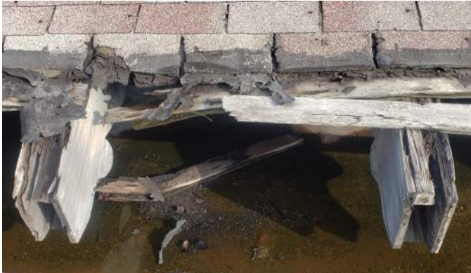
FIGURE A2.8 SIGNIFICANT DETERIORATION AT THE PERIMETER (TERMINATION OF DECORATIVE EAVES); EXTENSIVE WOOD ROT OF THE DECORATIVE EAVE OUTRIGGERS/RAFTER TAILS; PONDING WATER BELOW
