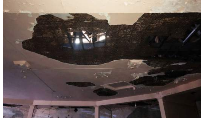
FIGURE A2.14 DETERIORATING INTERIOR PLASTER BELOW THE HEPTAGONAL ROOF STRUCTURE; SUN LIGHT IS VISIBLE THROUGH THE HOLE IN THE ROOF ABOVE
