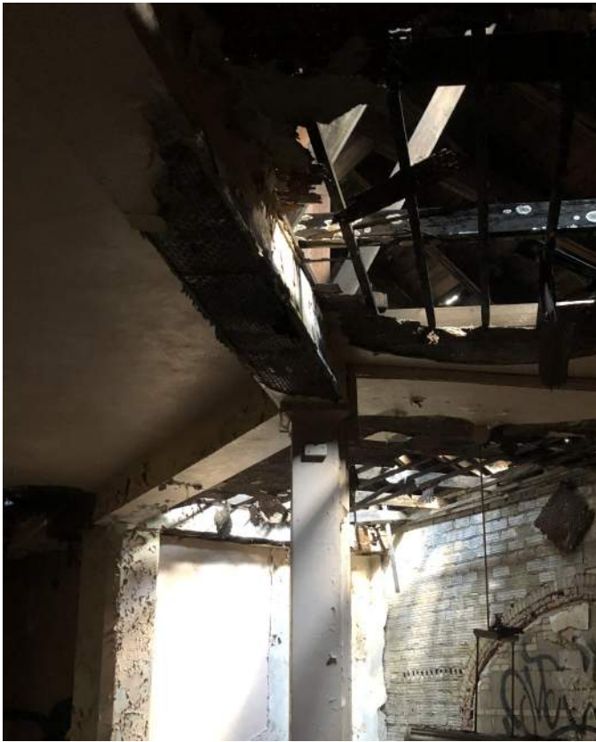
FIGURE INT 1.9 FAILED FINISHES AND DEBRIS IN CLASSROOMS OVER SANCTUARY; OPENINGS THRU ROOFS EXPOSING INTERIOR TO ELEMENTS
