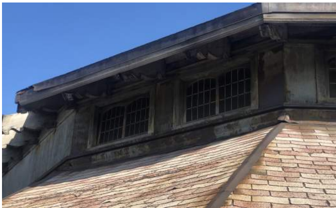
FIGURE A2.11 THE UPPER TIER OF THE POLYGONAL ROOF; VISIBLE RUST ON THE METAL WINDOW FRAMING AND ROOF HIPS; METAL FLASHING IS CORRODING AND DETACHING FROM THE FASCIA BOARD AND HEAD OF LOWER ROOF
