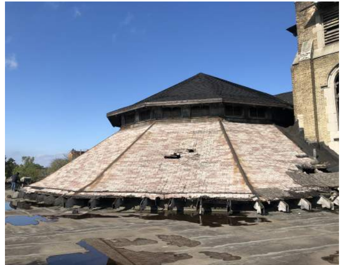
FIGURE A2.1 OVERVIEW OF THE TWO TIERED HEPTAGON ROOF; ROOF DECAY AND WATER INFILTRATION, WORN AND MISSING ASPHALT TILES, WEATHERED AND ROTTED DECORATIVE EAVE OUTRIGGERS/RAFTER TAILS.
