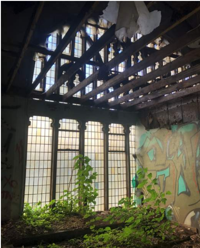
FIGURE INT 1.8 FAILED FINISHES AND VEGETATION IN SANCTUARY MEZZANINE OPEN TO THE ELEMENTS ABOVE
