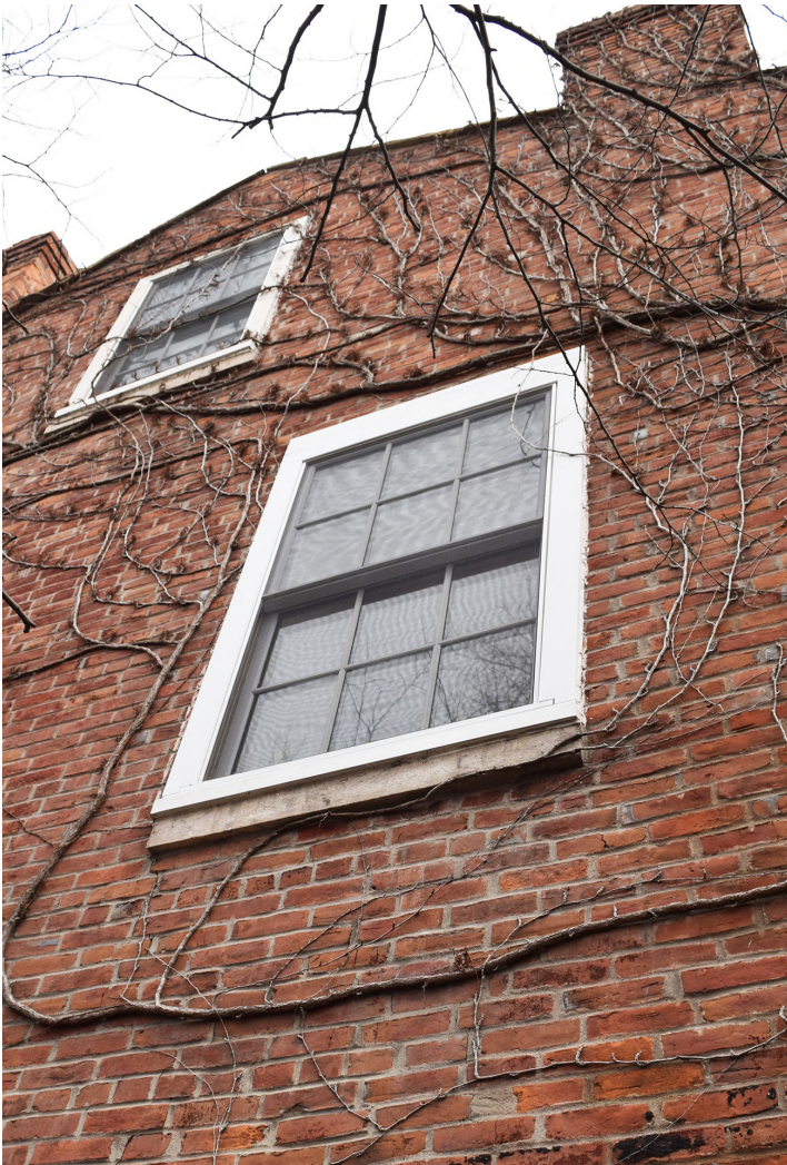
3. WINDOW TO BE REMOVED AND OPENING TO BE ENLARGED DOWN TO SECOND LEVEL FLOOR LINE. DOOR AND FRAME REMOVED FROM KITCHEN BELOW TO BE INSTALLED IN OPENING.
