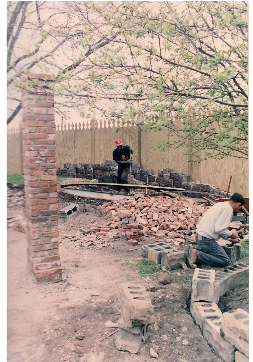
PERGOLA AND CMU PLANTER BEING CONSTRUCTED OF MATERIALS FROM DEMOLISHED GARAGE AND SIDE PORCH DURING 1992 RENOVATION
