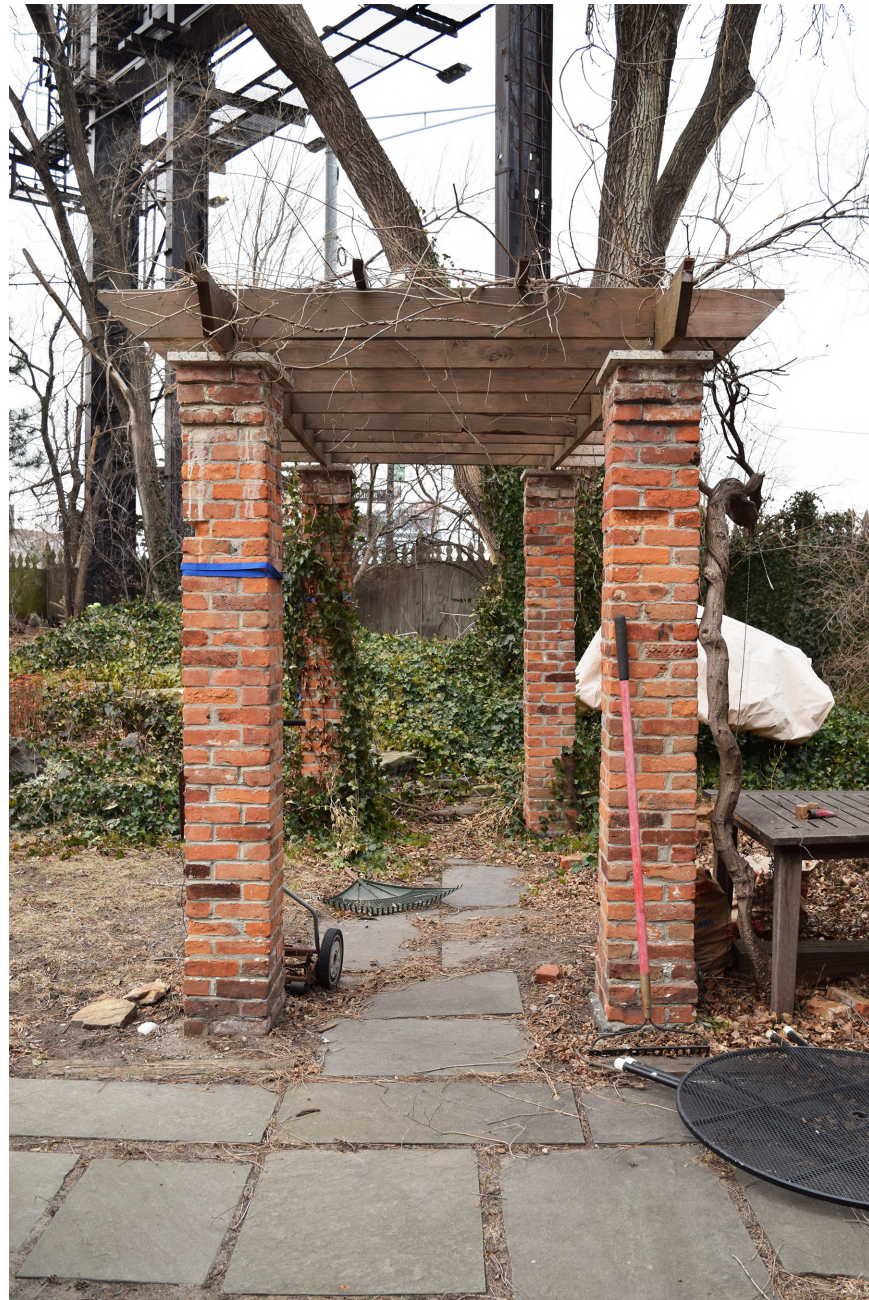
BRICK PERGOLA AT SIDE YARD CONSTRUCTED DURING 1992 RENOVATION TO BE REMOVED
