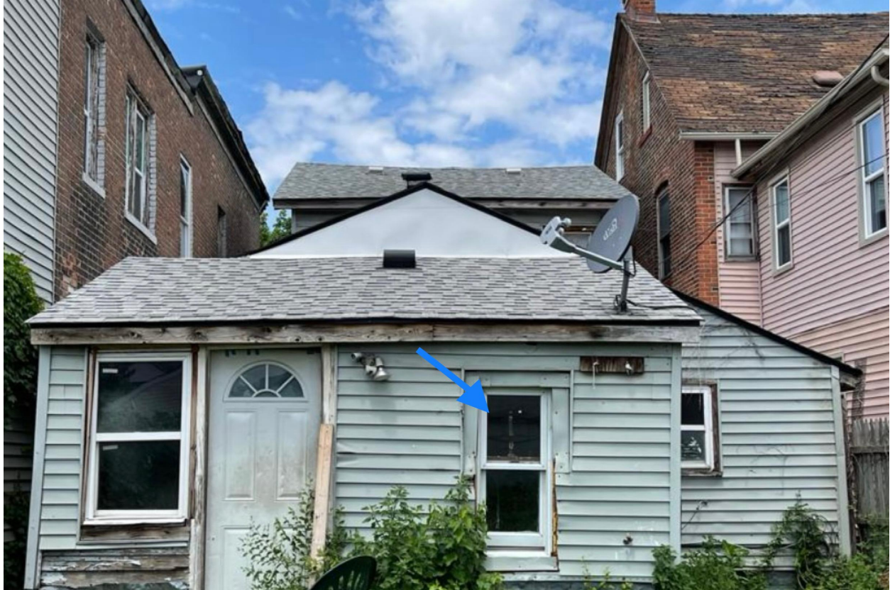
DETERIORATION TO EXISTING WINDOWS
