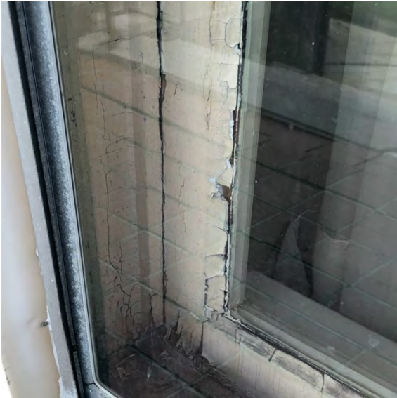
Deteriorated Window Sash
