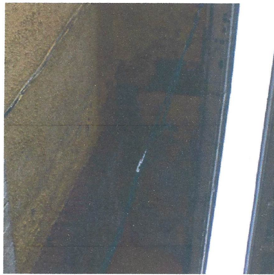
Roof Soffit Damage
