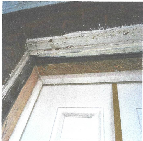
Deteriorated Exterior Door Jamb, Lintel & Casing
