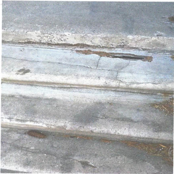
Porch Step Damage (Side A)
