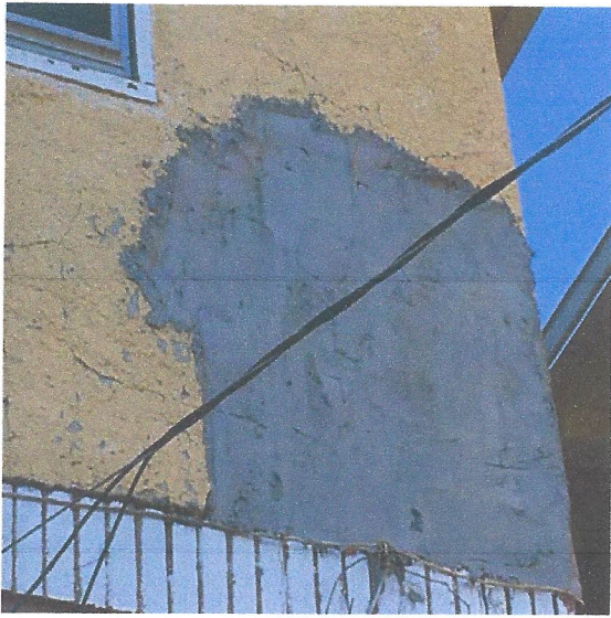
Deteriorated Exterior Walls
