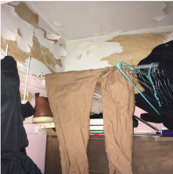
Bedroom 2 Closet Moisture Damage
