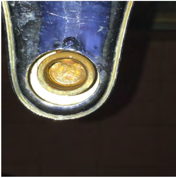
Bathroom Faucet With No Aerator
