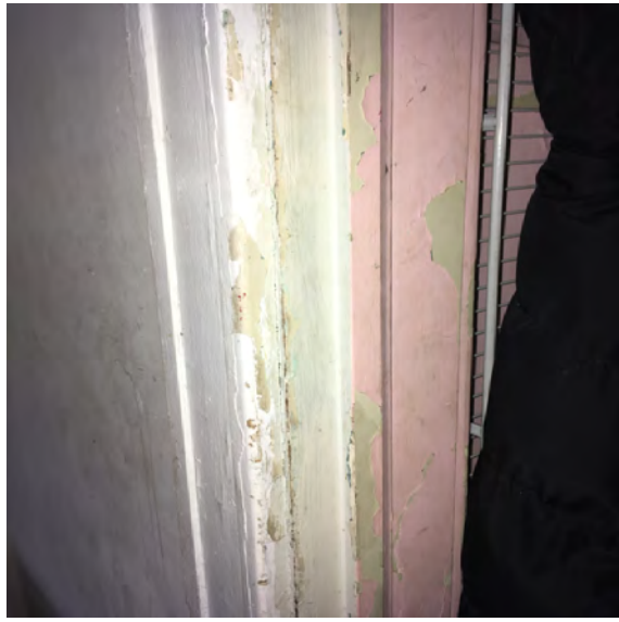
Deteriorated Interior Door Components
