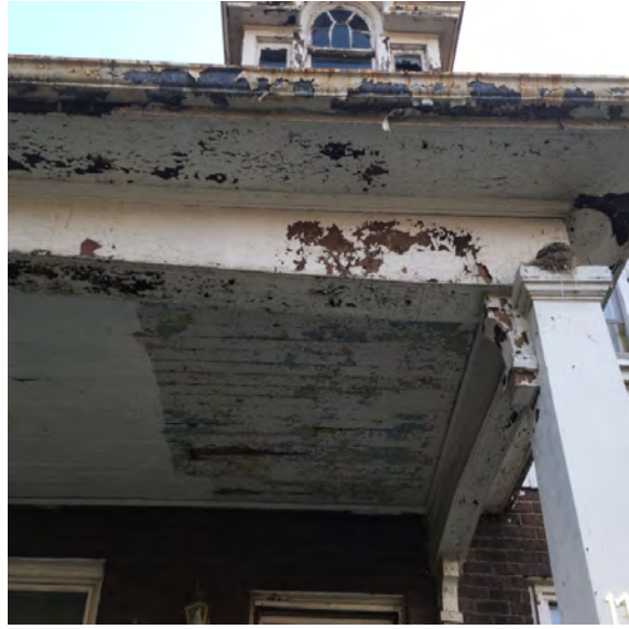
Deteriorated Porch Ceiling, Ceiling Beam & Columns
