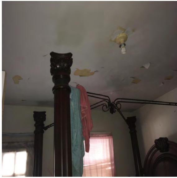
Bedroom 1 Ceiling Moisture Damage
