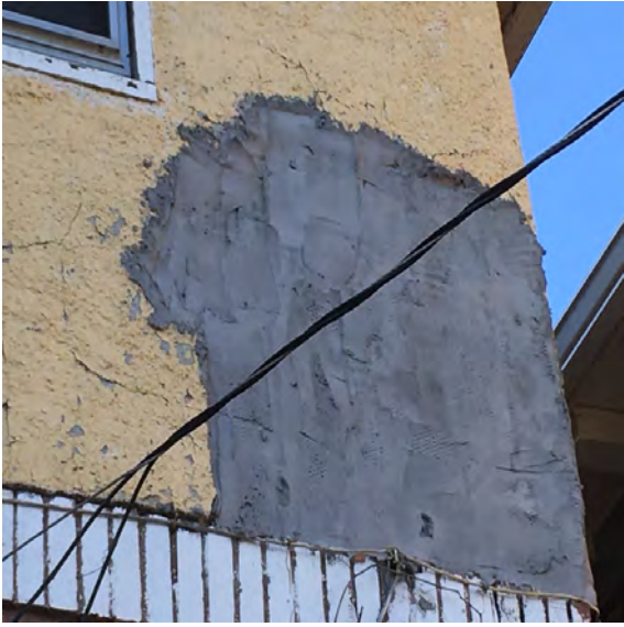
Deteriorated Exterior Walls
