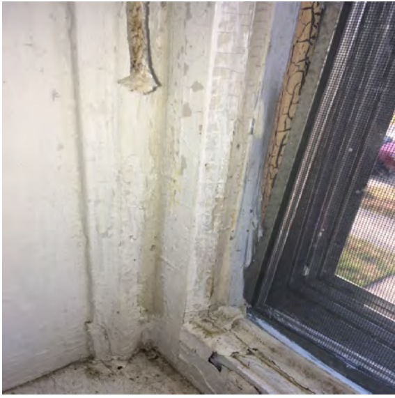
Some Windows are Painted Shut Pic 1
