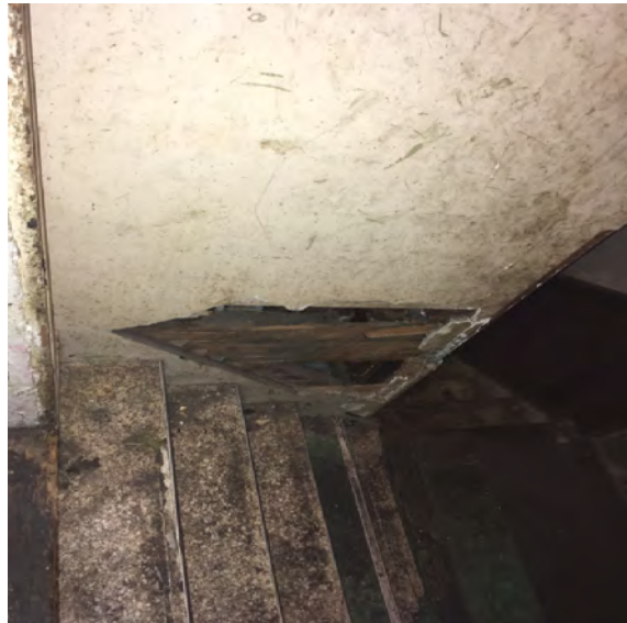
Stairwell 3 Wall Damage
