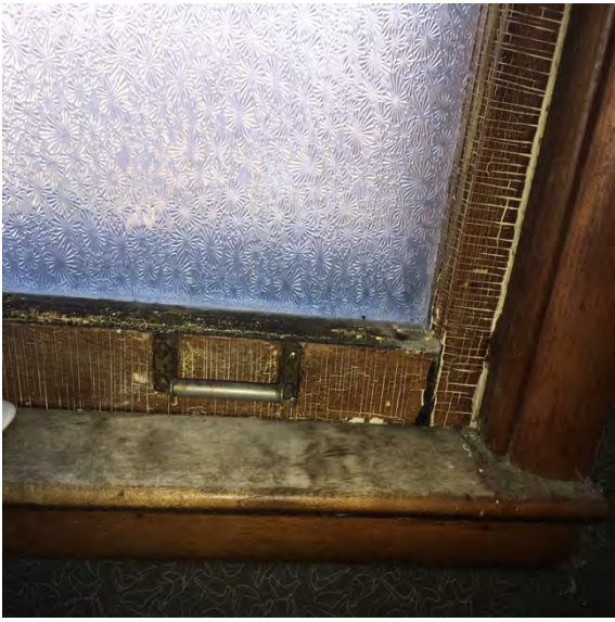
Bathroom Deteriorated Varnish Window Sash
