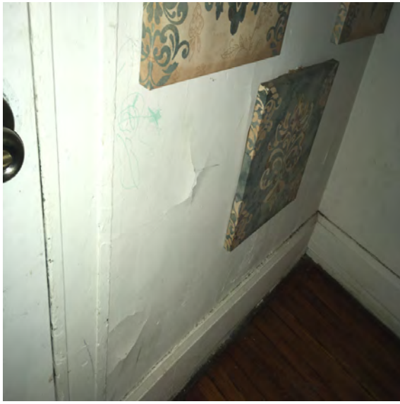
Stairwell 1 Wall Damage
