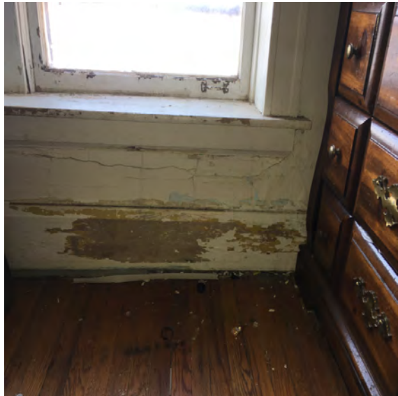
Bedroom 2 Moisture Damaged Wall & Baseboard
