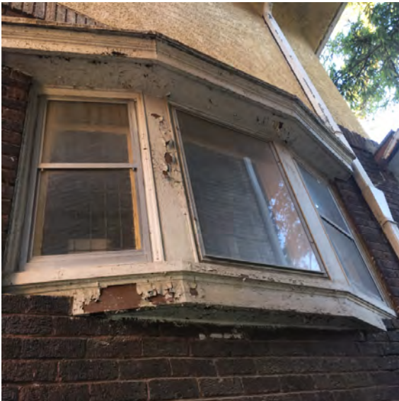
Deteriorated Exterior Window Components Pic 2
