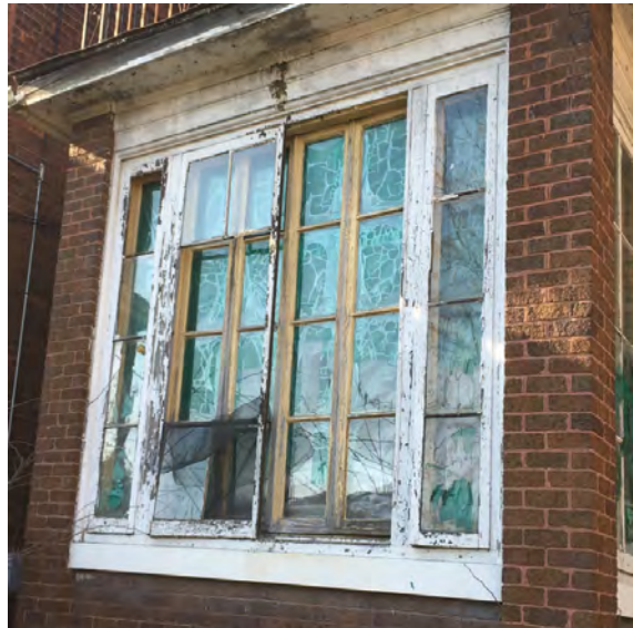
Deteriorated Exterior Window Components Pic 3
