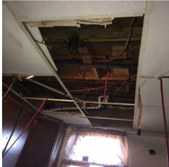
Kitchen Ceiling Pic 1
