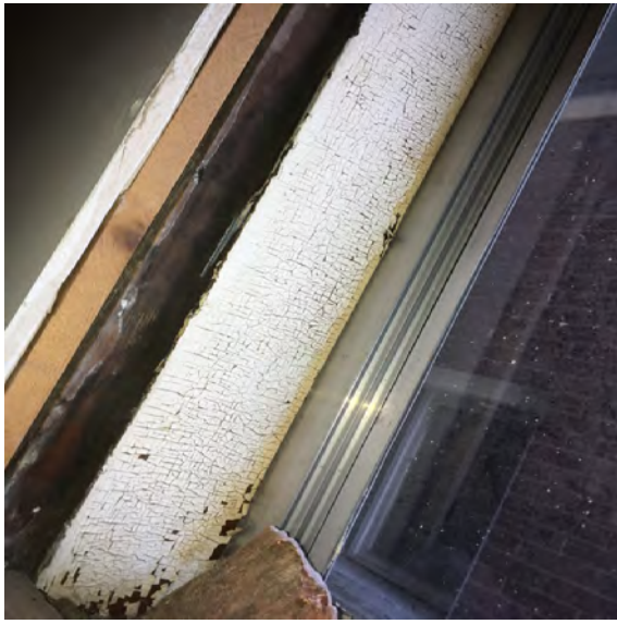
Deteriorated Exterior Fixed Window Jamb
