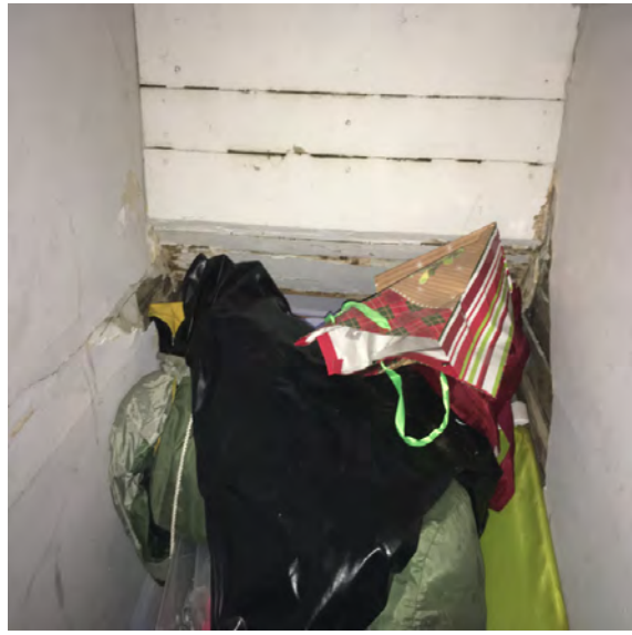
Stairwell 1 Closet Damage
