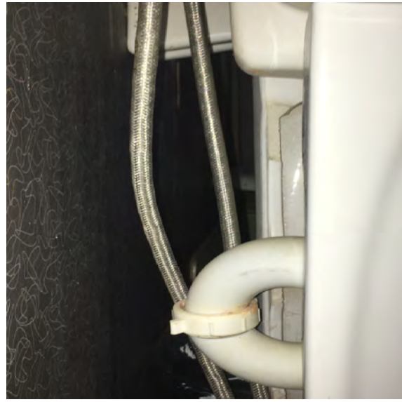
Bathroom Sink Pipes
