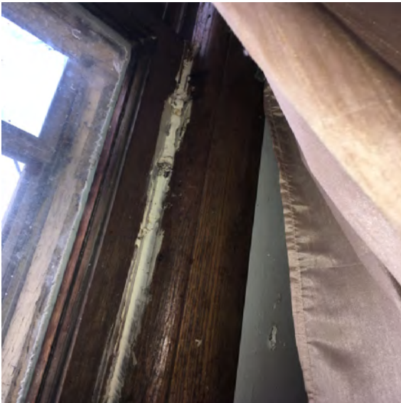
Window Calked Shut (Wall C)
