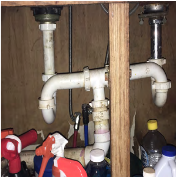
Kitchen Sink Pipes
