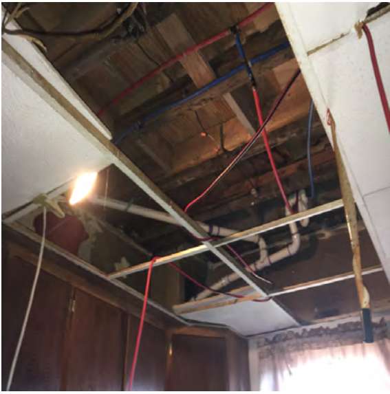
Kitchen Ceiling Pic 2
