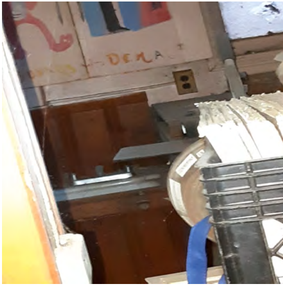
Bar Sink in Basement Not in Use
