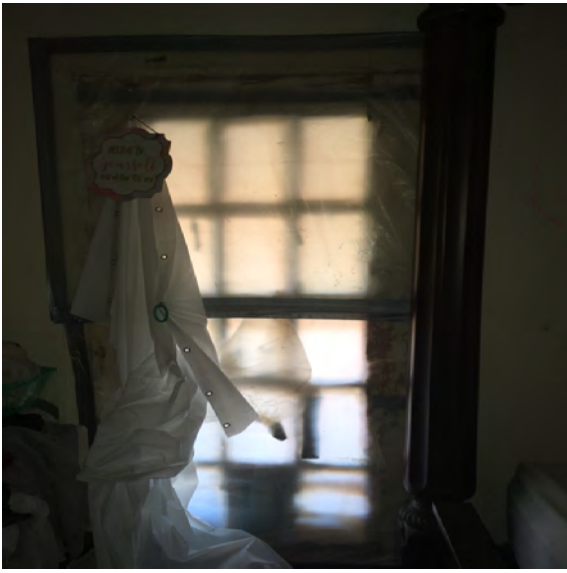
Bedroom 1 Exterior Door Screwed Shut
