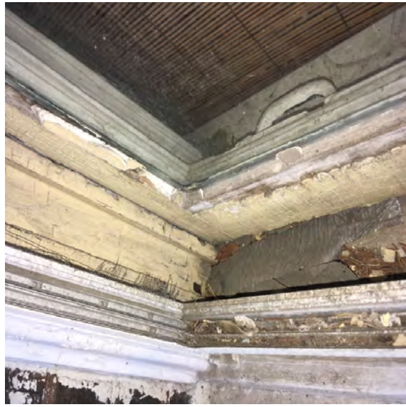
Deteriorated Exterior Window Components Pic 1
