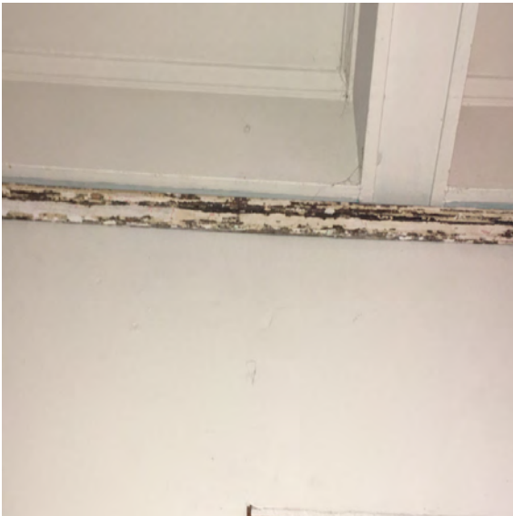
Living Room Deteriorated Crown Molding
