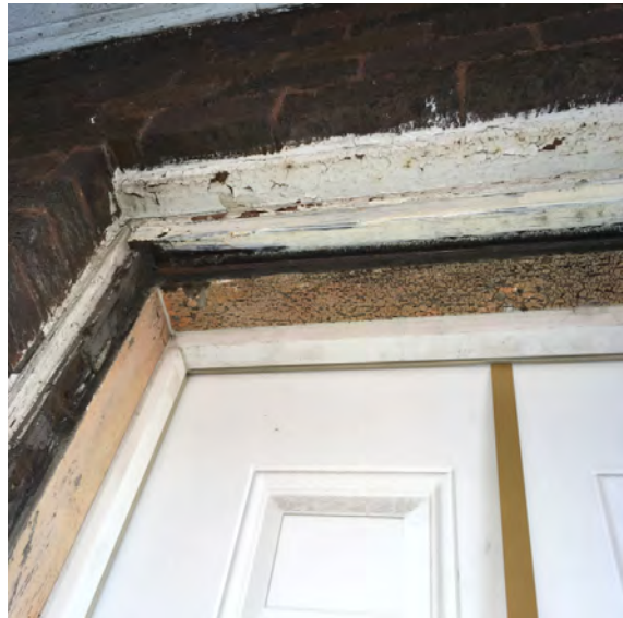
Deteriorated Exterior Door Jamb, Lintel & Casing
