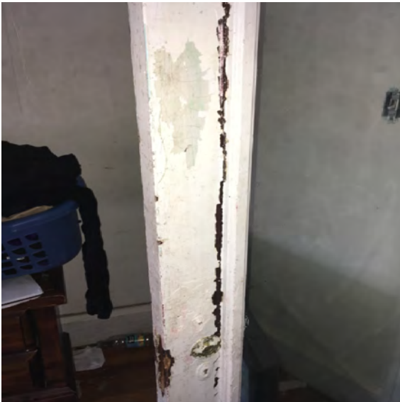
Deteriorated Interior Door Stile
