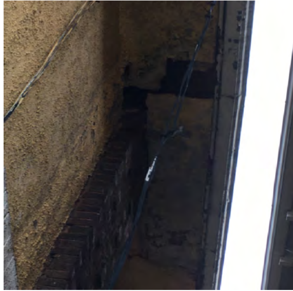
Roof Soffit Damage
