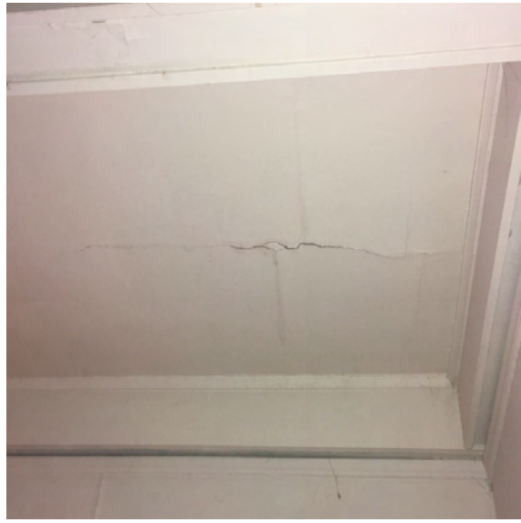
Living Room Ceiling Damage
