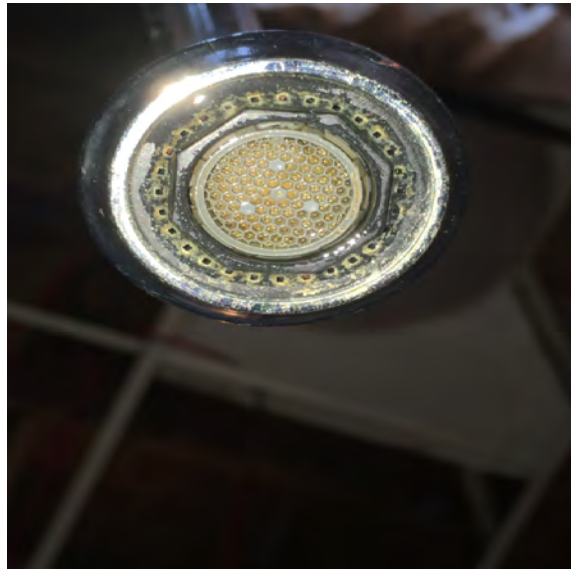
Kitchen Sink Faucet with Aerator
