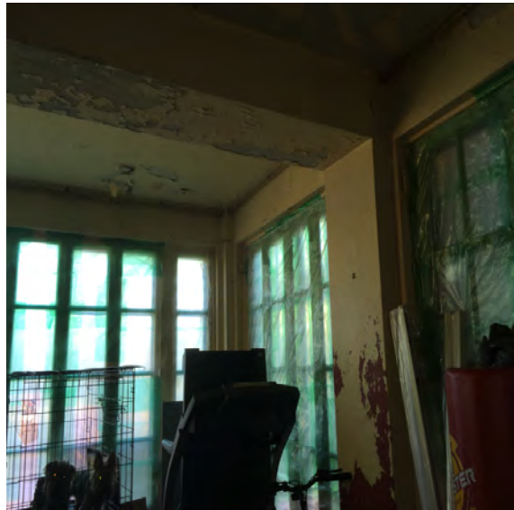
Enclosed Porch Deteriorated Ceiling & Walls
