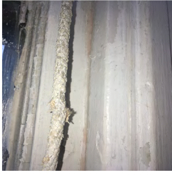
Some Windows are Painted Shut Pic 2
