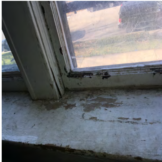
Deteriorated Interior Window Components
