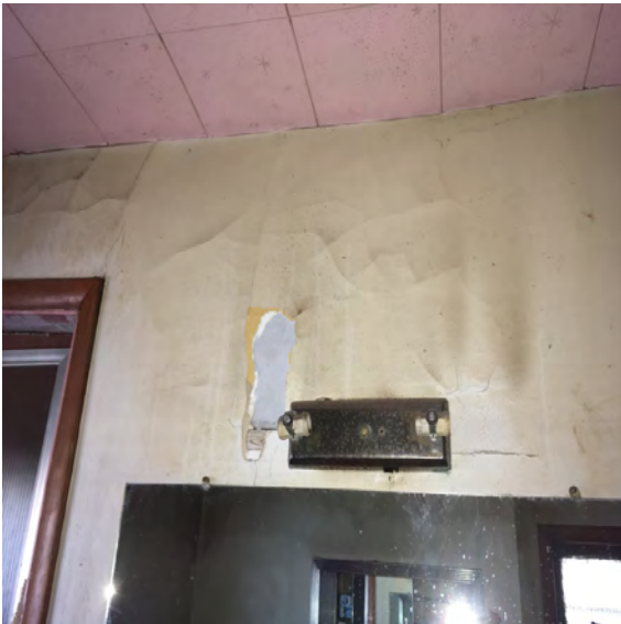
Bathroom Deteriorated Walls
