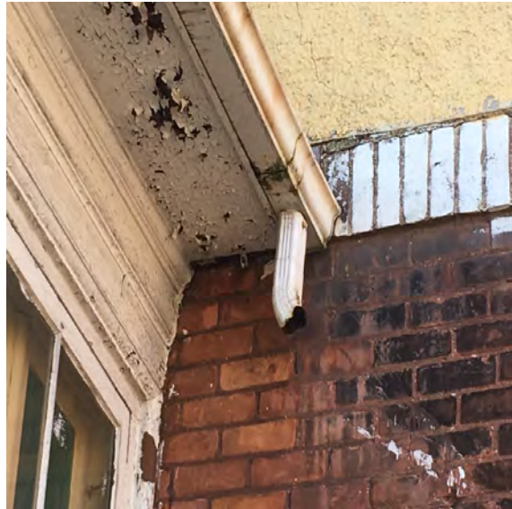
Damaged Gutter Downspout Pic 2
