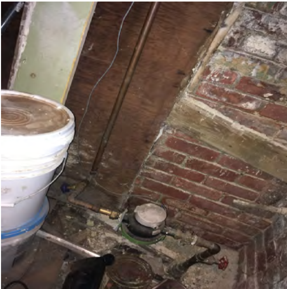
Water Meter with A Cooper Line
