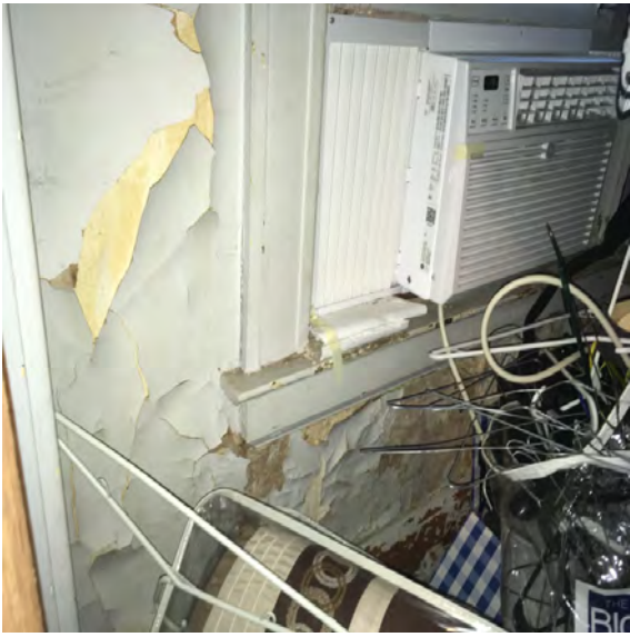
Bedroom 3 Closet 1 Moisture Damage
