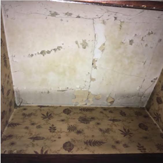
Foyer Ceiling Moisture Damage
