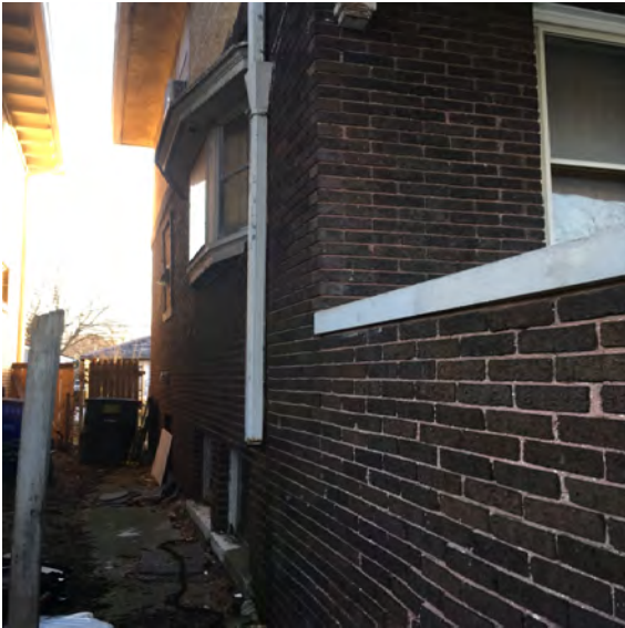
Damaged Gutter Downspout Pic 1
