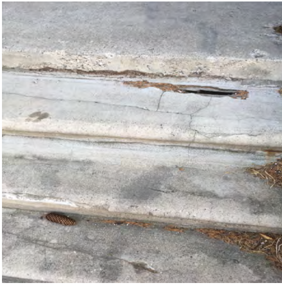
Porch Step Damage (Side A)
