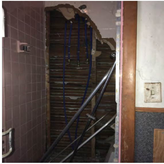
Bathroom Shower Damage
