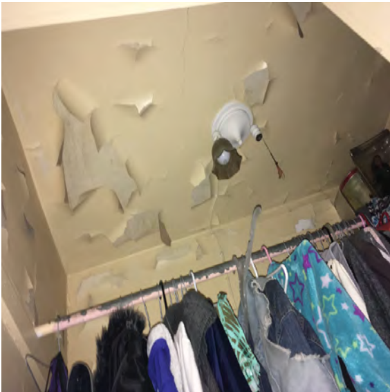
Bedroom 1 Closet Moisture Damage
