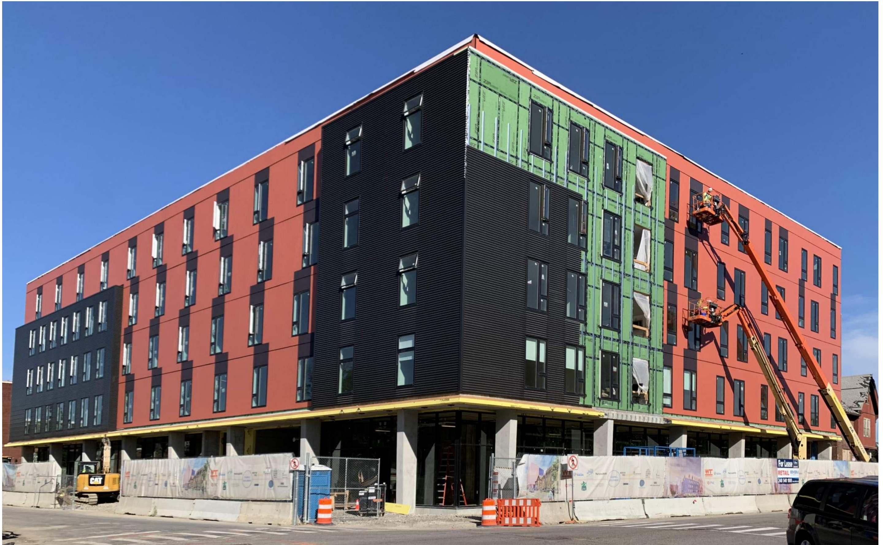
Photograph Showing Facade With No Window Inset. (Photo taken on 6/16/2021)
