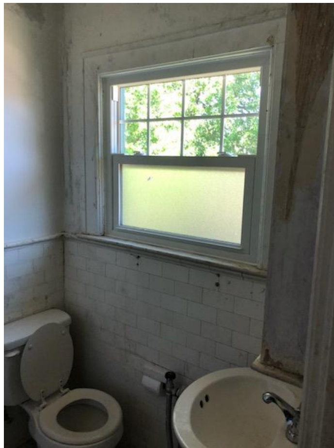
UPPER BATHROOM (BACK BEDROOM)
