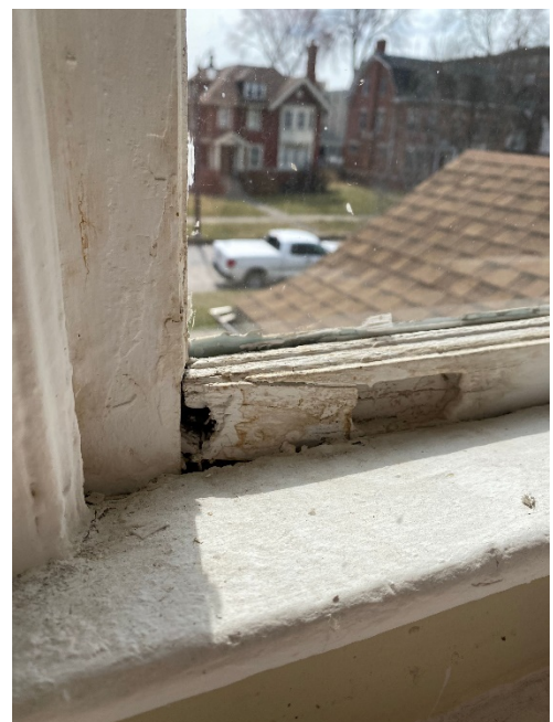
Rot at window sashes
