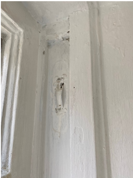
Operating hardware missing or inoperable
