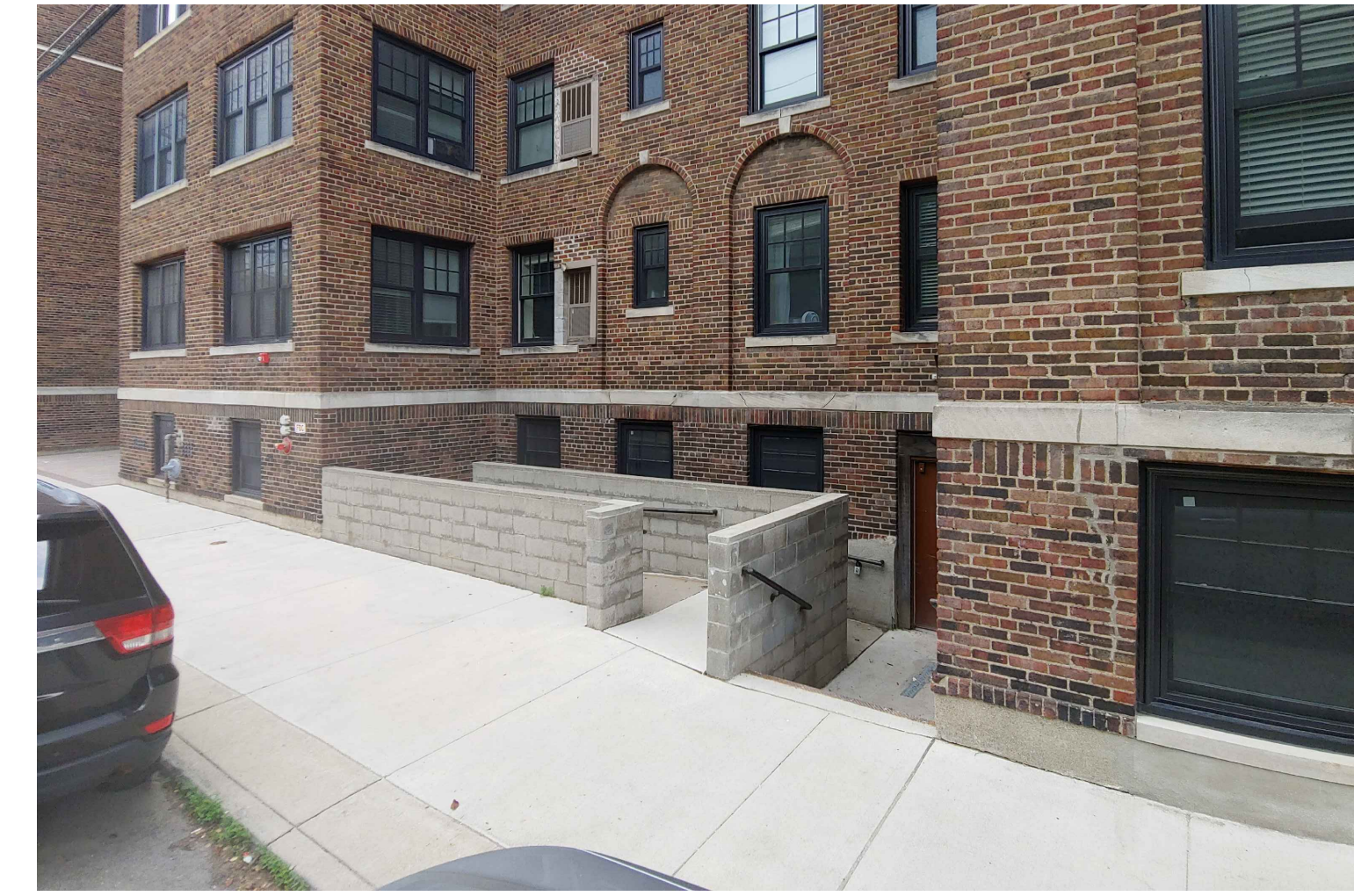
Proposed canopy location over existing ramp and stair off of Beaubien Street
