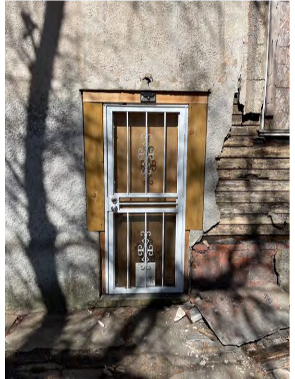
EXISTING GRADE DOOR TO BASEMENT W/ SECURITY DOOR PROPOSED FOR REPLACEMENT (EAST FACADE)
