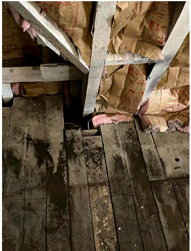
GAPS IN STRUCTURE CAUSED BY STUCCO WEIGHT
