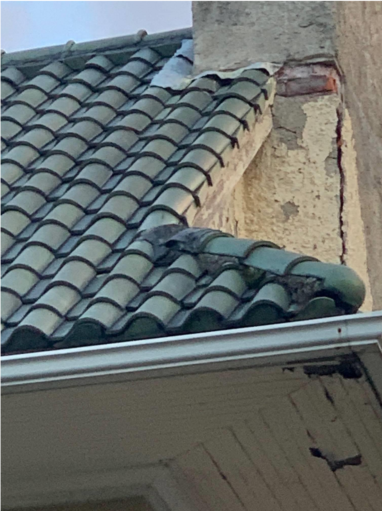
Missing Tile Detail 3 9-10
