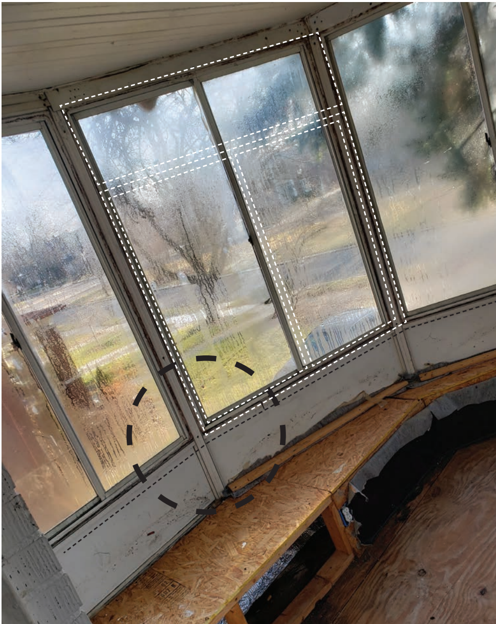
Fig. 9| Above: 2020 Interior photo shows existing Sunroom. To the left you can see the brick exterior wall that is now enclosed w/ 180 degree window view from the bow of the "boat." The dashed white lines highlight the proposed new window proportions.
