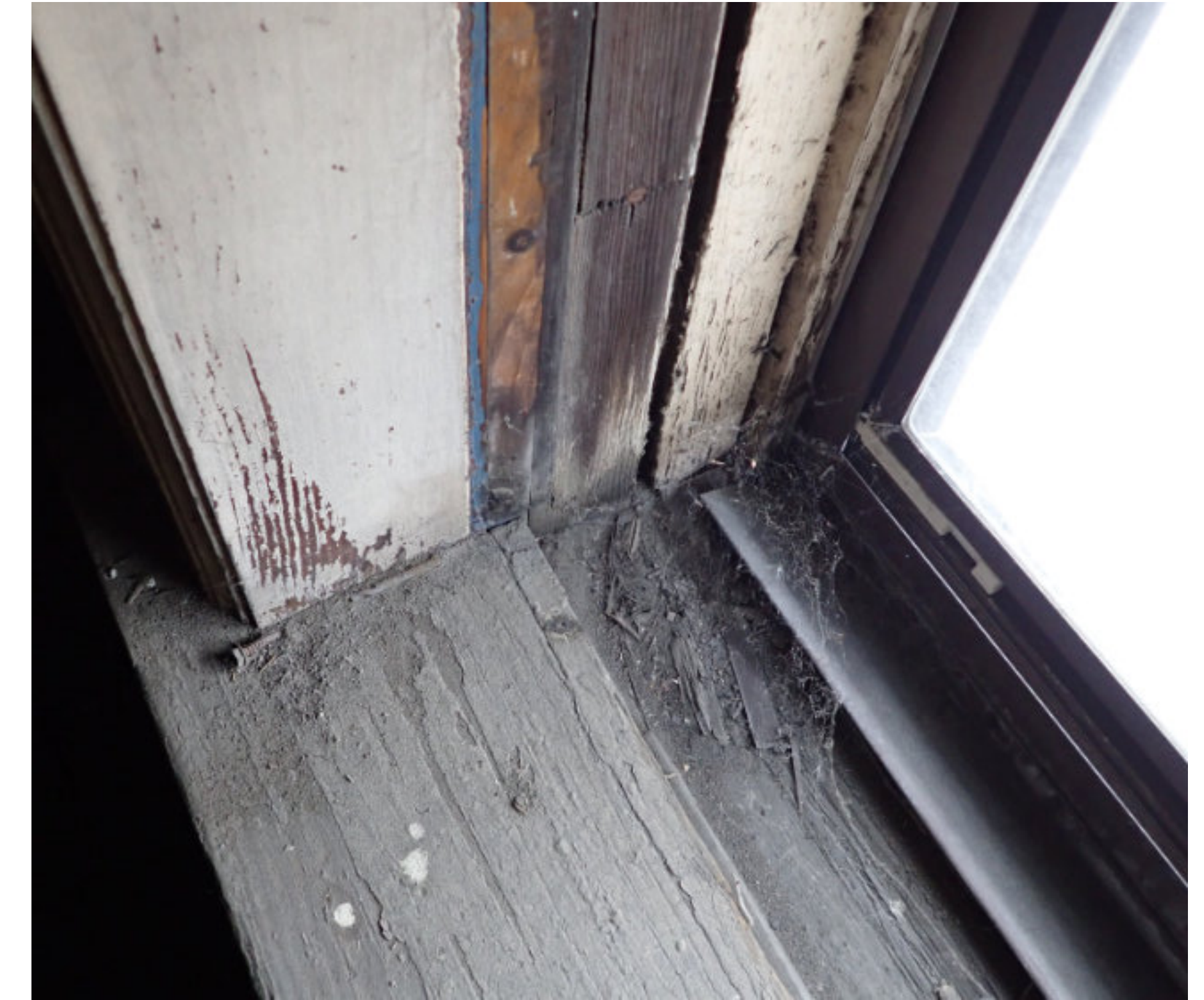
UNIT 204: DETERIORATED STOOP AND CASING
