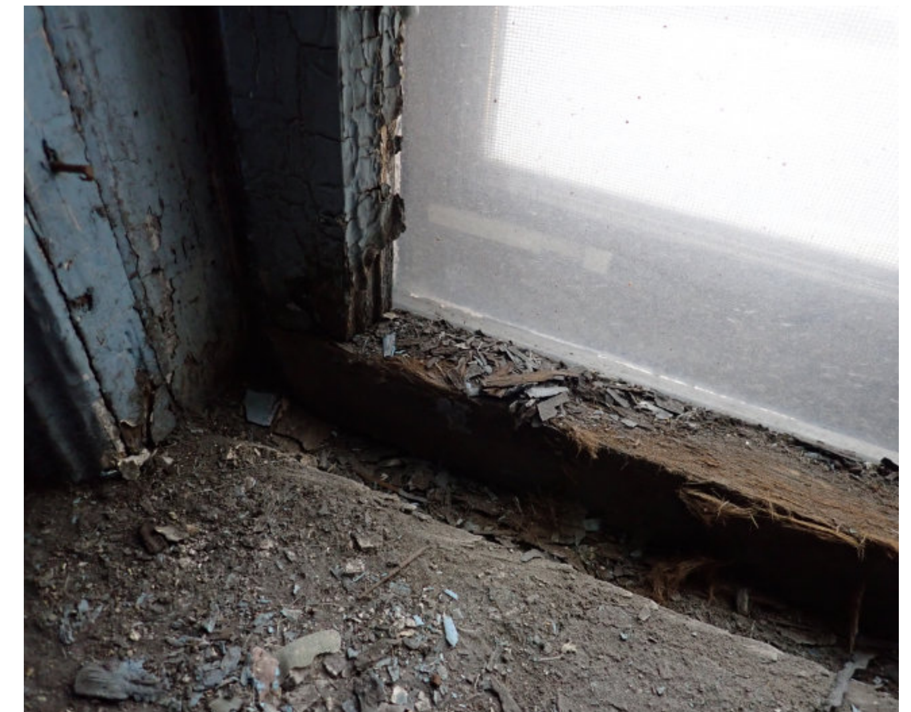
UNIT 204: DETERIORATED LOWER RAIL
