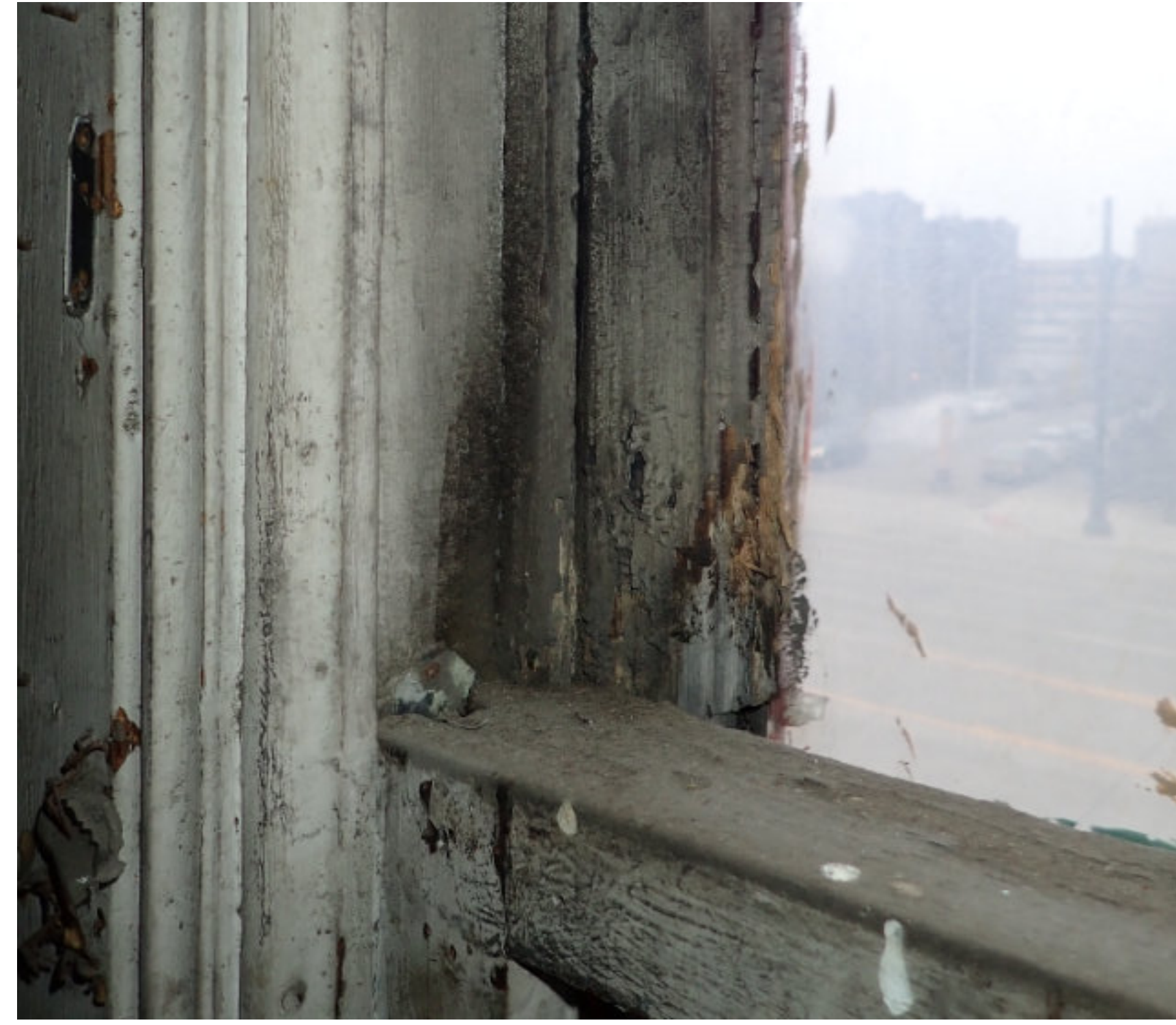
UNIT 208: DETERIORATED STILE
