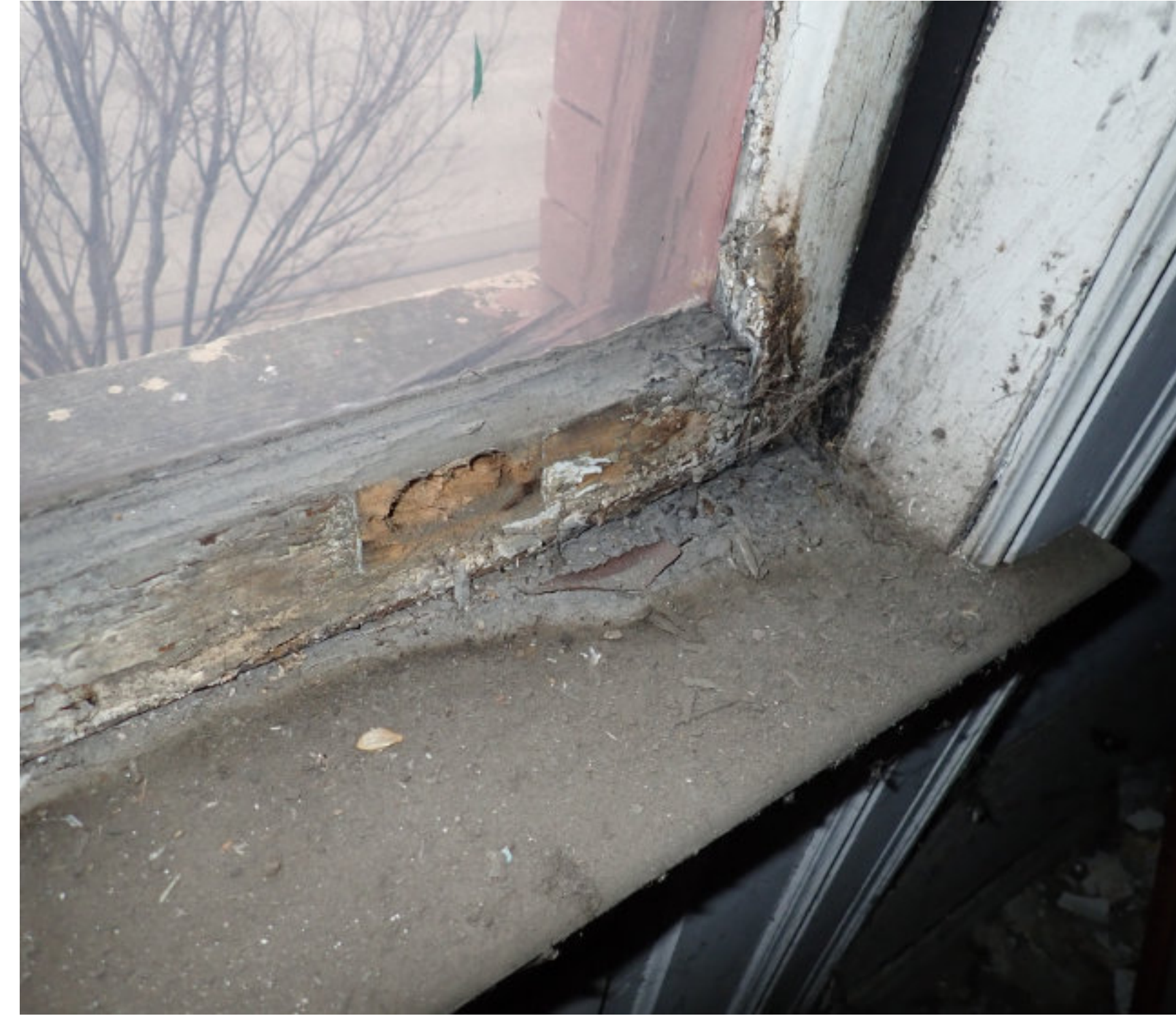
UNIT 206: DETERIORATED LOWER RAIL
