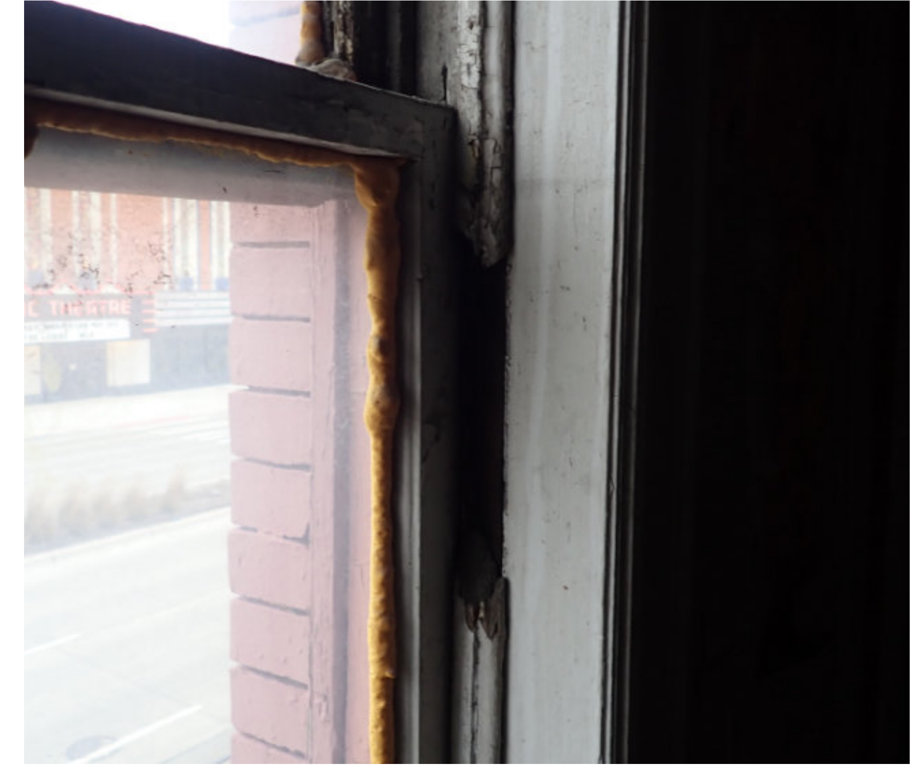
UNIT 207: BROKEN AND MISSING STOP
