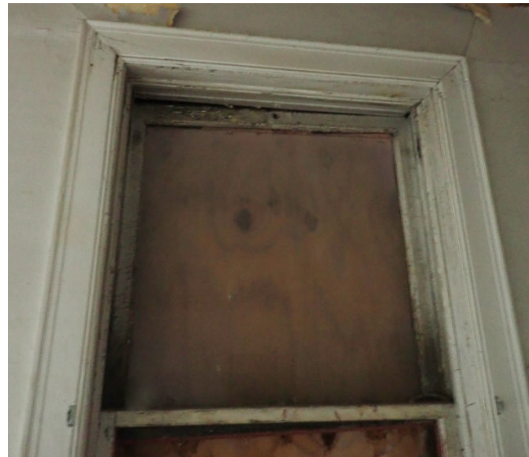
UNIT 206: BROKEN AND OUT OF ALIGNMENT RAILS
