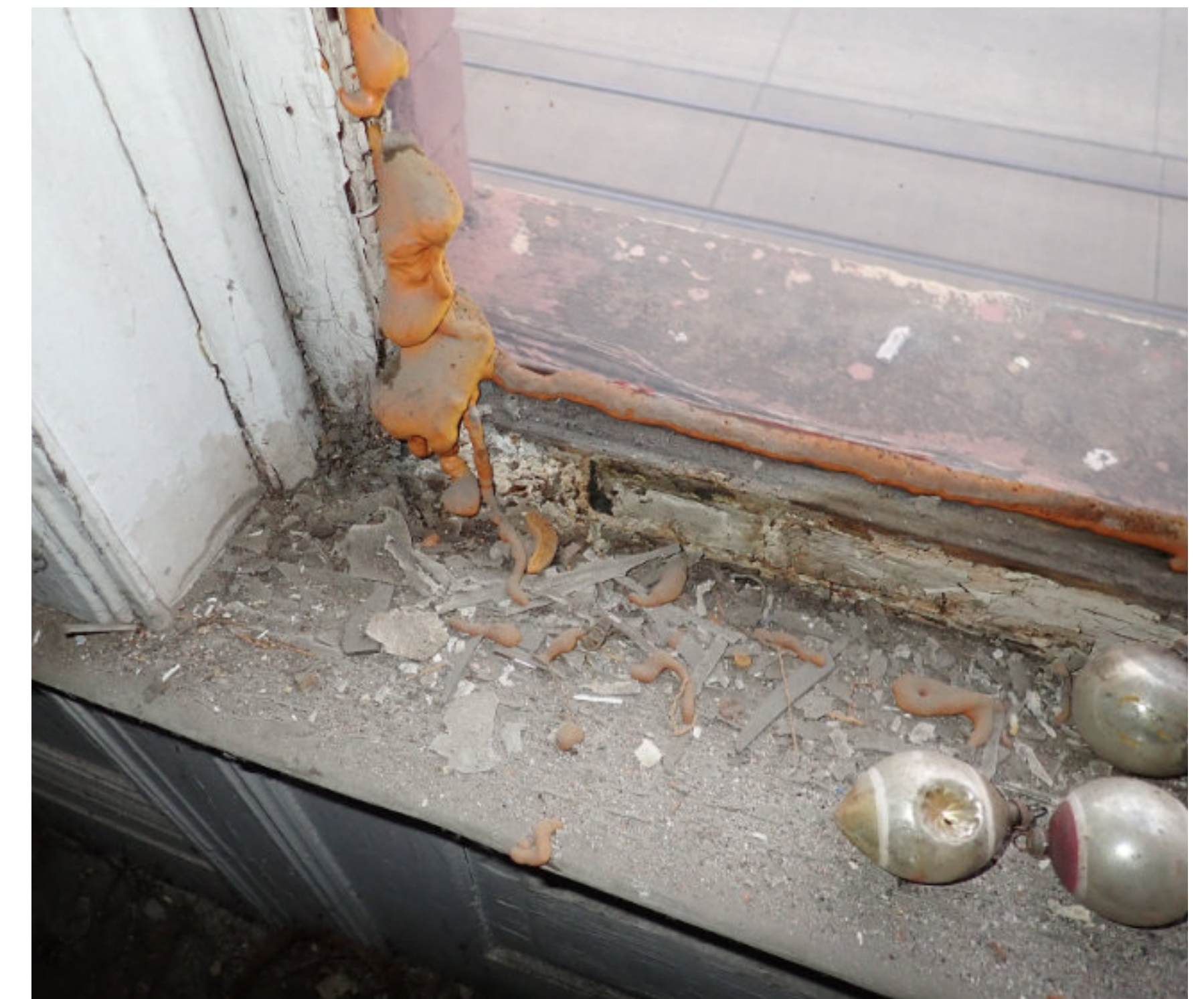
UNIT 207: INAPPROPRIATE MATERIAL
