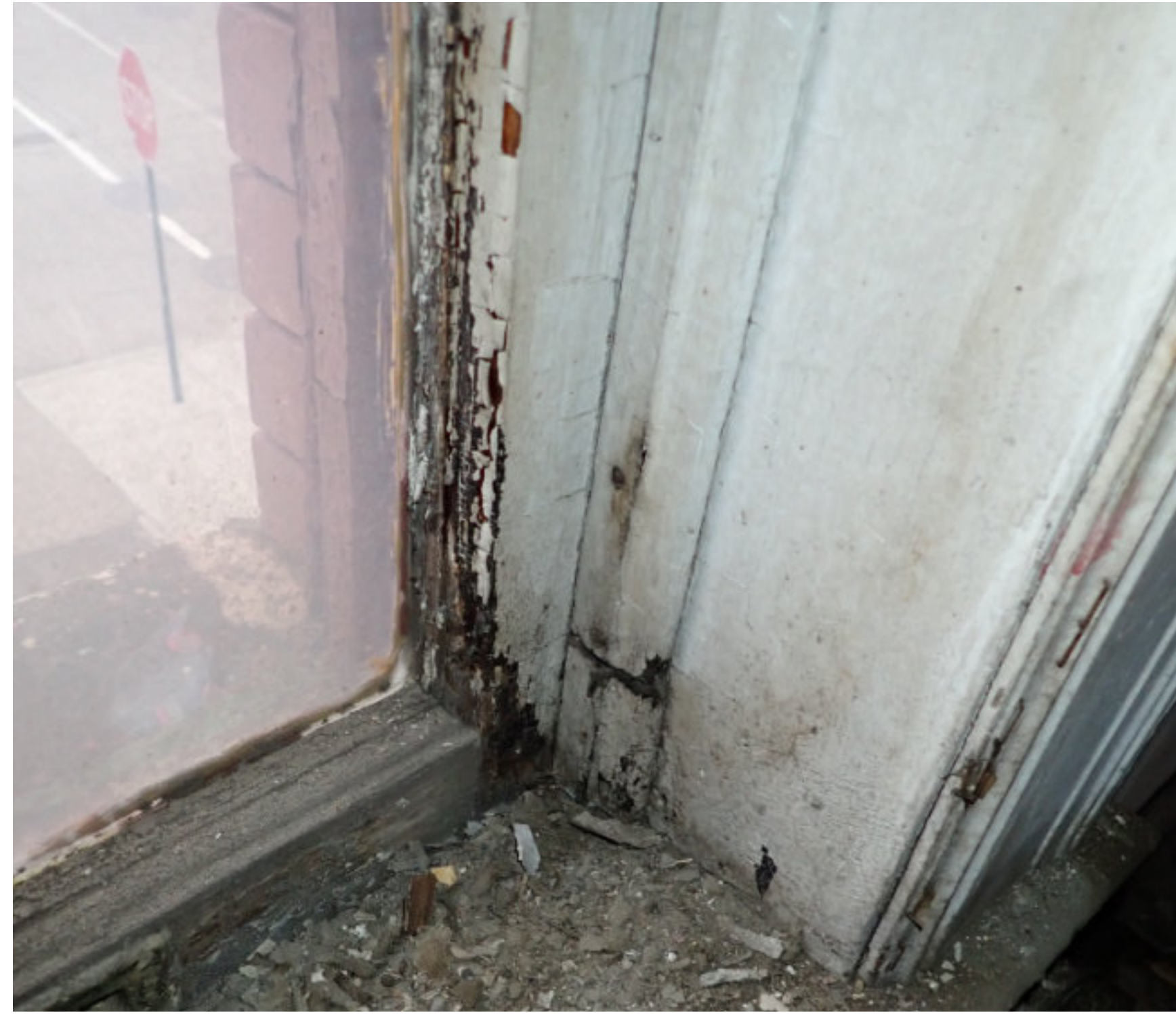
UNIT 208: DETERIORATED STILE
