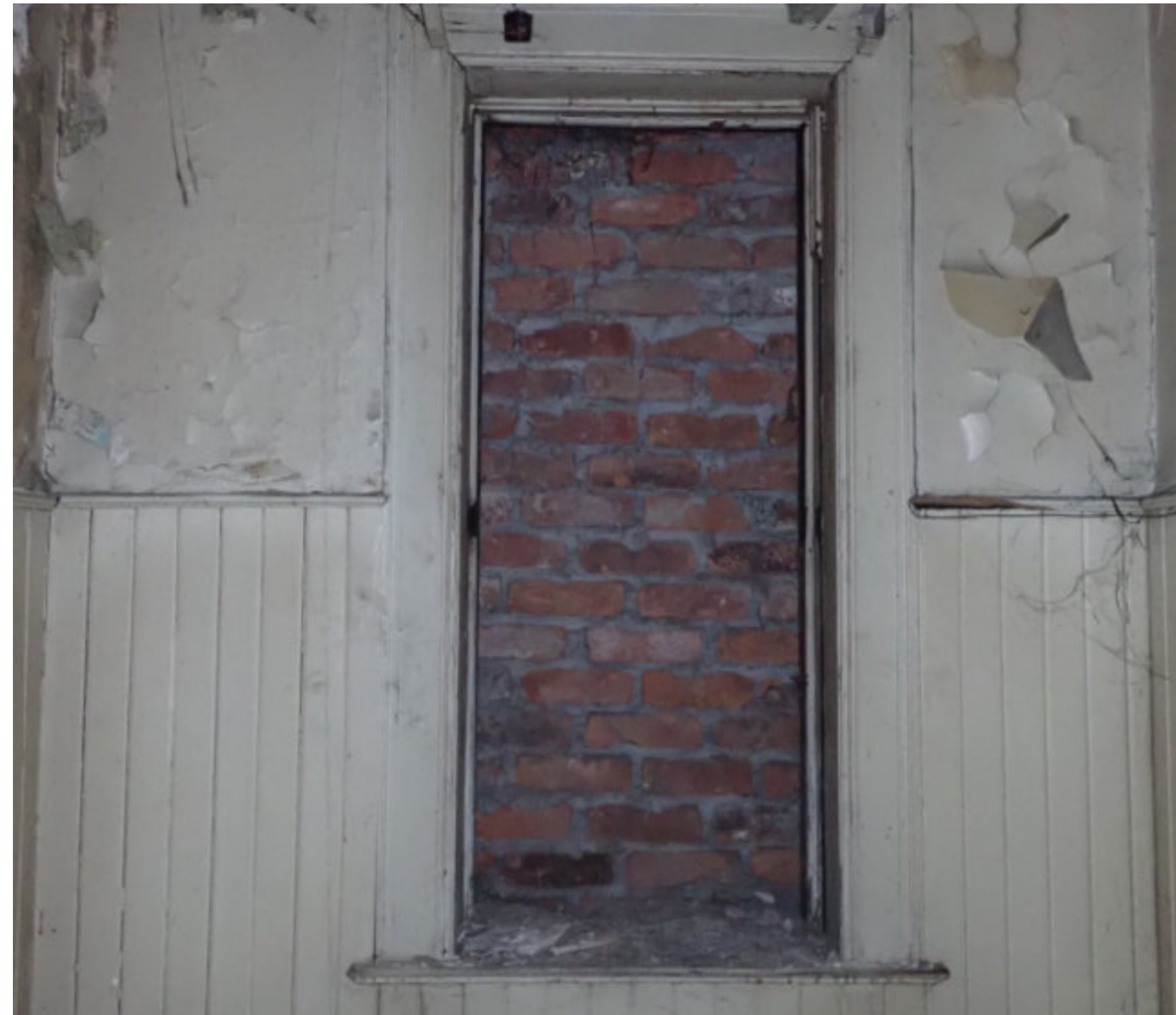
UNIT 206: MISSING WINDOW WITH BRICK INFILL
