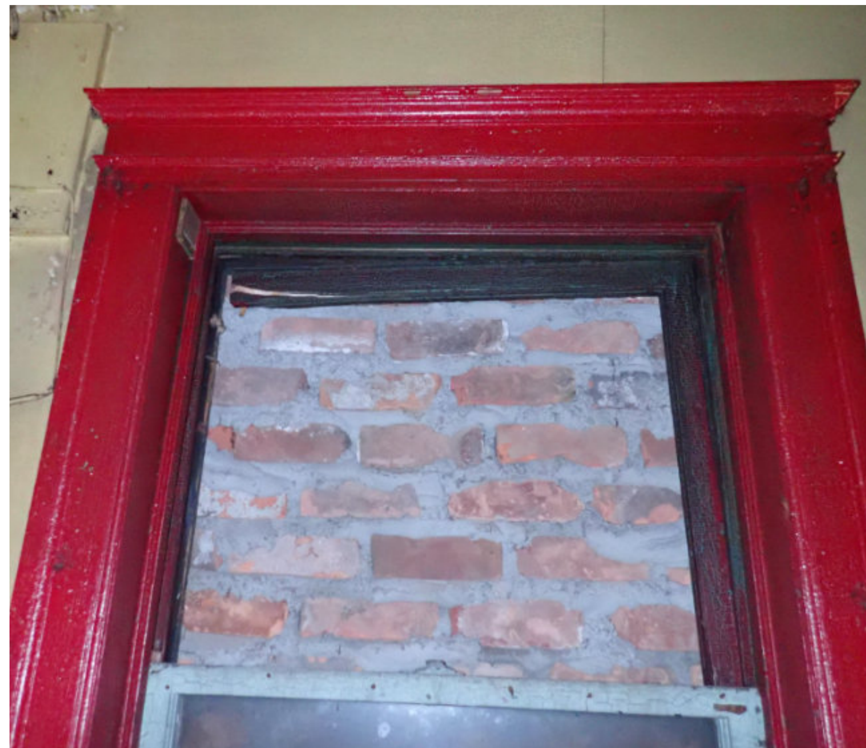
UNIT 202: BROKEN TOP RAIL
