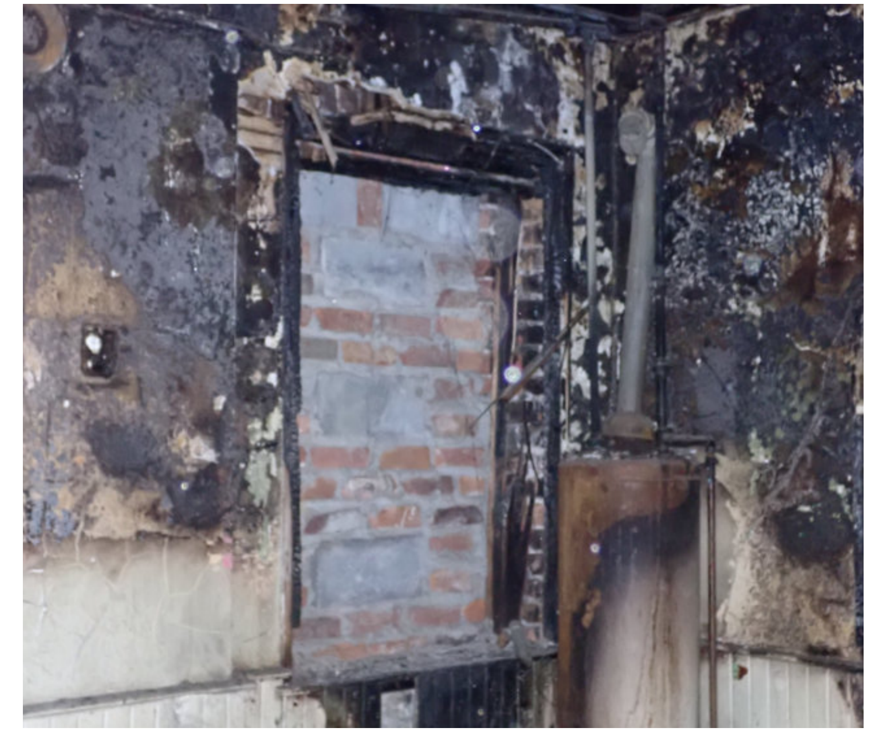
UNIT 208: FIRE DAMAGE
