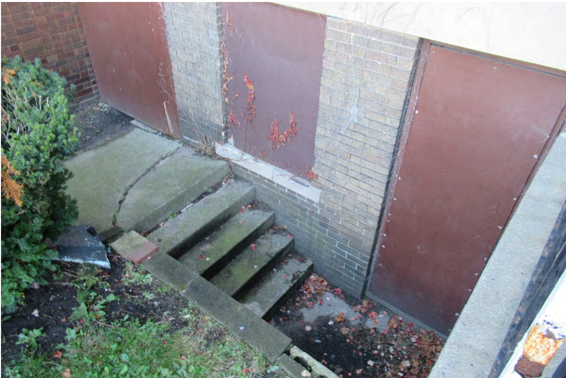
Figure #13: Exterior, Eastern side of North façade, Exterior access to basement, Looking Down. 10/28/20.
