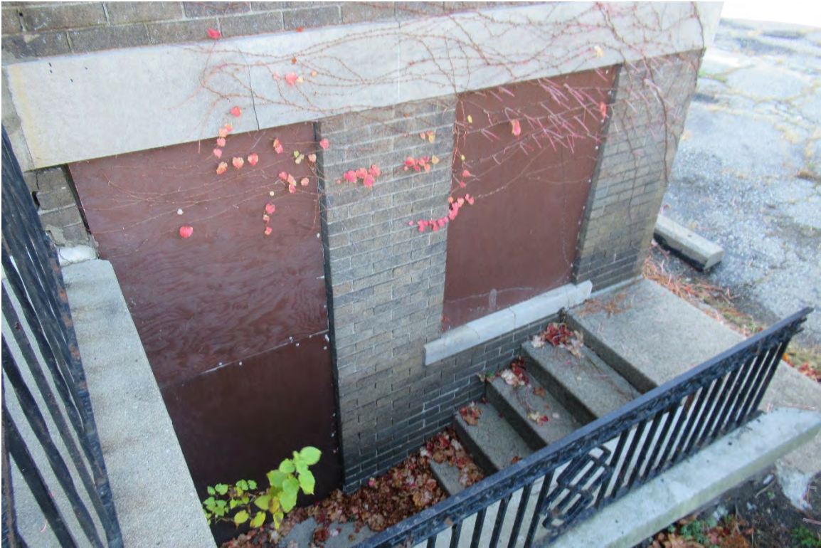
Figure #12: Exterior, Western side of North façade, Exterior access to basement, Looking Down. 10/28/20.
