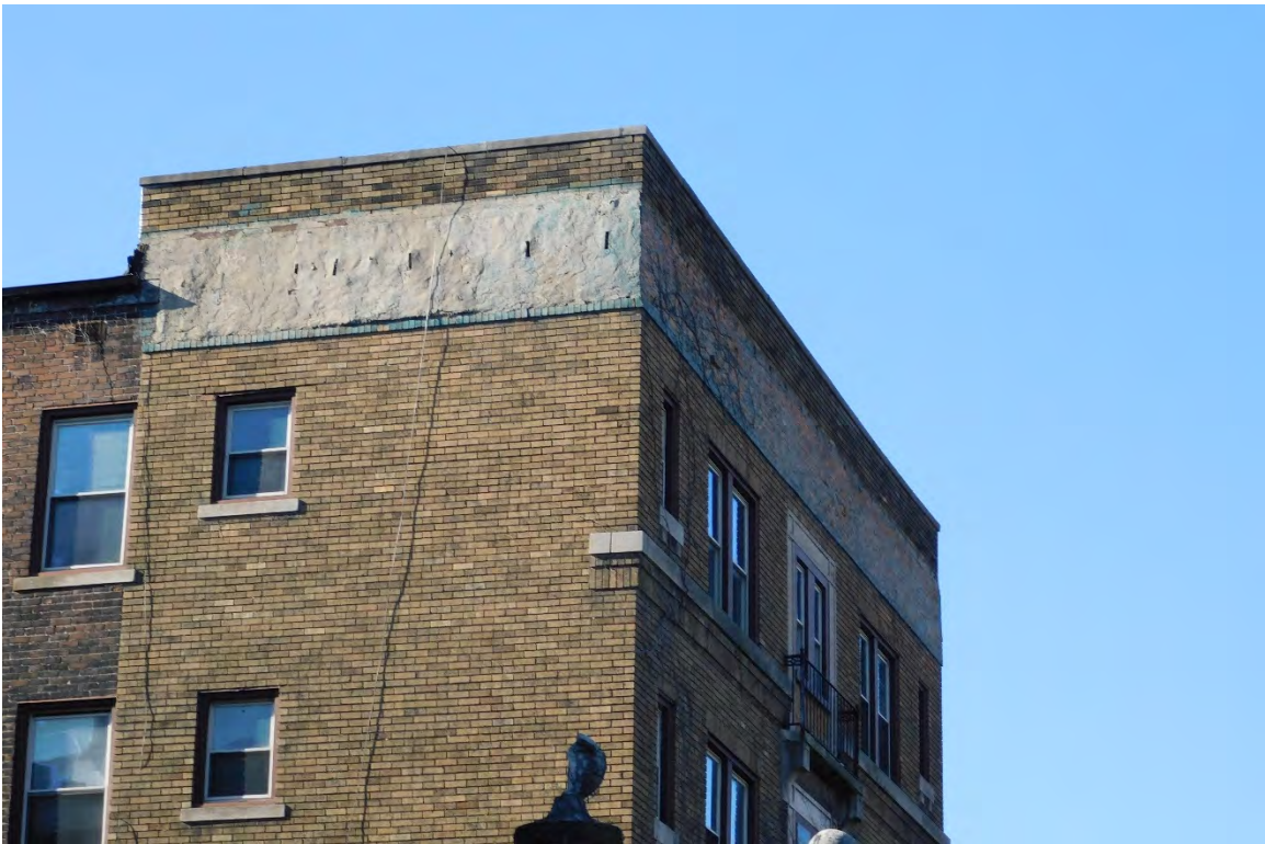
Figure #17: Exterior, North and East facades, missing cornice detail, Looking Up. 10/28/20.
