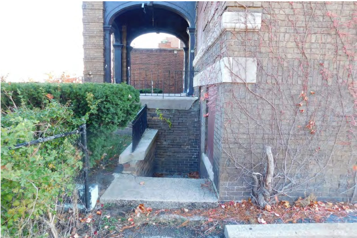
Figure #11: Exterior, Western side of North façade, Exterior access to basement, Looking East. 10/28/20.
