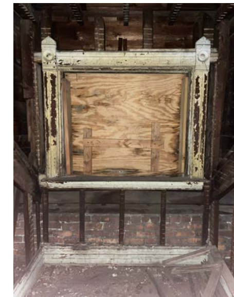
WINDOW 3B - WEST (INTERIOR) MISSING ASSUMED FRENCH CASEMENT
